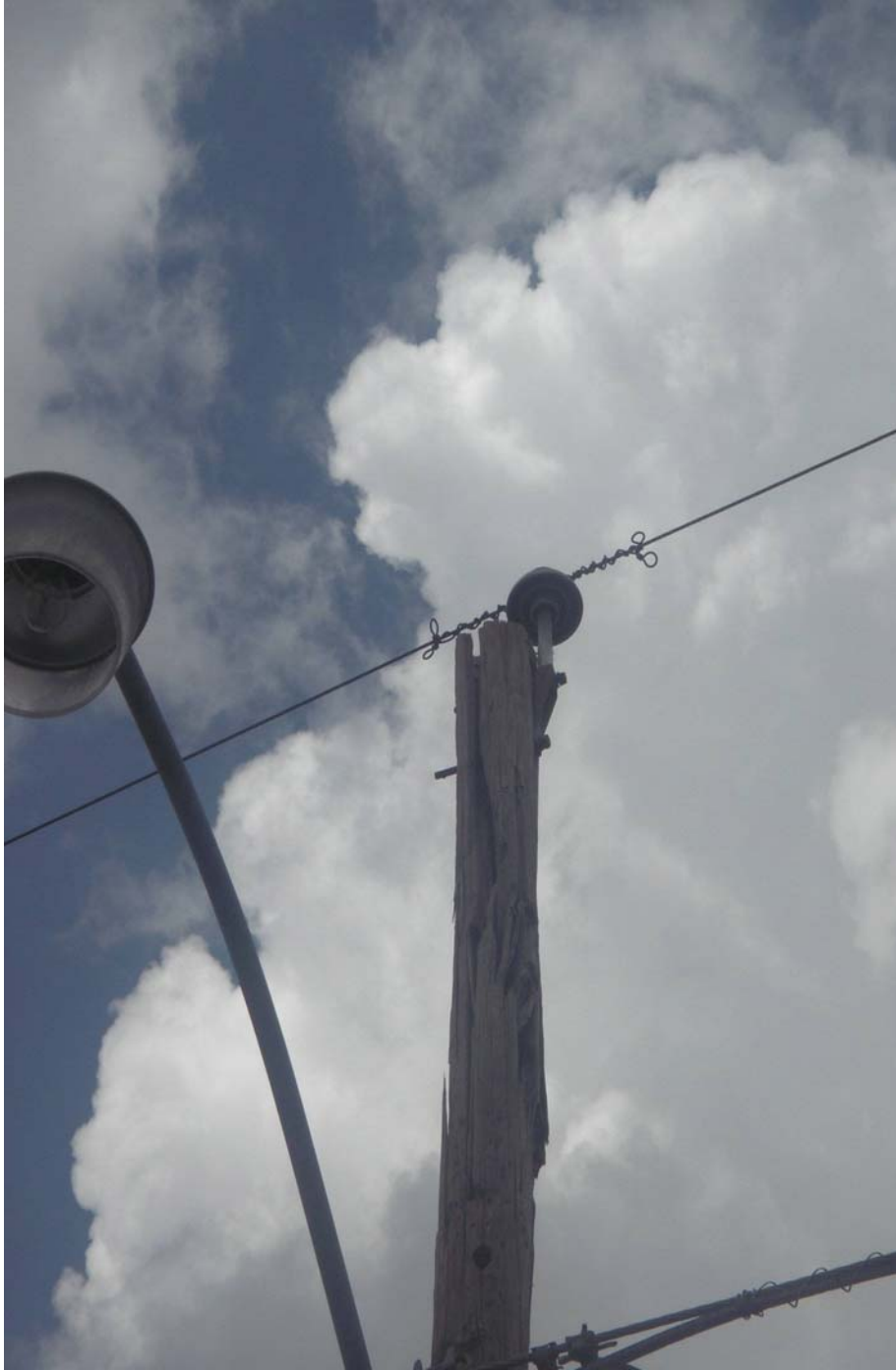
FPL Top of pole severely deteriorated. Pole supports single phase line. Pole # 8-6882-5450 at 8411 NW 24th Ct. in Fort Lauderdale.
