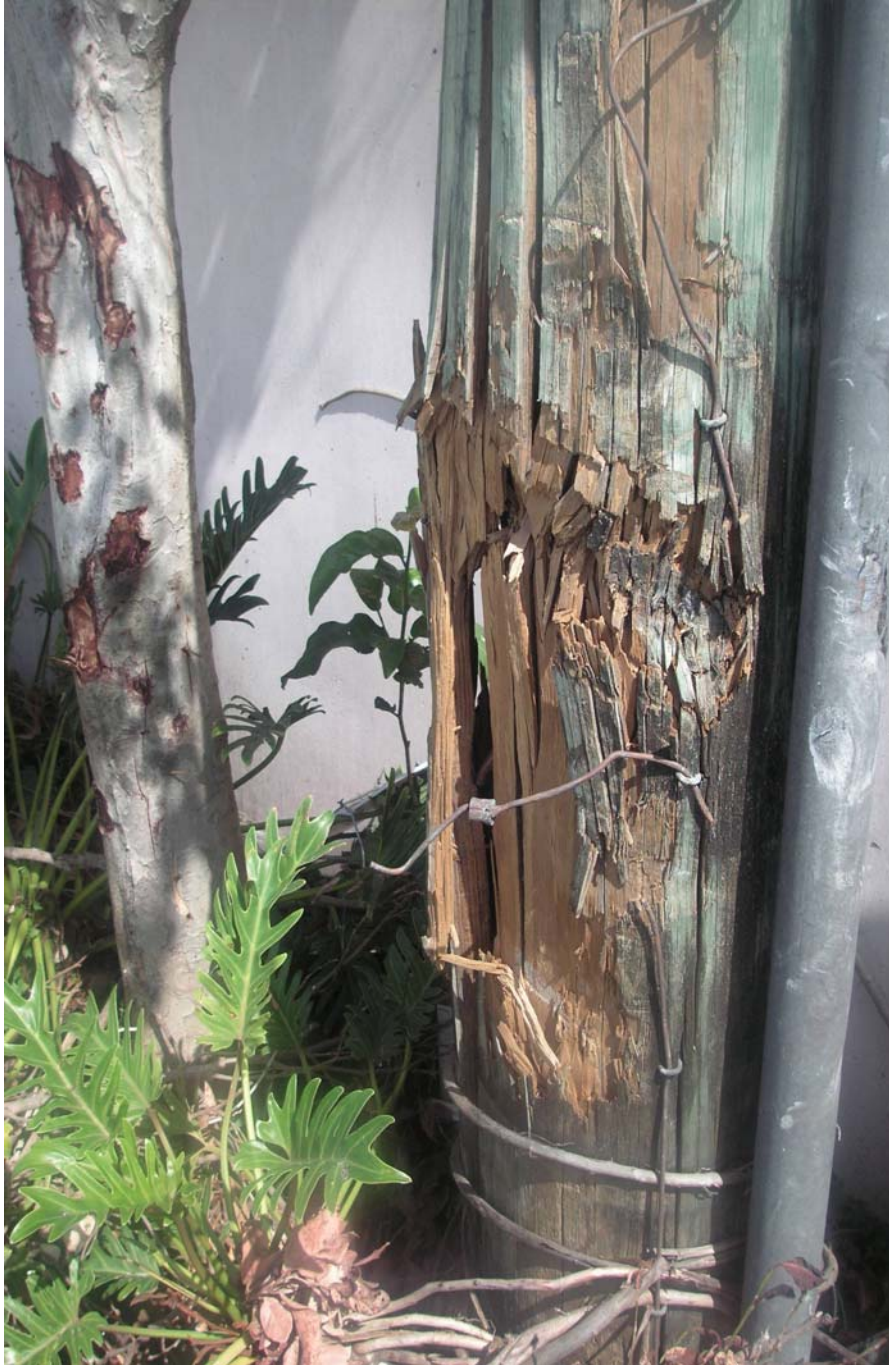
FPL Pole coming apart near ground level. Pole supports a two transformer bank. Pole # 8-6380-9583 2 poles north of NW 8th St. on east side of NW 136th Ave. in Sunrise.
