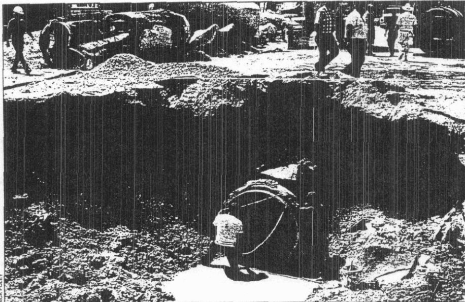
Force main expansion mandate requires construction of 60 miles of new transmission lines.
