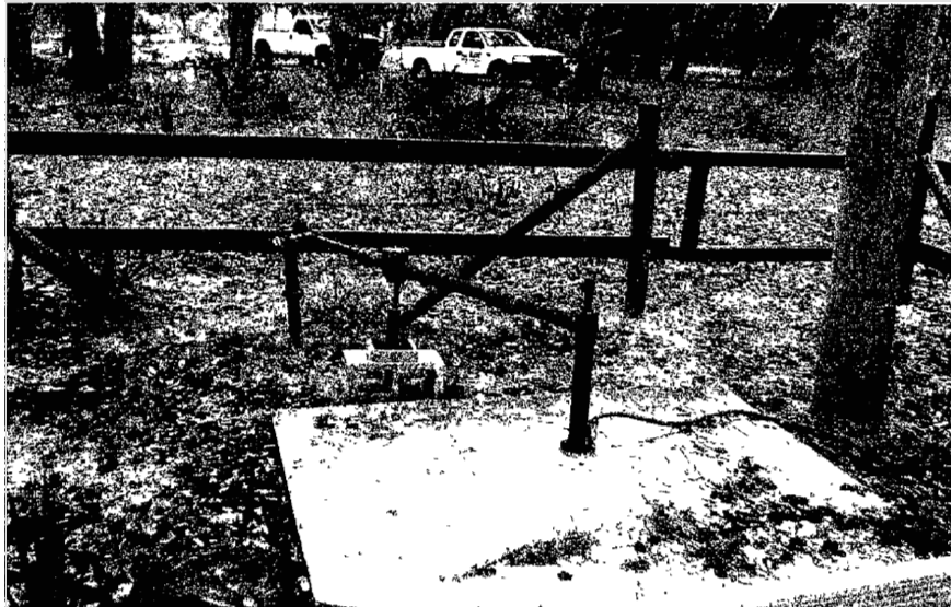
Well No. 2 at the Anclote Water System
