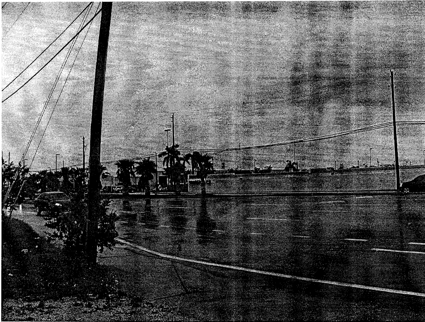
Three bundled cables attached within one foot of space on the pole (against FPL standards). Additionally there are multiple cables coming off the pole at the Sam's club sign (almost mid picture) and tossed together about thirty feet to the right of the pole. All the cables inter-twine at midspan, causing a very large cross-section sail for the wind to catch.
