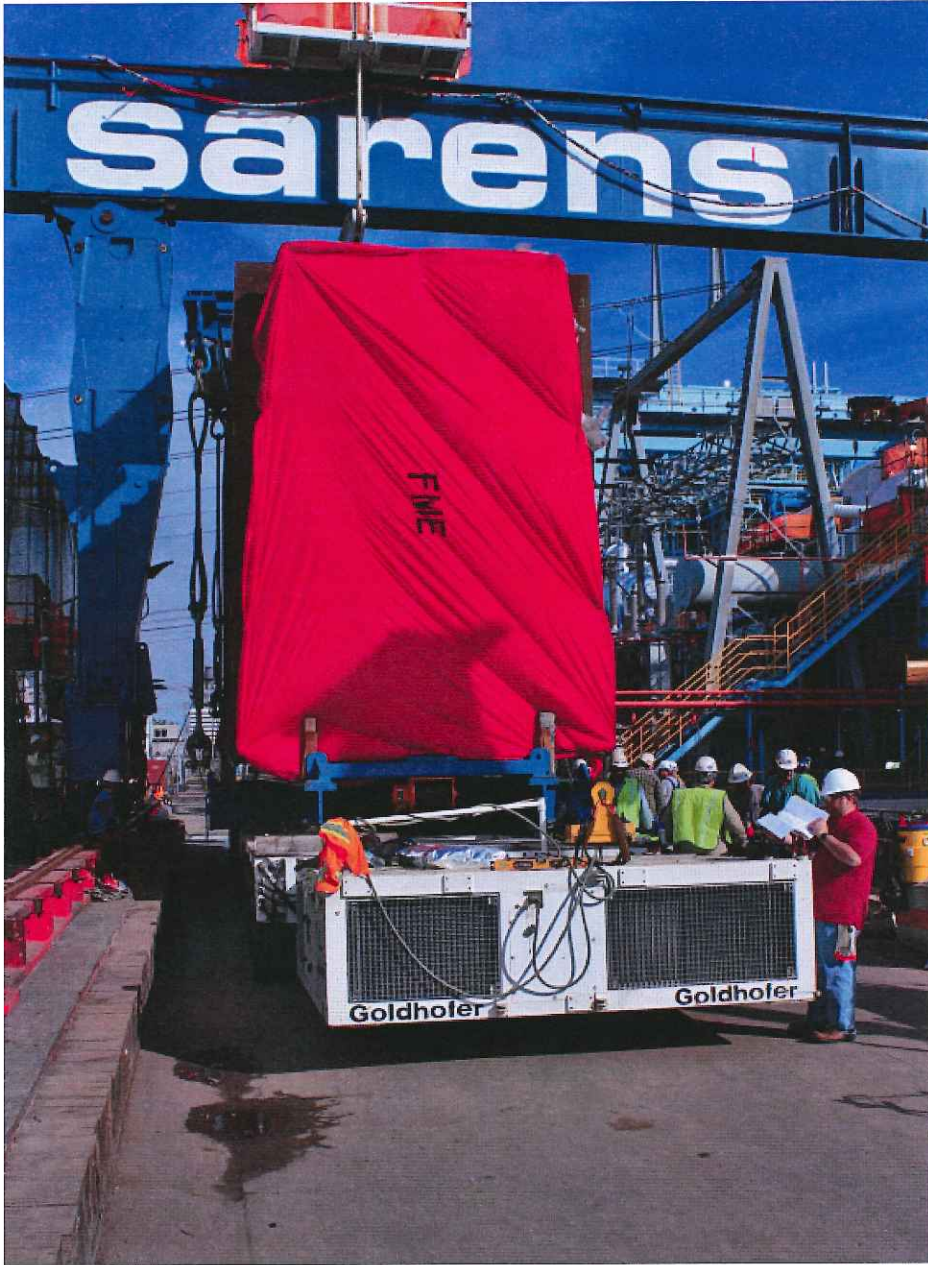
One of the four sections of the main condenser tubes and tube sheets moved into location by the multi-wheeled Goldhofer heavy hauler transporter for lifting by the condenser specialty crane and placement in the condenser pit for installation.
