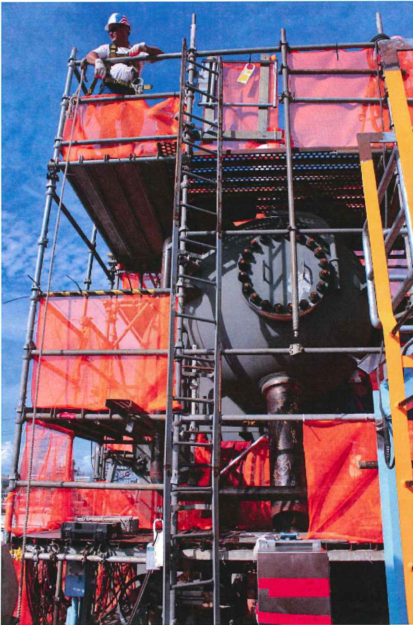
One of the four per unit new larger moisture separator reheaters in place on the turbine deck with scaffolding installed to support installation of the unit which includes installing and welding large diameter piping, relief, safety, and control valves, piping and valve supports, and instrumentation.
