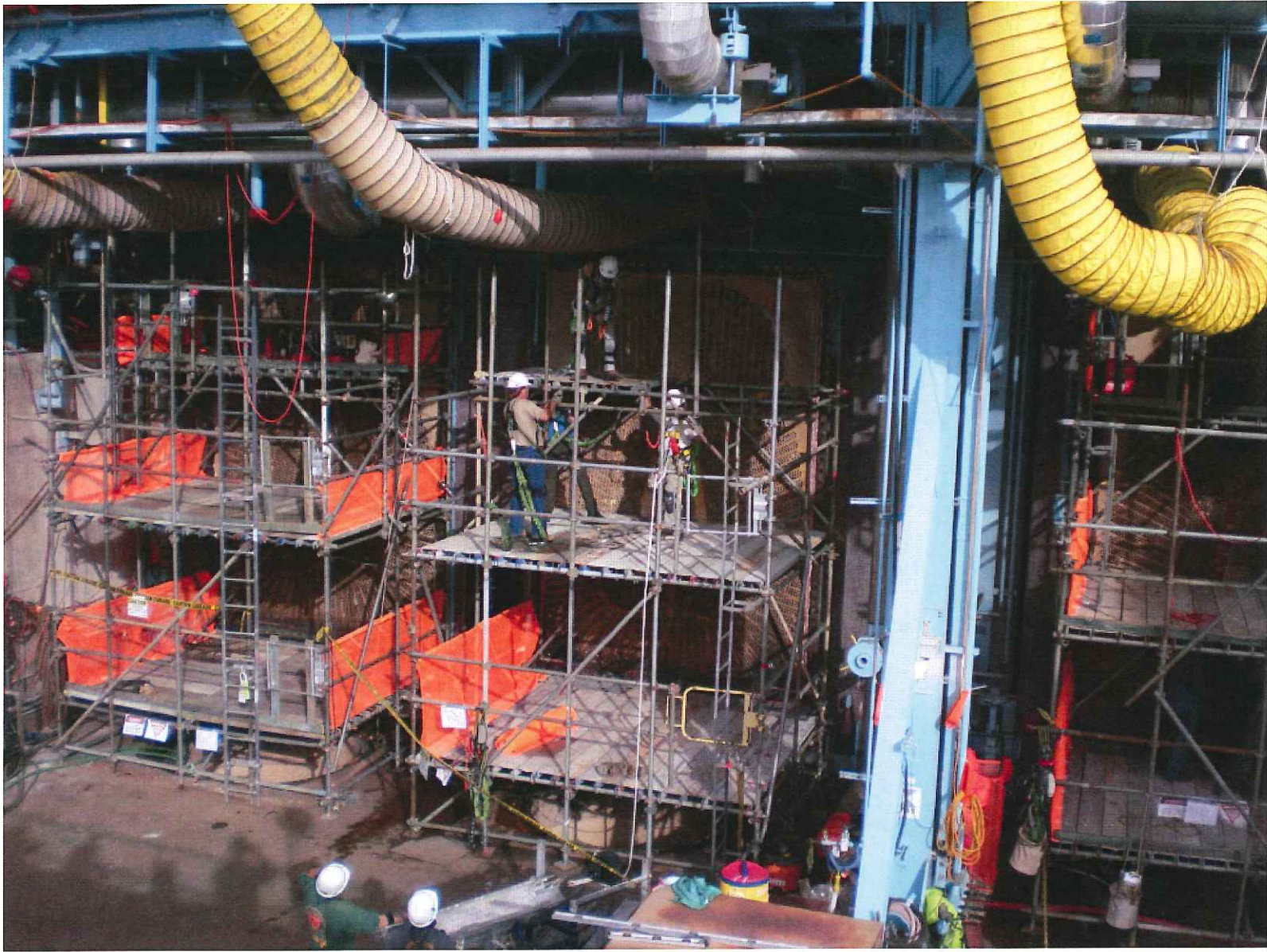
Scaffolding being erected to support the removal of the condenser tube sheets and tubes.
