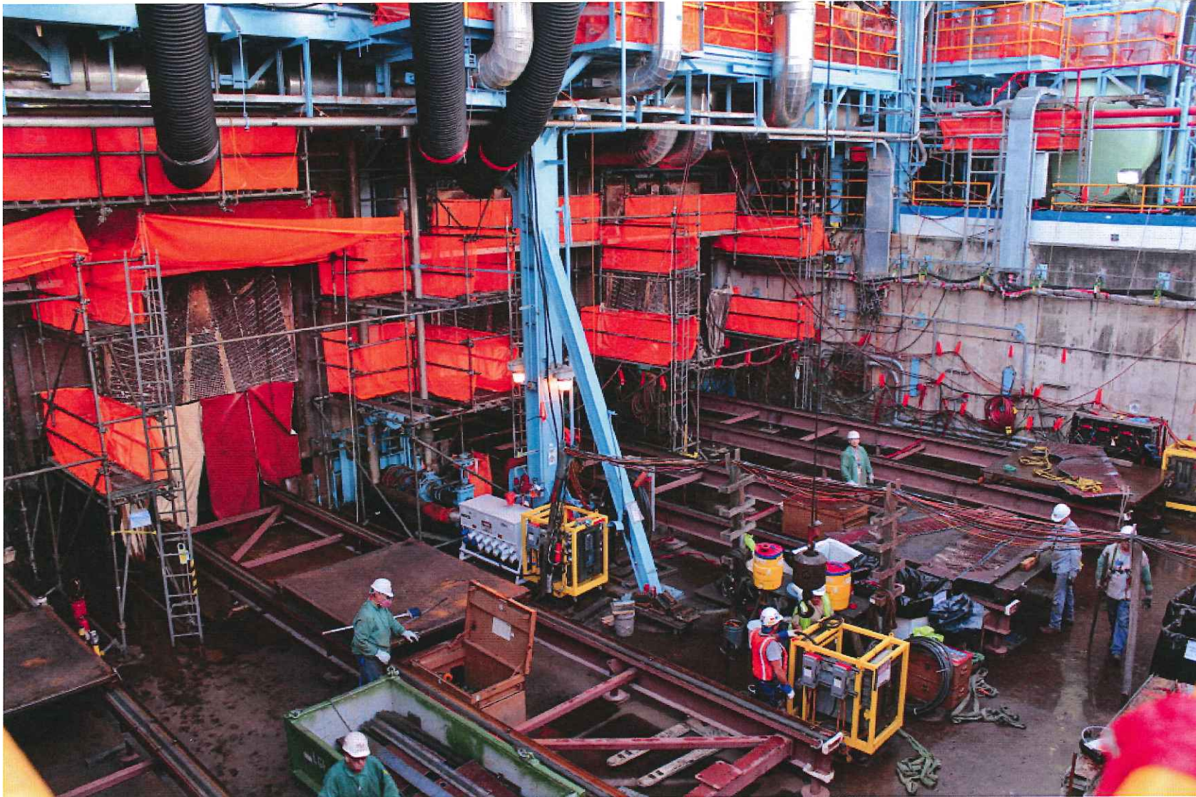
Condenser tube sheets and tubes being removed. Rails were erected to provide equipment access to the over 40 feet of tubes and tube sheets for removal and installation of the new larger condensers.
