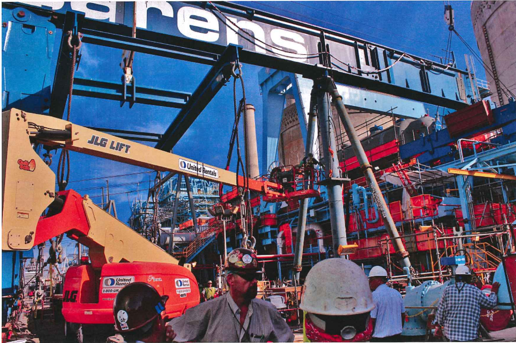
A specialty crane (blue SARENS) was installed to support the removal of the old condenser and tube sheets and the installation of the new larger condensers. One of the four new larger moisture separator reheaters (gray) is installed on the main turbine deck.
