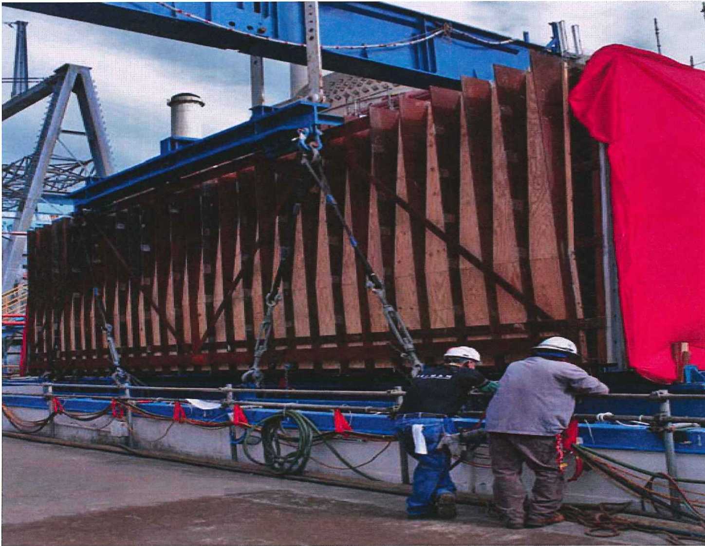
One of the four sections per unit of the main condenser being lowered by the specialty crane into the condenser pit area for installation into the condenser shell. Note the many dark brown steel tube sheets which are used to support the thousands of condenser tubes.
