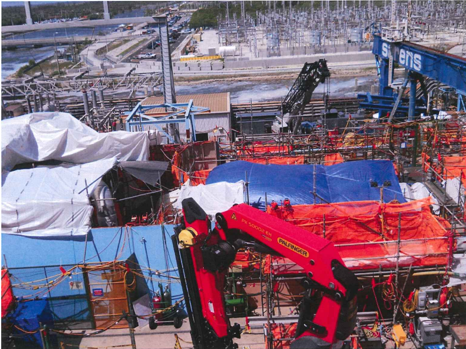
Near the top of the photo the blue colored specialty crane and staging area for condenser removal and replacement. The white and blue tarps are used to protect the equipment on the main turbine deck. The orange colored material on the elevated scaffolding protects workers.
