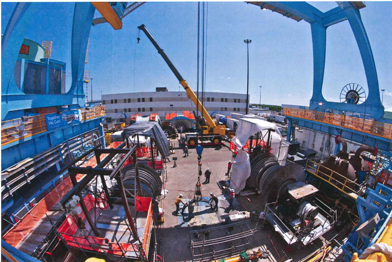
A fisheye view of the turbine deck ground storage and staging area. The blue turbine deck crane accesses the staging area lowering a turbine bearing to the ground. The two low pressure turbine rotors are staged in their respective storage stands. Temporary cranes are used to move equipment into and out of the turbine deck crane ground access area.
