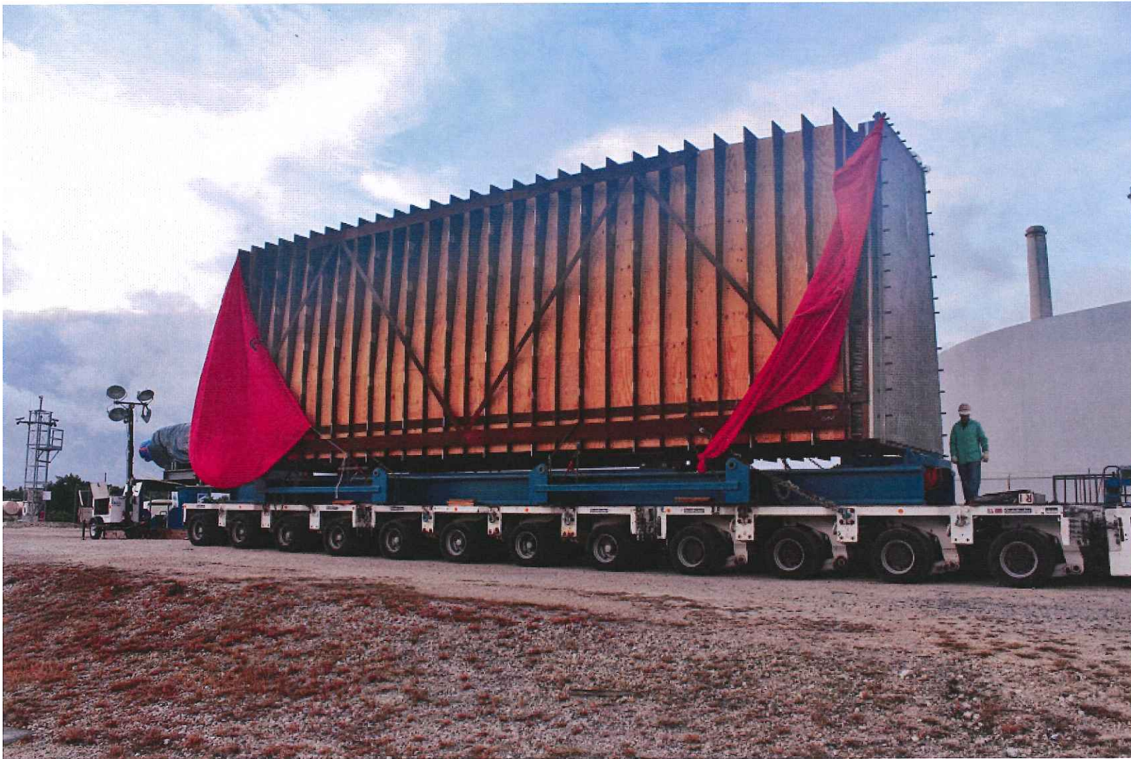
One of four sections per unit of the new main condenser on its heavy hauler being transported to the condenser pit staging area, where the specialty crane will lift it into the condenser pit for installation.
