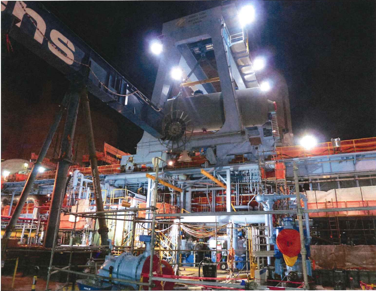
One of the four per unit new larger moisture separator reheaters being lifted by the turbine deck crane onto the turbine deck for installation. The large blue structure (upper left) is the special crane built for condenser replacement.
