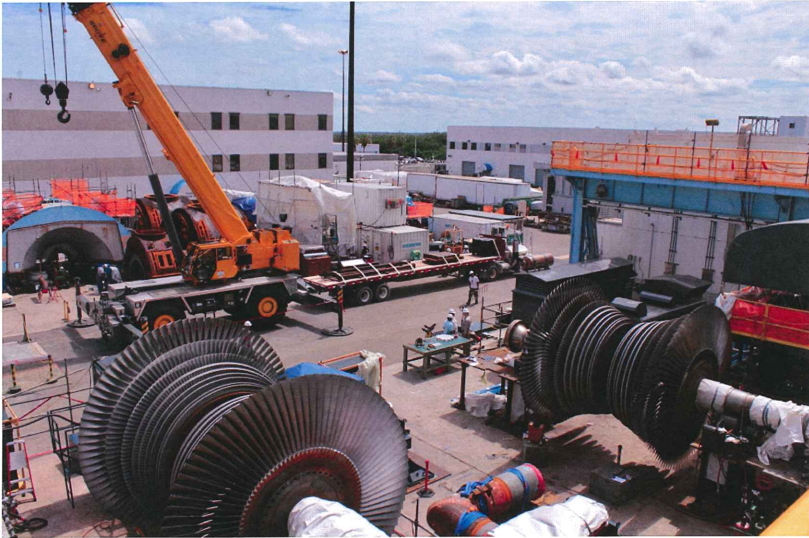
The turbine deck ground storage and staging area with a temporary crane unloading materials from a tractor trailer, behind the temporary crane, the brown main turbine high and low pressure casings being stored, behind the tractor trailer, several white containers and trailers with tools and equipment, and in the access area, the two low pressure turbine rotors in their respective storage stands.
