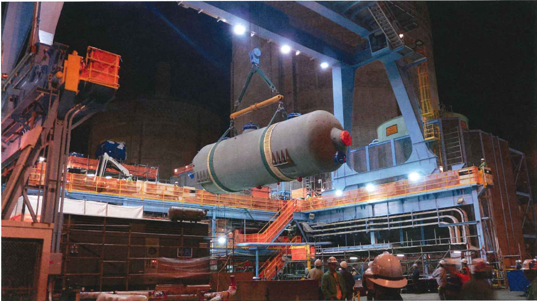
One of four per unit new larger moisture separator reheaters being lifted from the turbine deck crane ground access area onto the turbine deck for installation.
