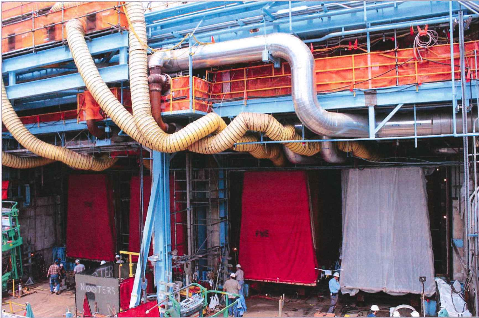
The four sections of the main condenser installed and the condenser pit area rail system removed. Workers making preparations for the reinstallation of the condenser outlet water boxes.
