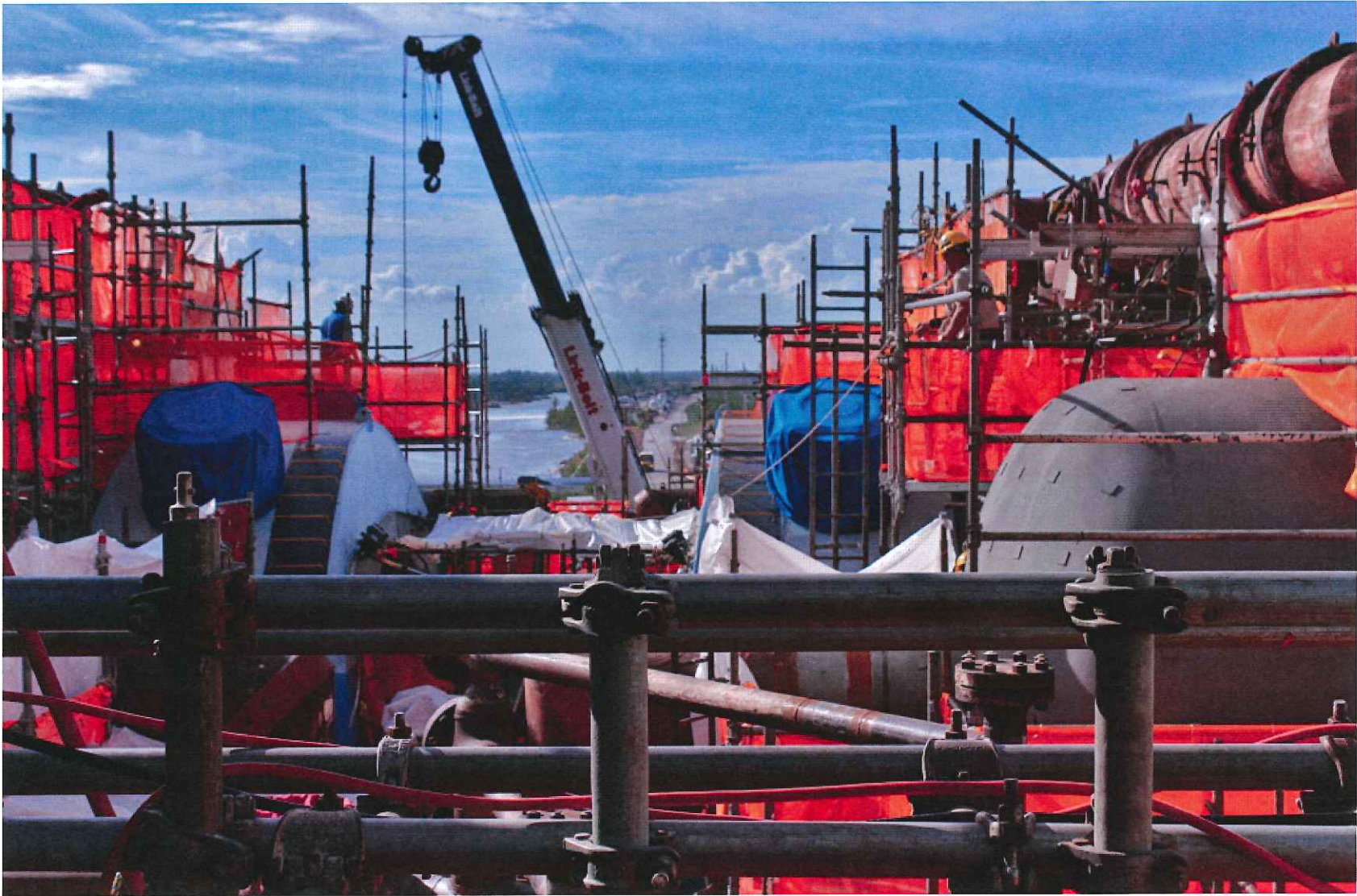
Workers on scaffolding which was erected on the turbine deck to support the installation and removal of equipment.
