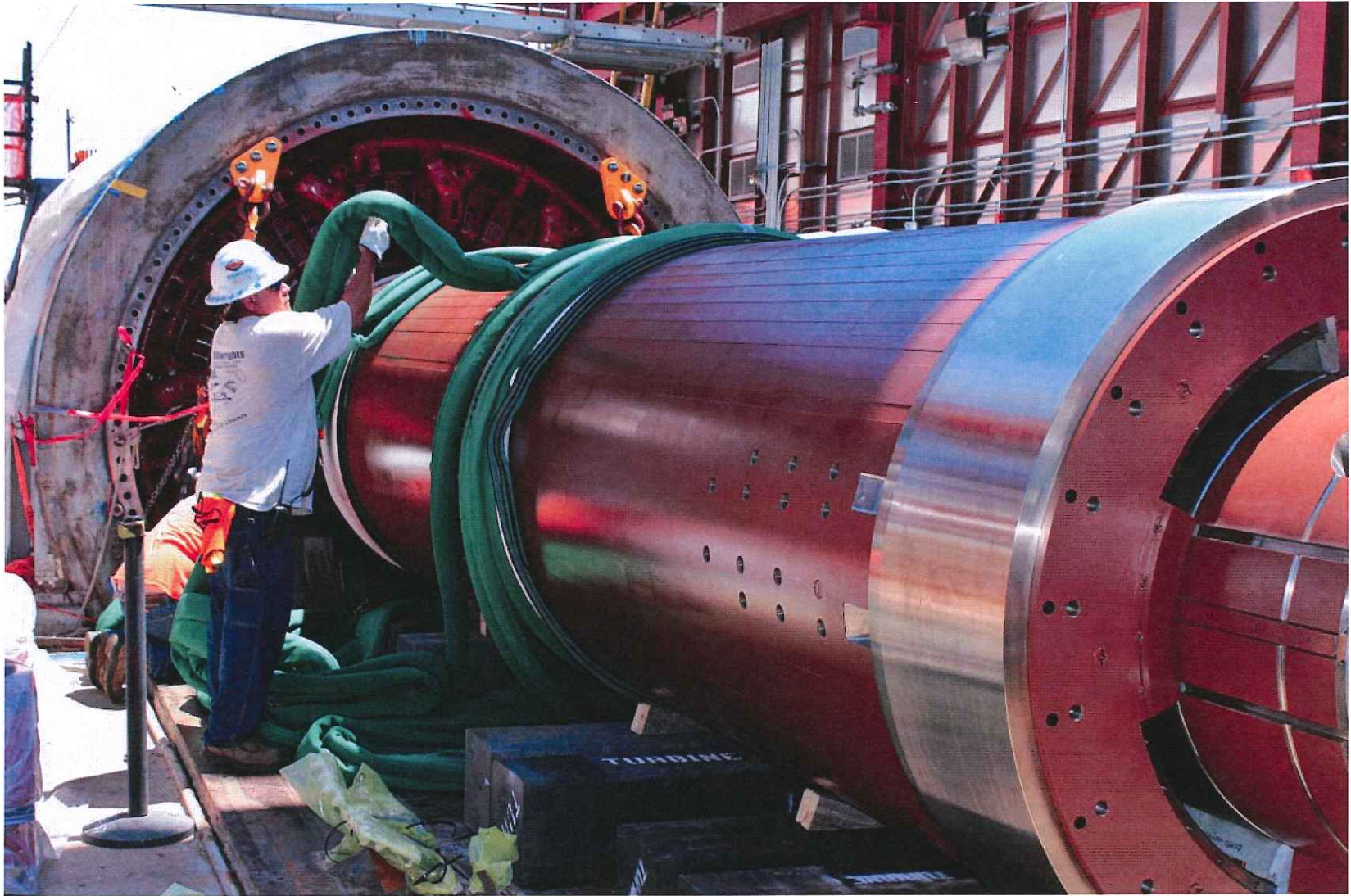
The main generator rotor staged on the turbine deck and being readied for installation into the main generator stator.
