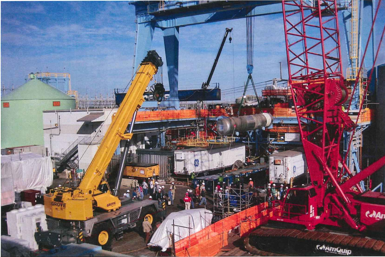
The turbine deck crane in the equipment access area lowering a feedwater heater to the blue transporter. Temporary cranes are used to move equipment into and out of the turbine deck crane access area. The white trailers in the staging area protect equipment and tools until they are installed or needed for use.
