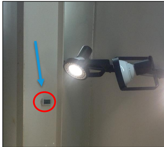
Figure 9. Lighting Logger Installed to Measure the Operating Hours of LED Spotlights
