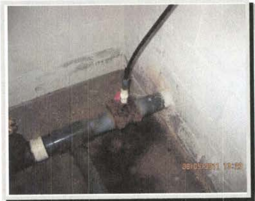
Chlorine injection point is rusted and leaking
