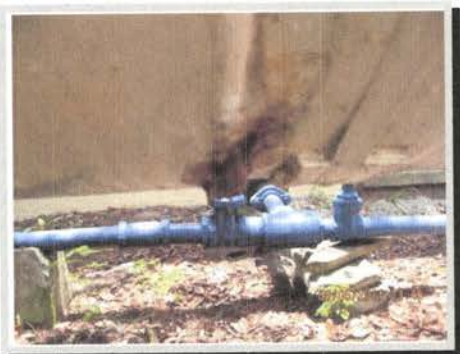
Leak on the underside of storage tank
