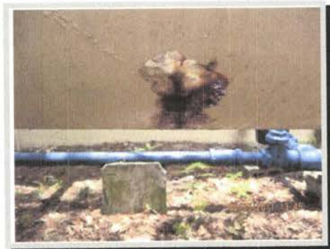
Leak on the underside of storage tank
