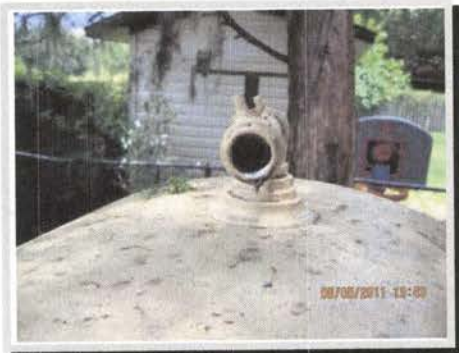
Pressure relief valve on tank needs screen
