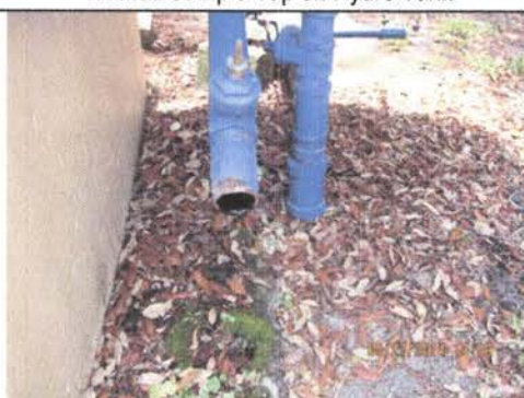
Tank Drain Pipe with bio-growth
