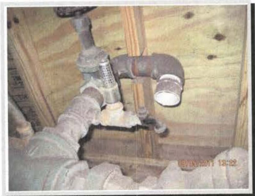
Well #1 (AAB4607) - well casing vent needs screen
