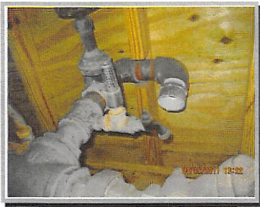
Well #1 (AAB4607) - well casing vent needs screen
