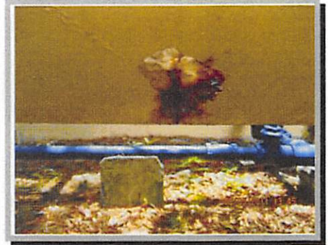
Leak on the underside of storage tank
