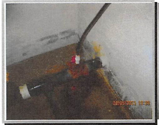
Chlorine injection point is rusted and leaking
