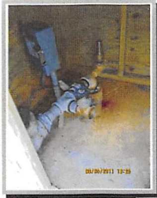
Well #2 (AAB4608) - well casing vent needs screen
