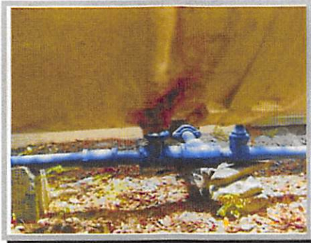
Leak on the underside of storage tank
