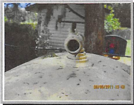
Pressure relief valve on tank needs screen
