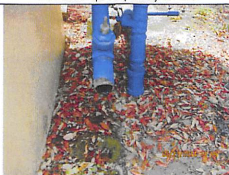
Tank Drain Pipe with bio-growth
