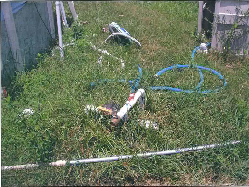
Photograph No. 11. View of the pool's pump system.
