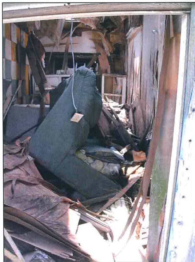
Photograph No. 38. View of the interior of one of the demolished trailers located on the western portion of the subject property.
