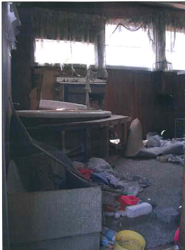
Photograph No. 37. View of the interior of one of the demolished trailers located on the western portion of the subject property.
