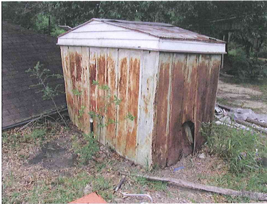
Photo Number 03: View of the Pump House on the Comalander Parcel. (No suspect asbestos-containing materials)
