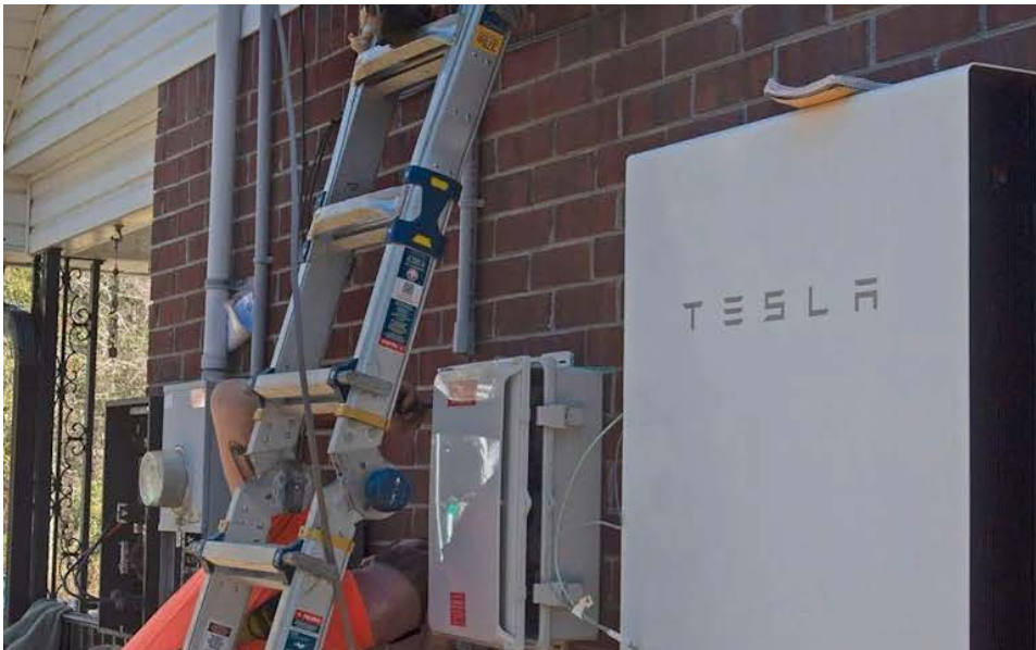
Sun Farm Energy workers install solar energy system on a home in Escambia County on Feb. 8.
