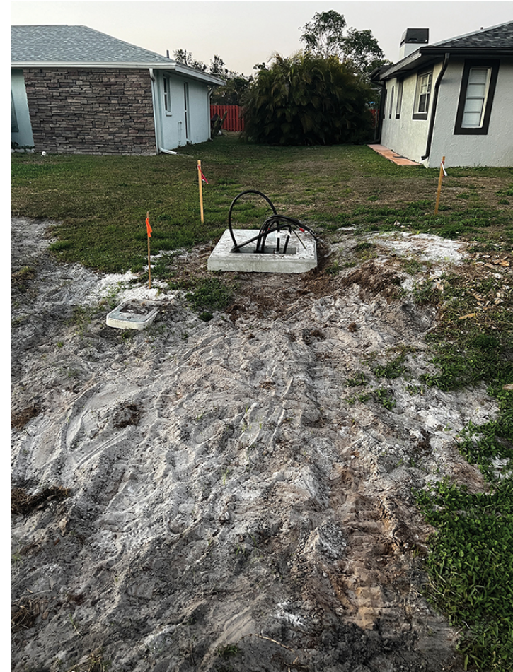
1. Underground power lines are more reliable than overhead lines, particularly during hurricanes and severe weather. Florida Power and Light says it has been installing underground service for decades and has about 45% of its distribution system underground today. The work shown here was done in Port Charlotte, Florida, after Hurricane Ian. Source: POWER
