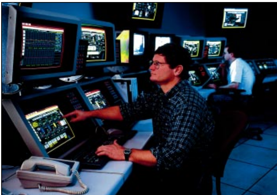
Polk Power Station control room
