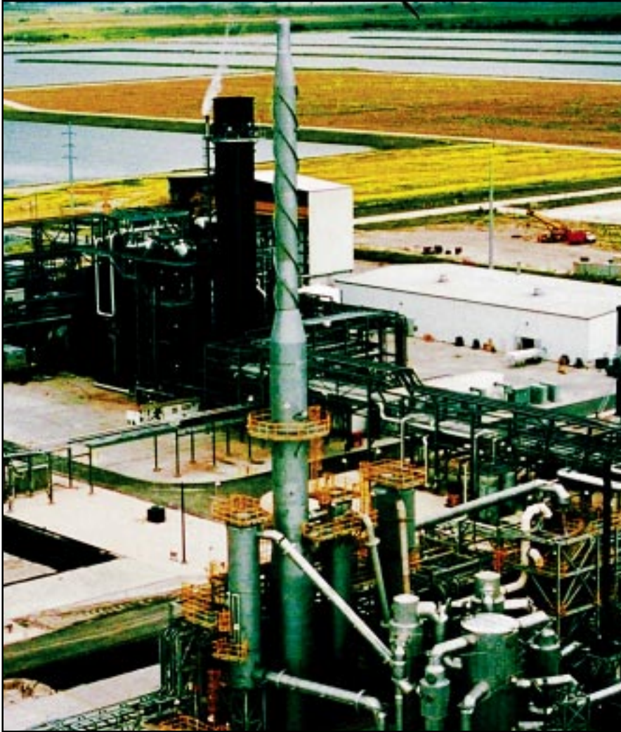
The sulfuric acid plant is in the foreground and the combined-cycle unit is in the background. The large black object (left center) is the heat recovery steam generator
