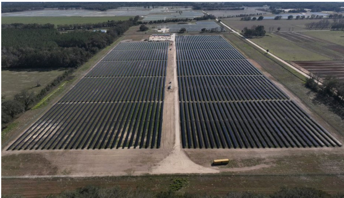
FIGURE 3.3 Hardeetown Solar Power Plant
