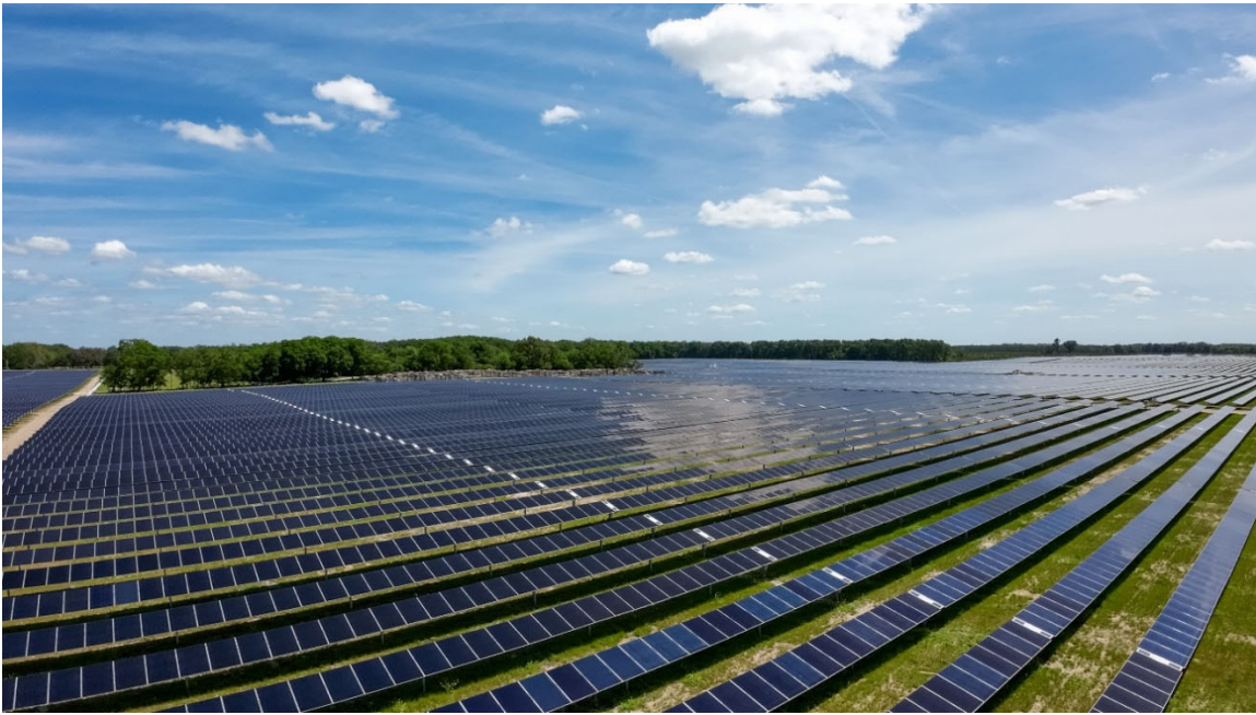
FIGURE 3.4 High Springs Solar Power Plant
