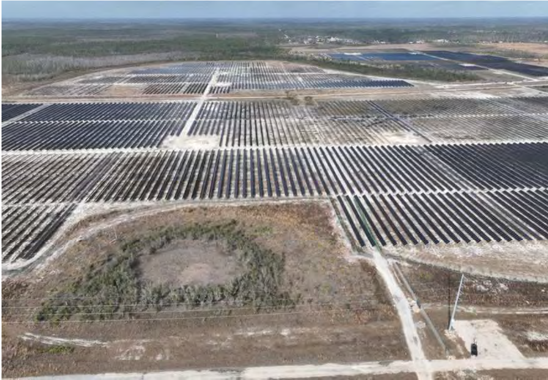
FIGURE 3.2 Bay Ranch Solar Power Plant
