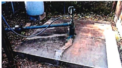
Photo 1: Well #1 Well Pad
