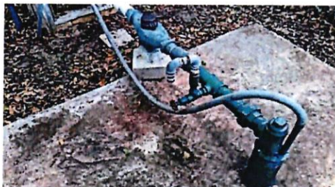
Photo 1: Casing Vent with No Screen
