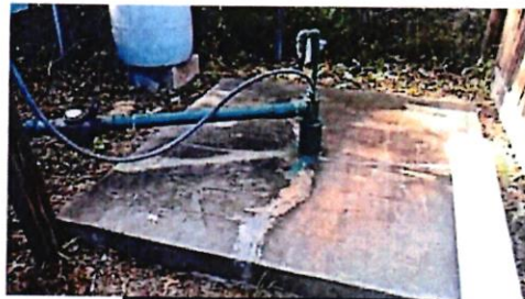
Photo 1: Well #1 Well Pad
