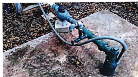
Photo 1: Casing Vent with No Screen
