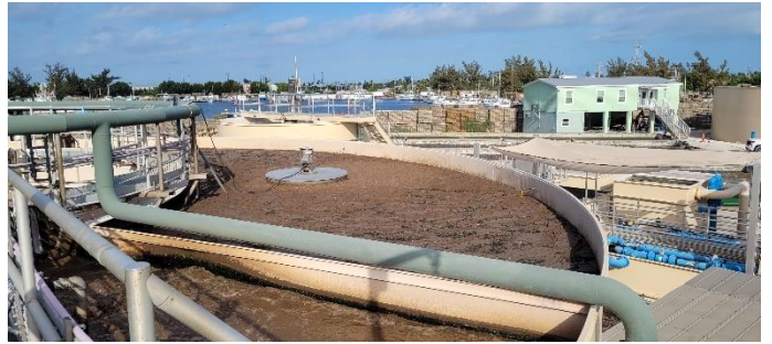
Dual train aeration and anoxic tank
