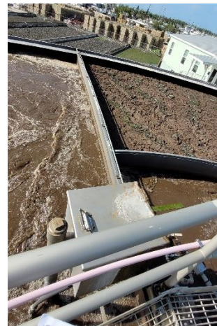
Train 3 aeration and anoxic tank
