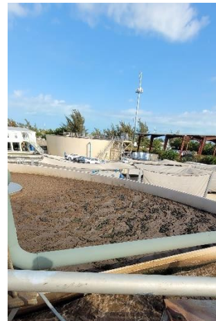
Dual train reaeration tank
