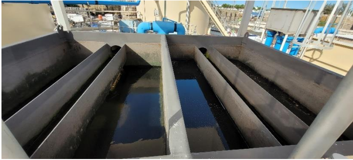
Chlorine contact chamber
