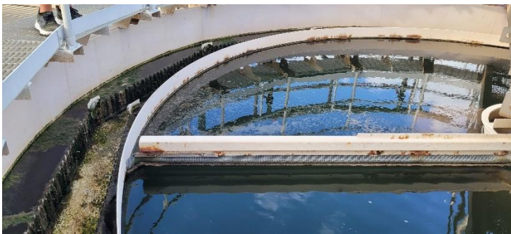
Dual train clarifier
