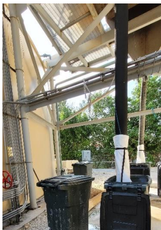
Dual train grit and screening collection
