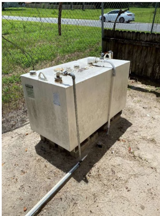
Figure 2-12: Emergency Generator Diesel Fuel Tank
