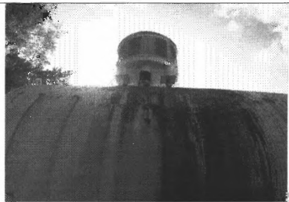
Corrosion on Wall from Aerator
