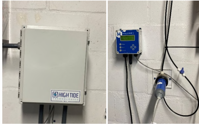
Remote monitoring unit (left) and continuous chlorine monitor (right) installed at Neighborhood Utilities
