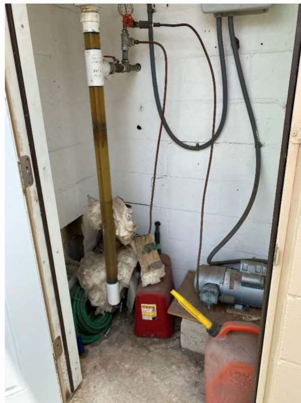
Figure 2-8: Hydropneumatic Tank Sight Gauge and Air Compressor
