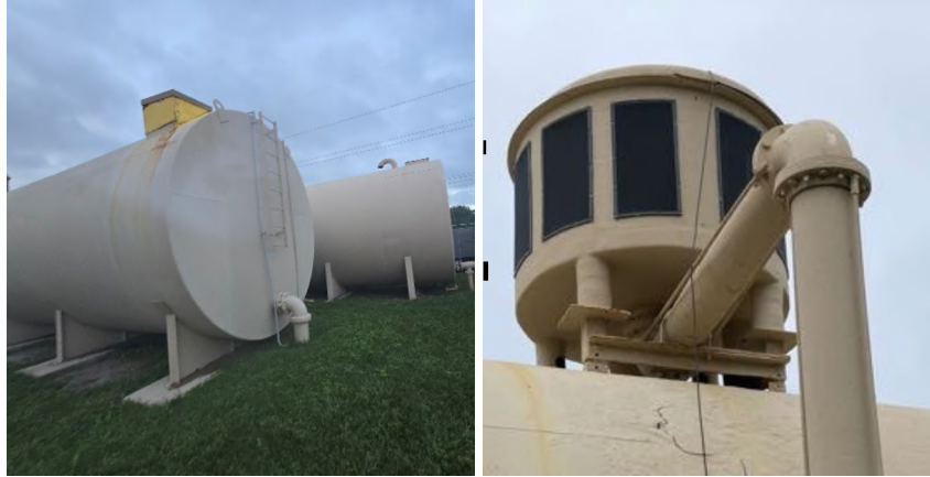
Tanks 1 & 2 (left) to be replaced with a single larger ground storage tank; and aeration treatment unit (right) to be replaced
