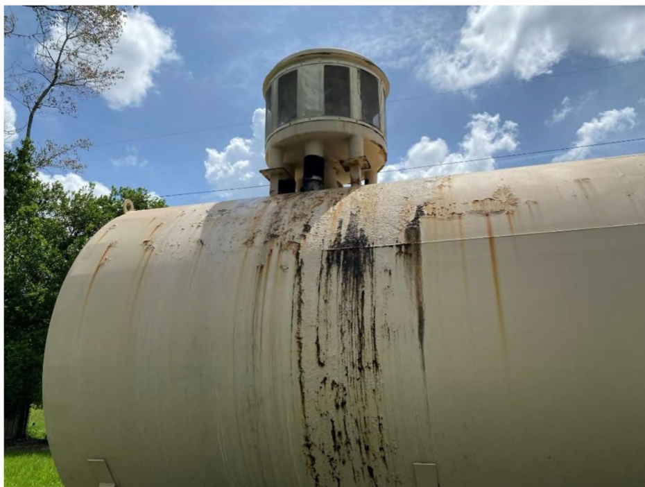
Figure 2-16: GST2 Exterior Corrosion
