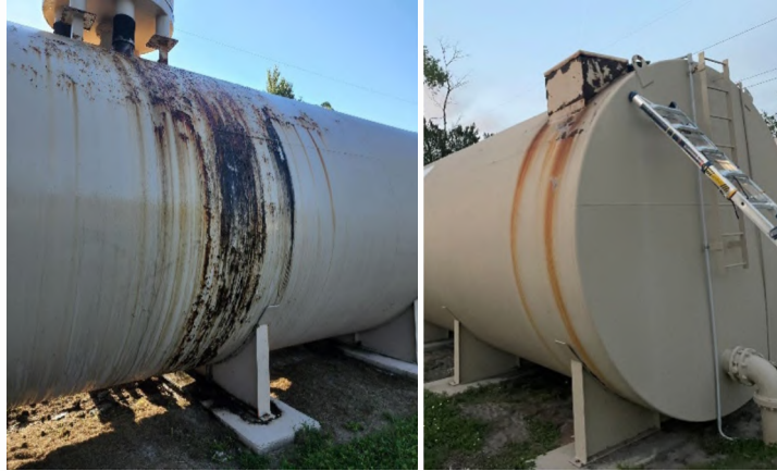
Examples of rust on the ground storage tanks and general poor condition.
