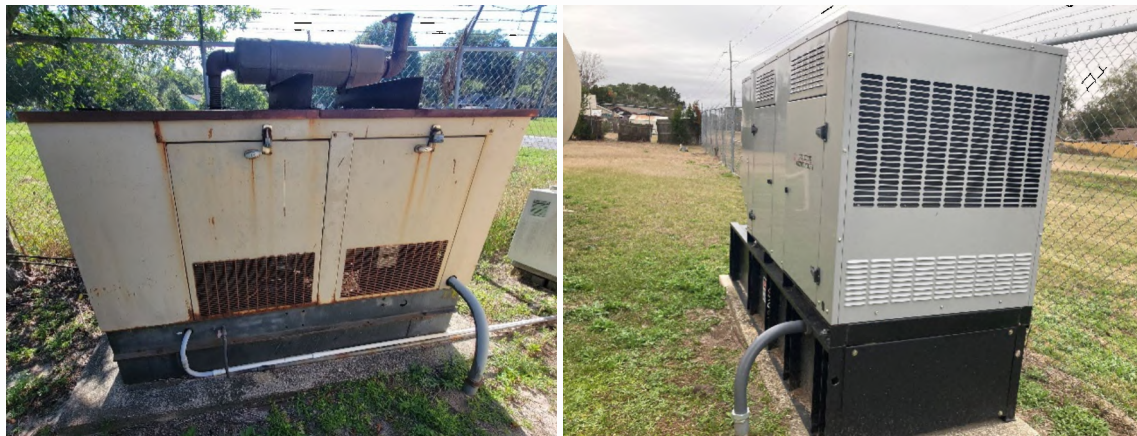
Emergency generator at Neighborhood Utilities before (left, nonfunctional) and after (right) replacement
