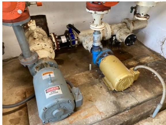
Booster pumps in need of replacement - note empty pump flange from pump which failed since acquisition by CSWR-Florida, emphasizing the poor condition of the pumps
