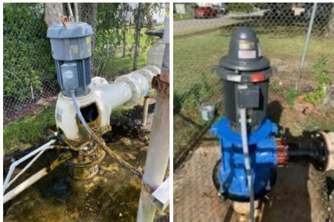
Well 2 pump before (left) and after replacement (right). The well casing and wiring were also replaced.
