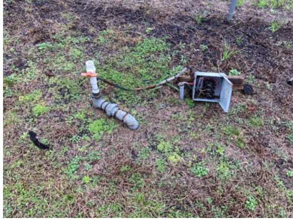
Well 1 needs to be properly decommissioned and removed.
