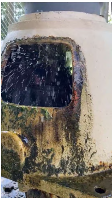
Figure 2-13: Pump Water Leak
