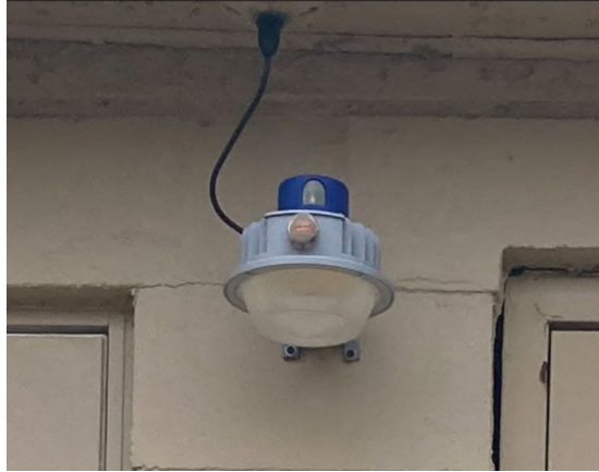
New flood lighting
