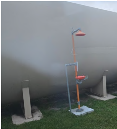
New emergency eye wash station and chemical shower
