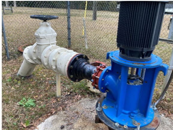
Well 2, new piping needs to be painted, flow meter needed, etc.
