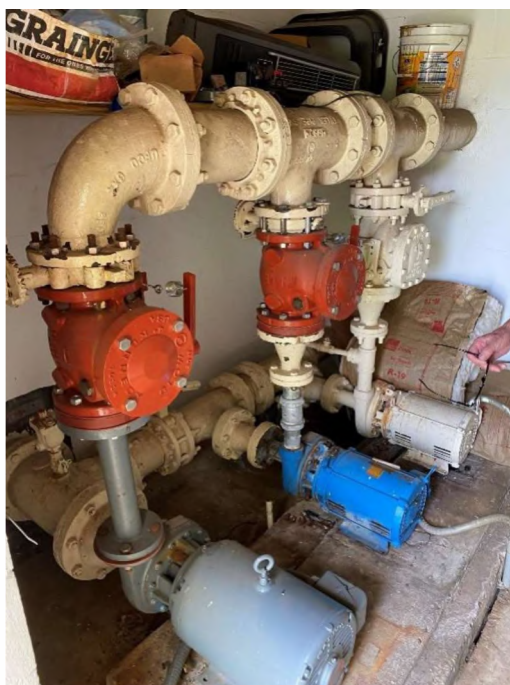
Figure 2-9: High Service Pumps
