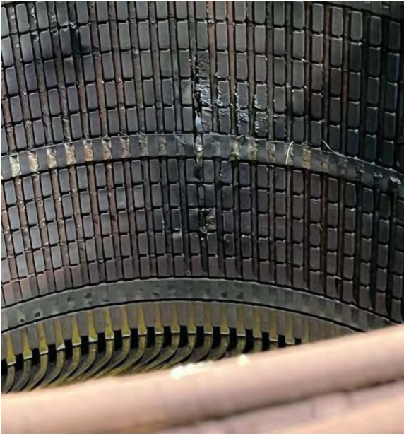
Stator points of failure
