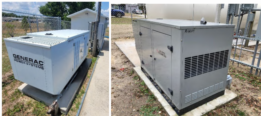
Backup generation at CSWR Florida systems.
