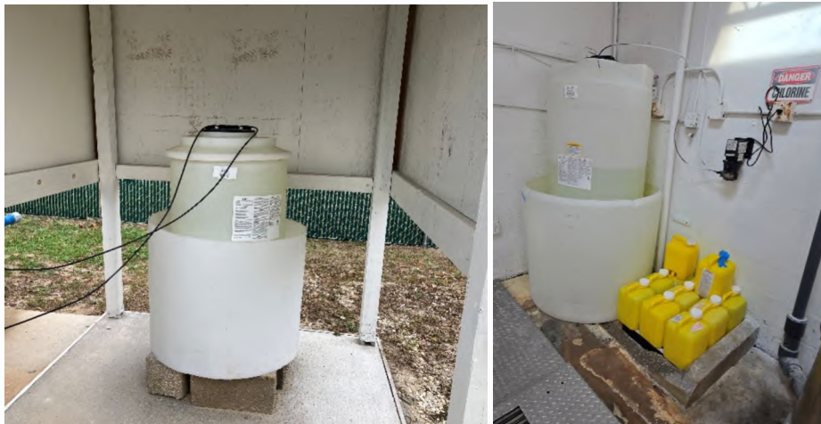
Liquid Chlorine Spill Containment Measures
