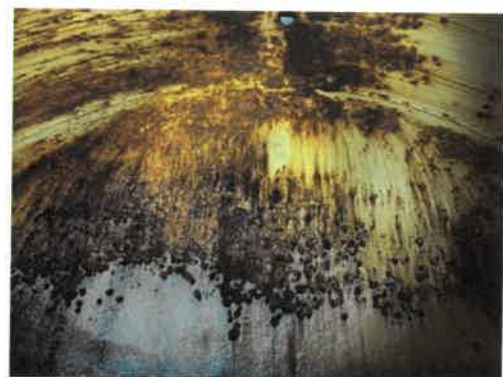
Hydropneumatic tank #1 interior
