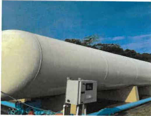
Hydropneumatic tank #1 exterior
