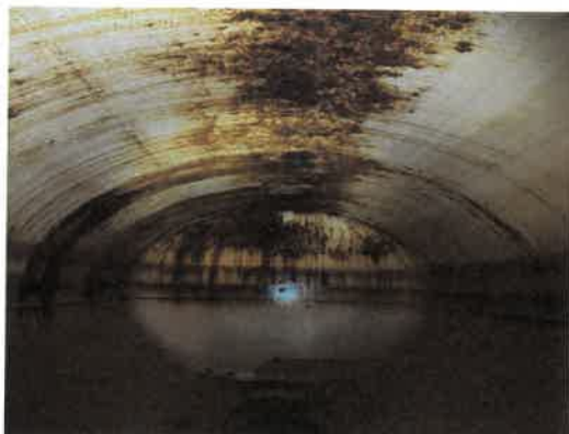
Hydropneumatic tank #1 interior
