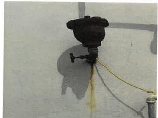
Corroded relief valve on rear of tank #1
