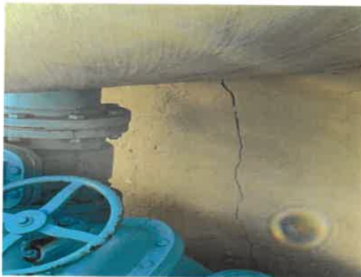
Front concrete footer cracked in half
