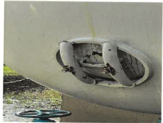
Hydropneumatic tank #1 manway
