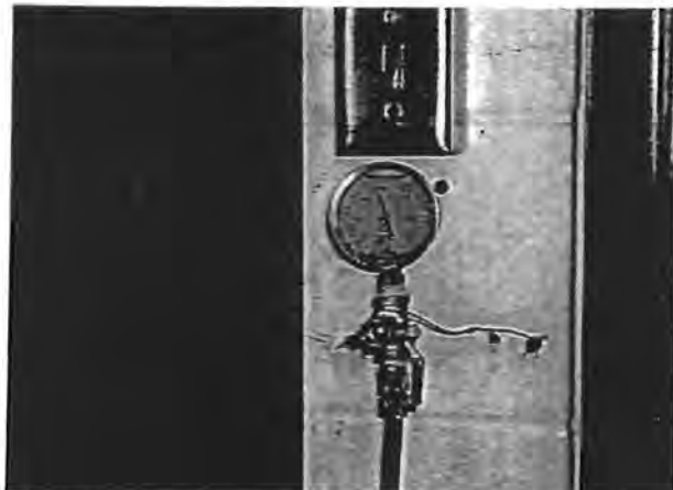
Fire System pressure at pump building 137 PSI
