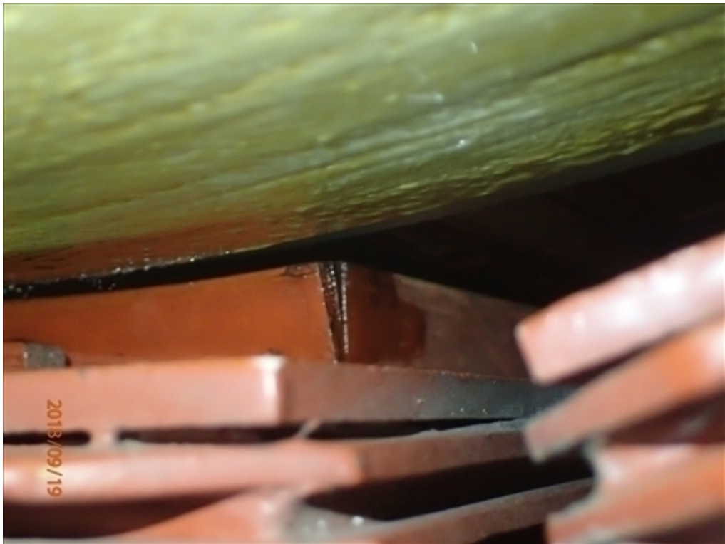
2.24 Typical Repair for Damaged Exciter Stator Pole Iron
