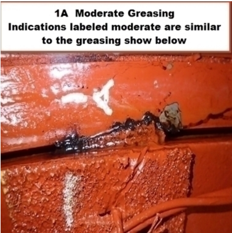
2.5 Turbine End Tuning Weight Inspection Moderate Greasing
