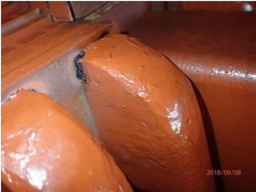
2.8 Worse Case for Greasing / Overheating Noted on Exciter and Turbine End Finger Plate Heavy Sheets
