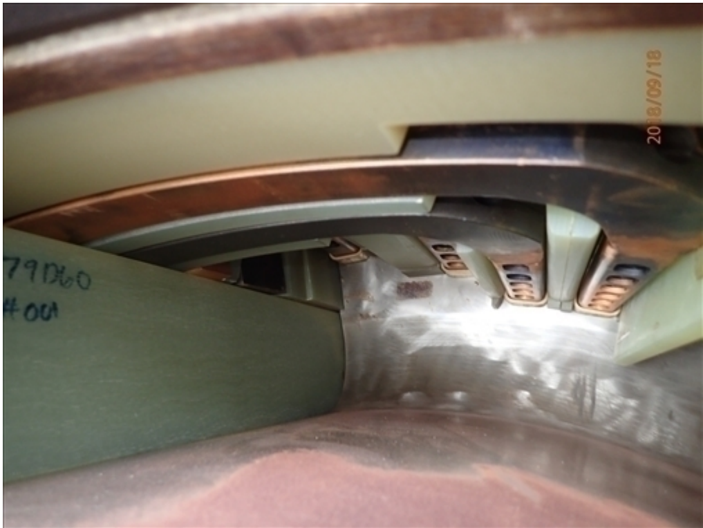
2.2 Typical Condition of Rotor Windings
