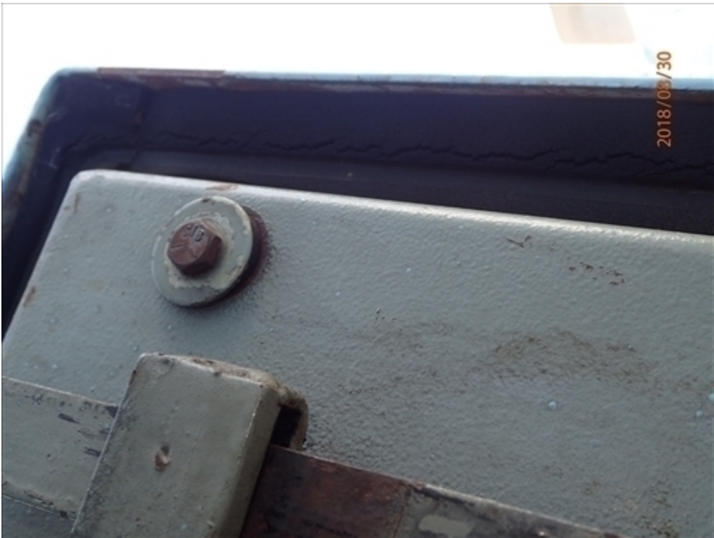
2.21 Weather Cracking on Exciter Dog House Door Gasket material
