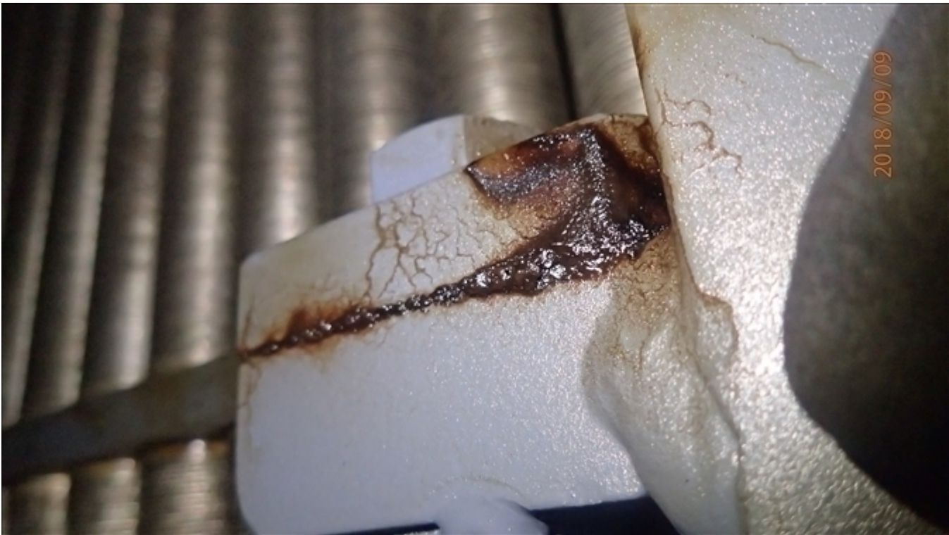
2.12 Grease On Bolts in Upper Cooler Bay Inspection
