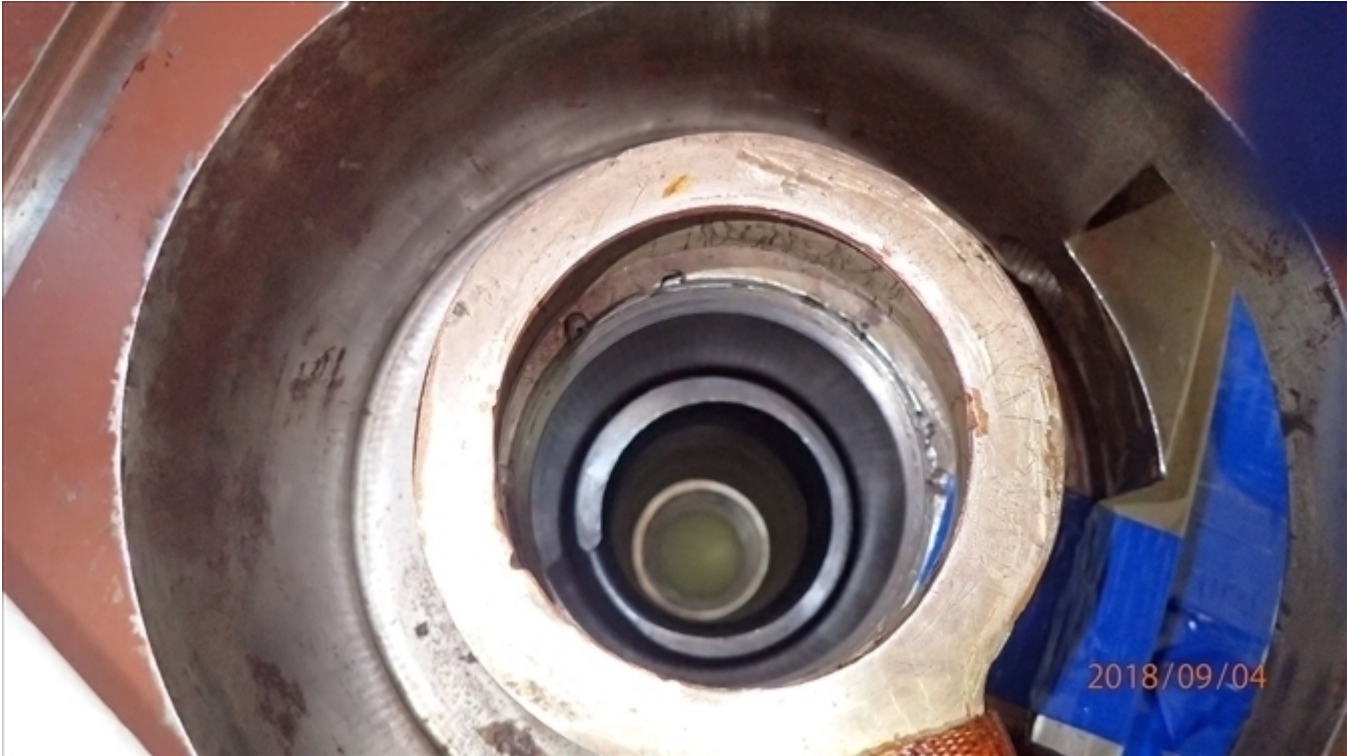
2.1 As Found Condition of Gen Rotor Radial Lead P1
