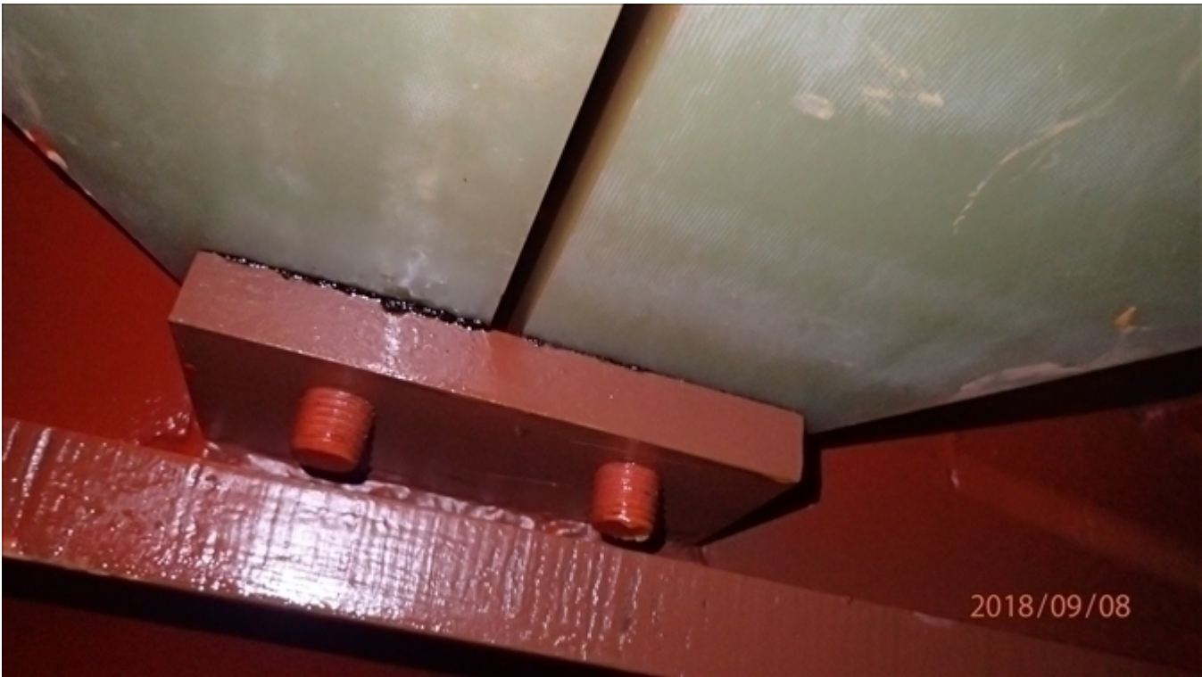
2.13 Typical Greasing on Exciter end Upper Cleats
