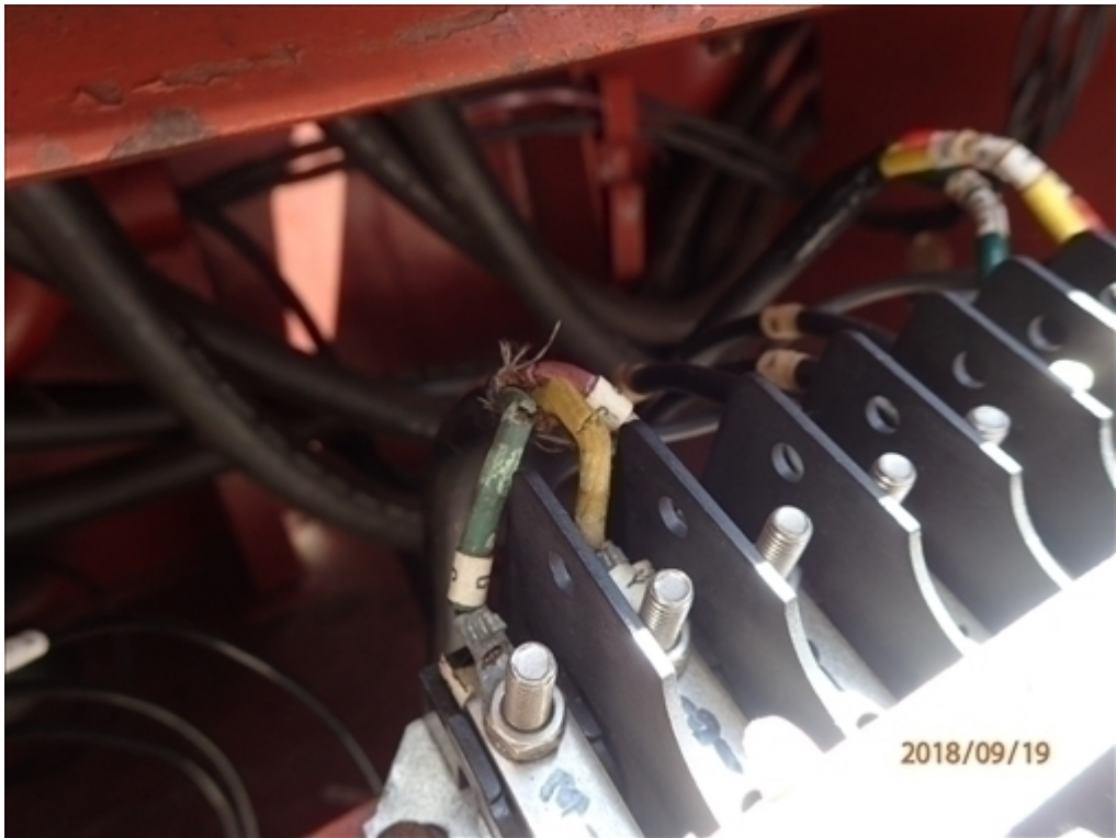
2.19 Exciter RTD Wires Chafed
