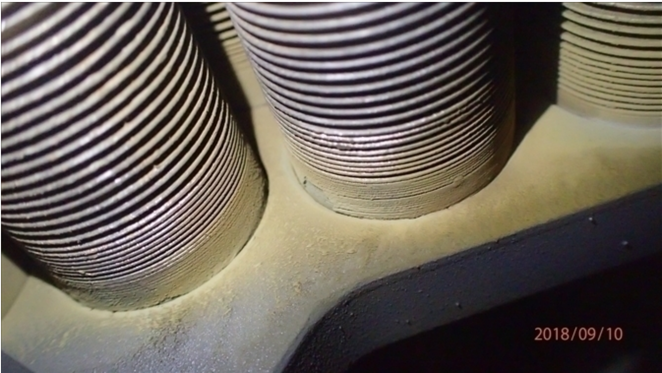
2.11 Possible Lead Carbonate Found in Generator Coolers
