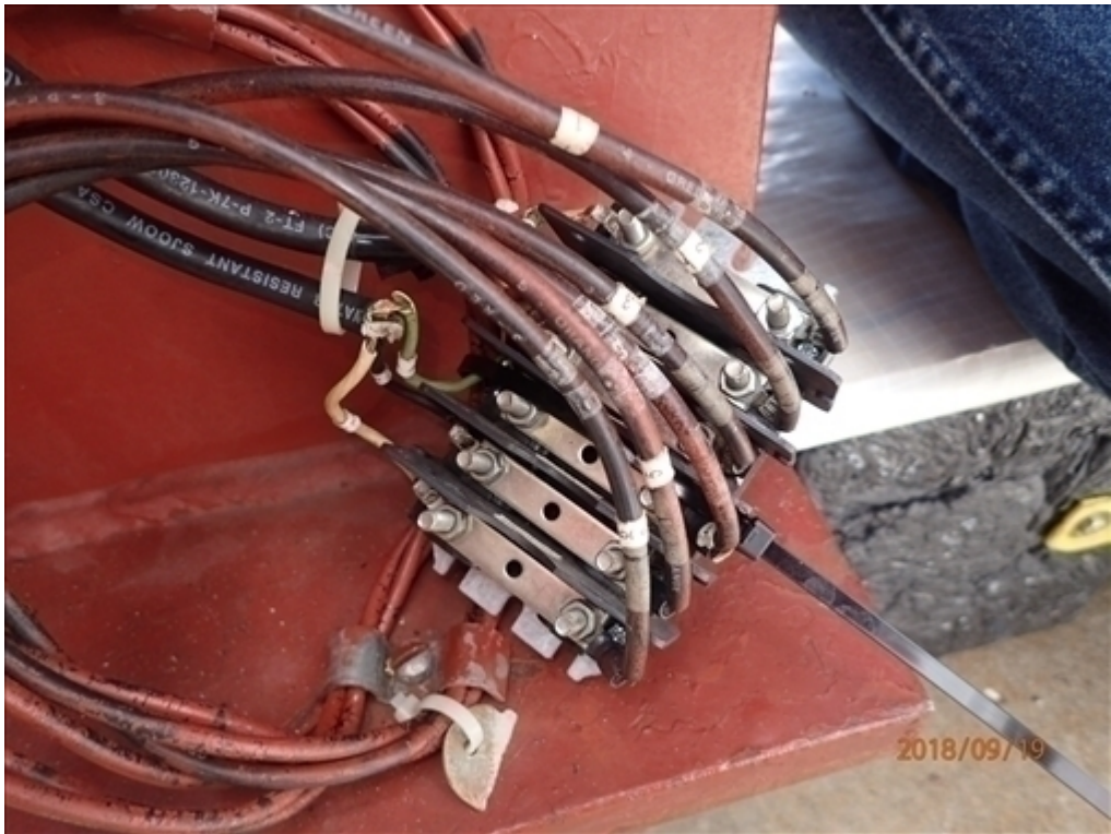
2.18 Exciter RTD Cables Chafed on Intermediate Terminal Board
