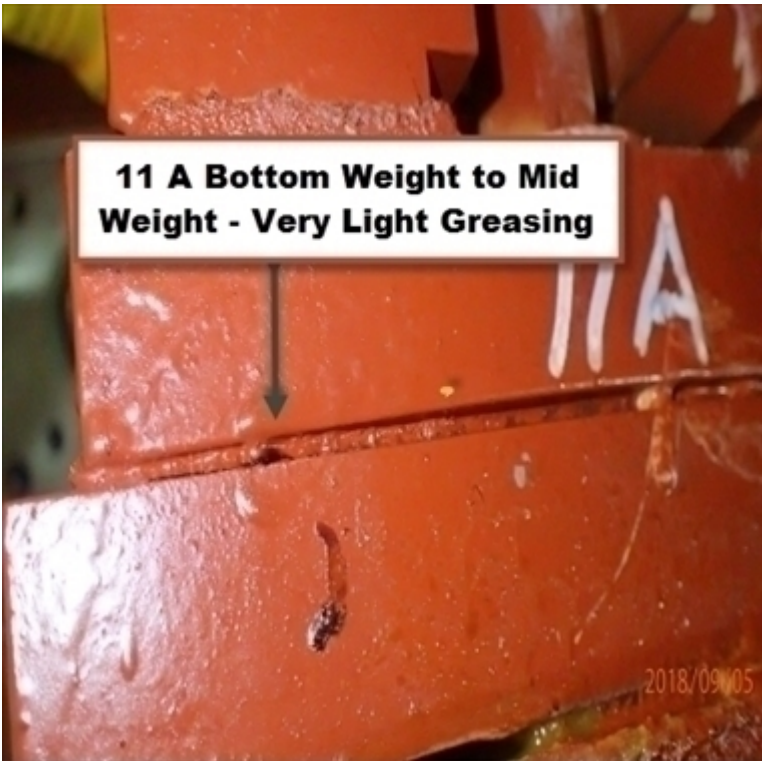
2.7 Turbine End Tuning Weight Inspection Very Light Greasing
