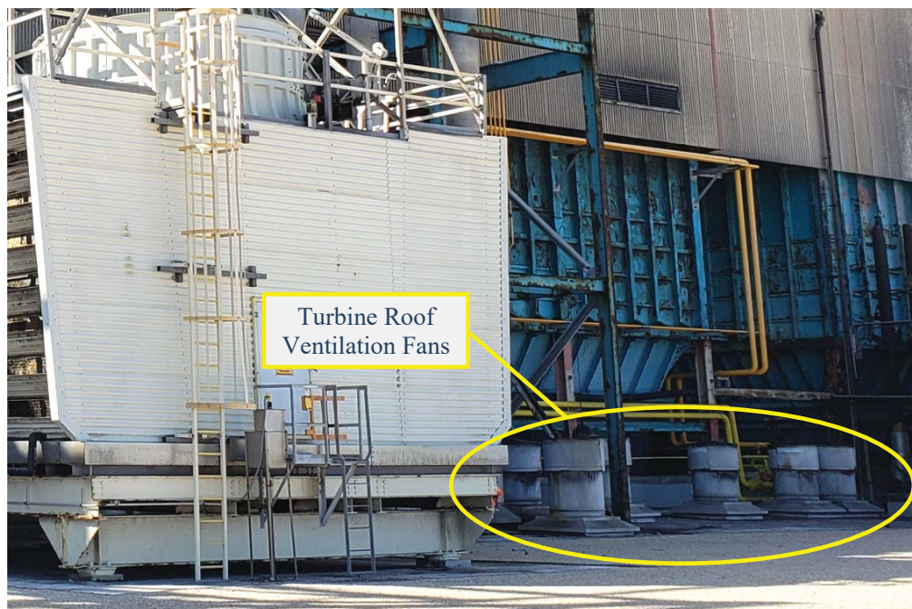
Figure 7 – Turbine Building Ventilation Fans
