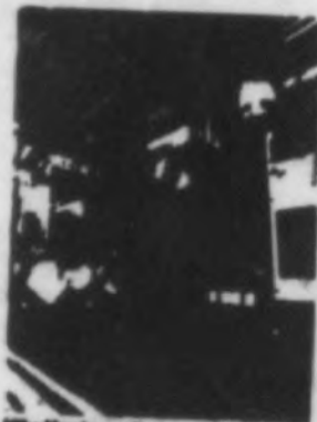
Blake Murphy, medical center air conditioning equipment dealer, and Peter Bloch, FPL account manager, examine the emergency generator which has allowed for load control savings.
