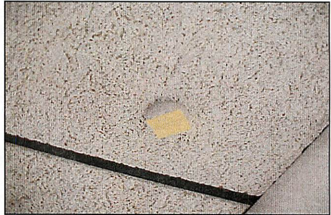
Figure 8. Ceiling mounted photosensor covered with post-it note by occupant making it inoperable.
