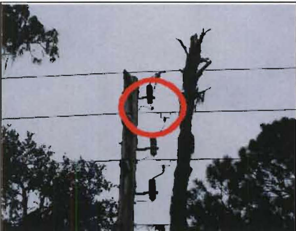
Sobriano No. 28: Failed lightning arrester on pole #723187.
