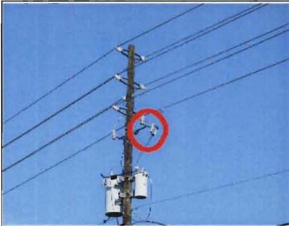
Sobrino No. 9: The pole is located just east of Lexington Avenue on US 92. Failed lightning arrester.
