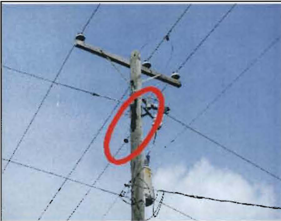
Sobrino No. 17: Failed lightning arrester on Dirksen Dr. and Fredricka Road.
