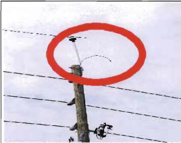
Sobriño No. 1: South side of US 192 just east of US 441 at Holopaw. Broken ground line on lightning arrester.
