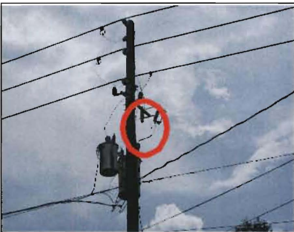
Sobrino No. 7: Pole is located across the street from 19 Main St., Windermere. Failed lightning arrester.
