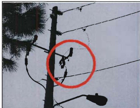
Sobriano No. 29: Failed lightning arrester on pole #129215 at the entrance to Lake Yale Landing.
