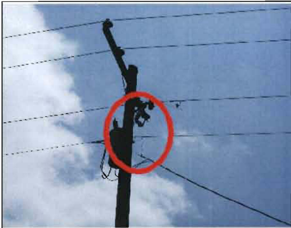
Sobrino No. 32: Failed lightning arrester approximately three miles from the entrance to Tarmac quarry on Hartwood Marsh Road.
