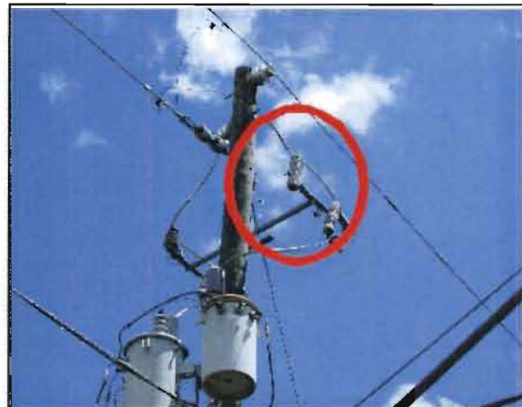
Velazquez No. 10: Pole at corner of Laurel Ave and Halibut Rd. Connection of failed lightning arrester can be seen between the arrester and the fuse holder on the right-hand side of the pole.
