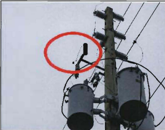
Velazquez No. 17 Pole 132108-047324 at Lily Ave East and 9th St North. Lightning arrester of leftmost transformer failed. Connector is dangling to left of fuse holder.
