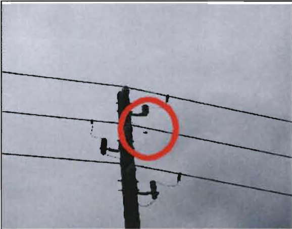
Sobrino No. 30: Failed lightning arrester at the pole on CR 561 near Leatrice Drive and at the entrance to Sugar Ridge Estates.
