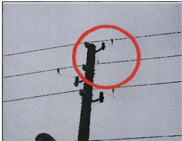
Velazquez No. 16: Pole 6-75351 in front of 2604 4th St South. Top phase lightning arrester failed. Connector dangling on right side of pole beneath arrester.
