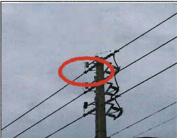
Sobriño No. 24: Failed lightning arrester just north of previous photographed pole along US 19 in Eustis.
