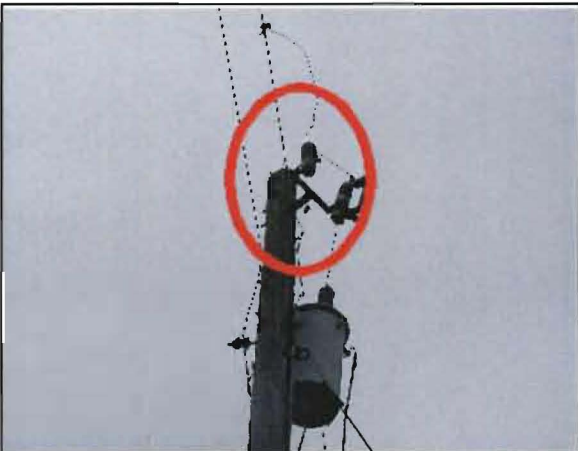
Velazquez No. 19: Pole 132477-044360 on Ridgewood Ave, first pole east of 6th St. Lightning arrester failed. Connector can be seen directly below arrester.
