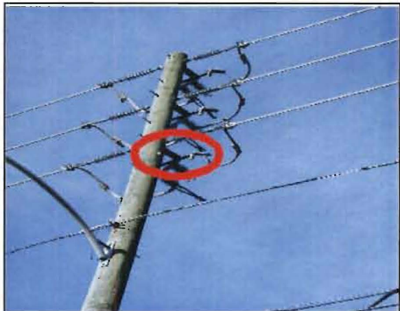
Sobrino No. 12: The pole is located at the northeast corner of Amelia Ave. and New York Ave., De Land. Failed lightning arrester.
