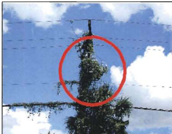
Velazquez No. 4: Approximately 1/10 of a mile south of pole 6357034 on Scenic Hwy (Alt 27). Vines have engulfed a capacitor bank.
