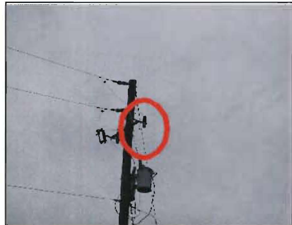
Sobrino No. 33: Failed lightning arrester along Hartwood Marsh Road approximately 1/4 mile south of the entrance to the Tarmac quarry.
