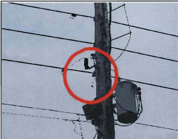
Sobriño No. 22: Pole # 131190, serving 18515 US 441, north of Mount Dora. Failed lightning arrester.
