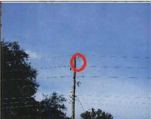
Sobrino No. 11: The pole is on US 17 south of De Leon Springs. Failed lightning arrester.
