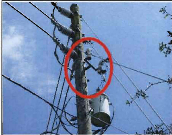
Sobrino No. 33: Failed lightning arrester on E. Bay Street one pole west of Ninth Street.
