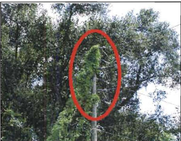
Velazquez No. 3: Across from pole 6357034 on Scenic Hwy (Alt 27) between Egg Farm Rd and Mountain Lake Cutoff Rd. Vines are encroaching on primary lines here and at various locations along this stretch of highway.
