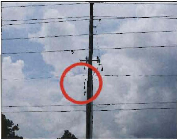
Sobrino No. 5: Pole is located by the Bay Meadows Elementary School on CR 435. Failed lightning arrester.
