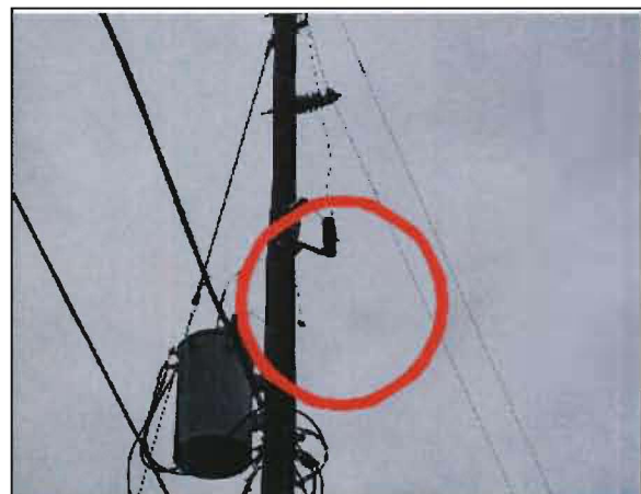
Sobriño No. 25: Pole #130168, located on Key Ave. and a half block east of S. Grove St. (US 19). Failed lightning arrester.
