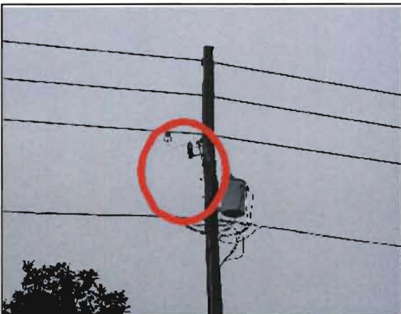
Velazquez No. 15: Pole next to 1915 10th St. Lightning arrester failed. The connector is dangling on left of pole beneath fuse holder.
