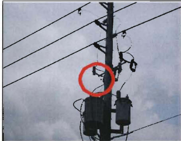
Sobrino No. 18: Failed lightning arrester at Semoran and Wilshire Blvd.
