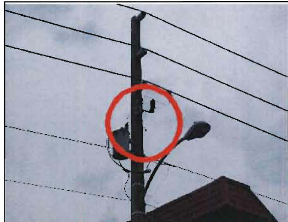
Sobriño No. 23: Failed lightning arrester in front of Eustis Square, on US 19, in Eustis, Florida.
