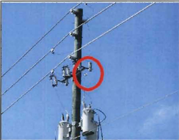
Sobrino No. 13: Pole #142597 located on Enterprise Road, 5 poles north of Saxon Road. Failed lightning arrester.
