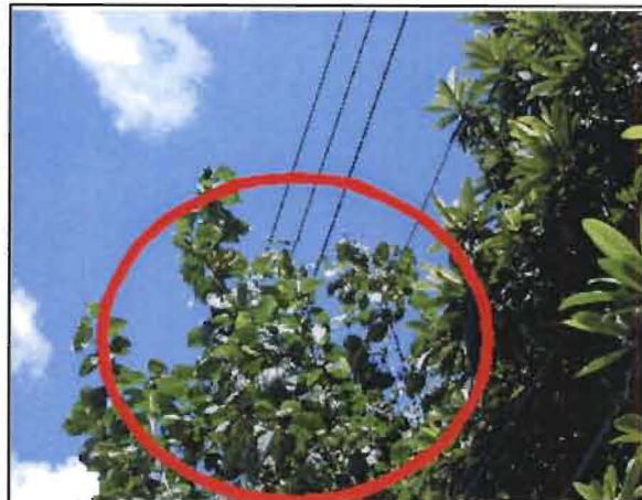
Velazquez No. 2: Adjacent to pole 133647-039450 on Frontage Rd between Towerview Dr and 7th St. Tree limbs at several locations in this general vicinity are contacting the power line.
