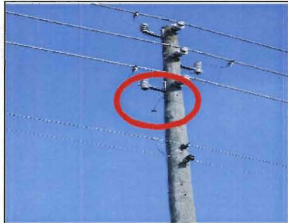
Sobrino No. 14: Failed lightning arrester on pole serving 1440 Normandy Blvd., Deltona.
