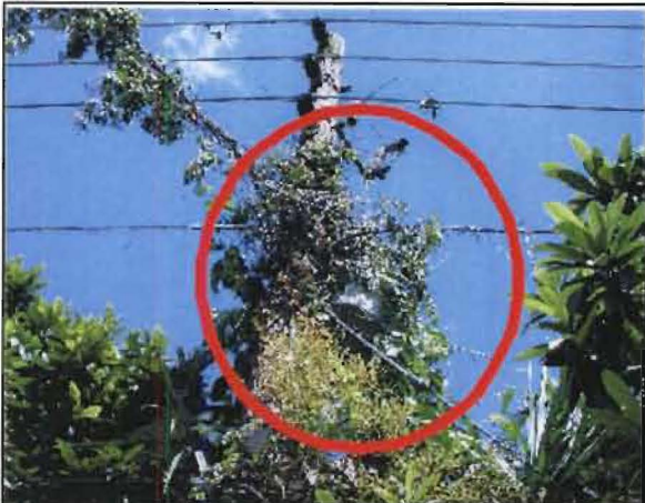
Velazquez No. 1: Pole 133647-039450 on Frontage Rd between Towerview Dr and 7th St. Vines have engulfed a transformer.
