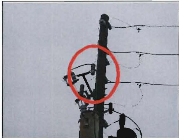
Velazquez No. 20: Pole 6-77498 on Lake Mabel Loop Rd just east of Lake Trask Rd. Lightning arrester failed. Connector can be seen next to fuse holder.
