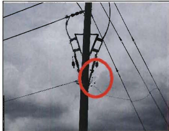
Sobriño No. 4: Pole #136344, ½ mile north of previous location on SR 535. Failed lightning arrester.
