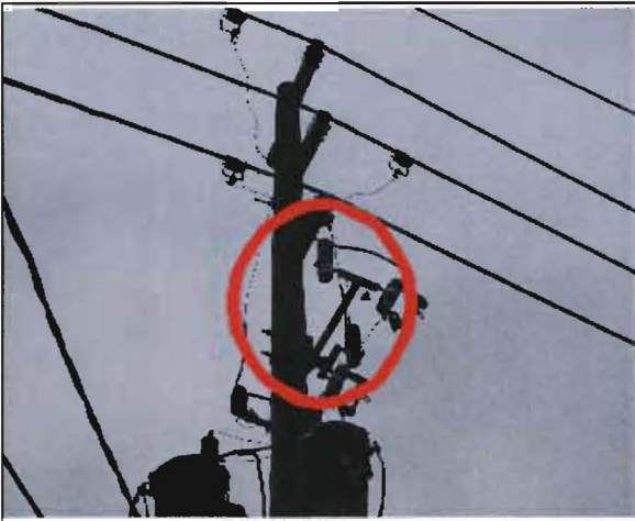
Sobriano No. 26: Failed lightning arrester one block north of the previous photograph (See No. 25). The pole is located on the corner of Ward Ave. and S. Grove St.
