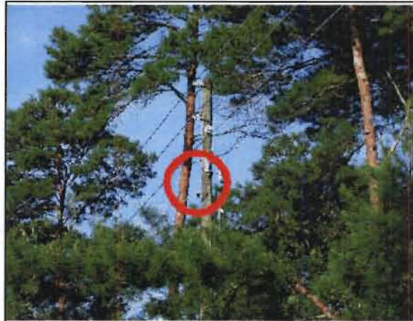
Sobrino No. 10: The pole at the intersection of CR 15A and Trail-in-the-Pines Ave. Failed lightning arrester.
