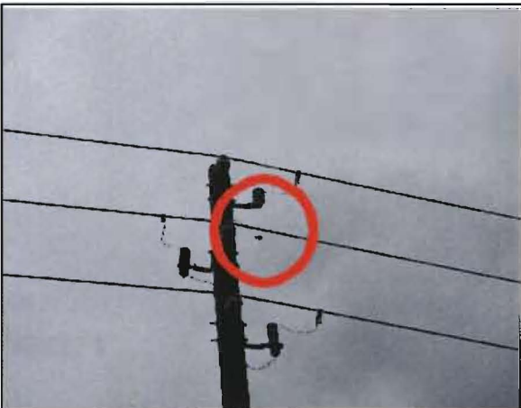
Sobrino No. 32: Failed lightning arrester along SR 50 between Clermont and Groveland at the entrance to Green Valley Country Club.
