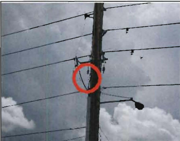
Sobriño No. 3: Pole #136404/056017, on SR 535, ½ mile north of US 192 on parking lot of Lake Buena Vista Factory Outlet. Failed lightning arrester.
