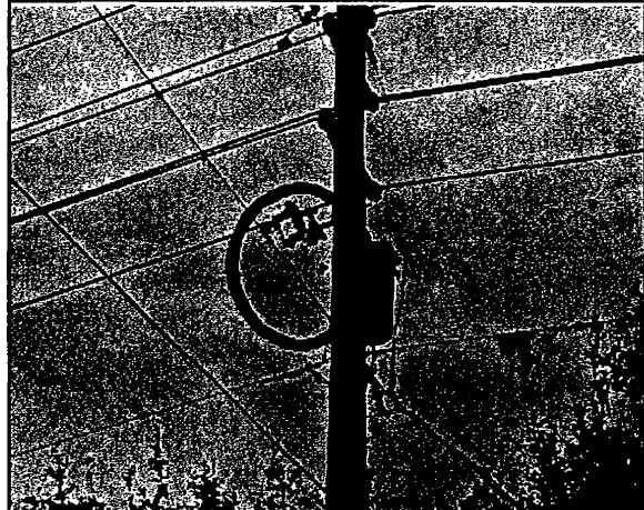
Sobrino No. 6: Pole is located at the intersection of Magnolia St. and 6th Ave., north on CR 435 and west on CR 439 towards Windermere. Failed lightning arrester.
