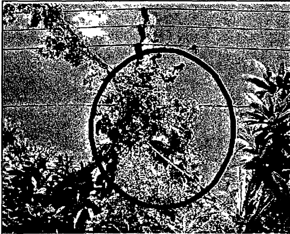
Velazquez No. 1: Pole 133647-039450 on Frontage Rd between Towerview Dr and 7th St. Vines have engulfed a transformer.
