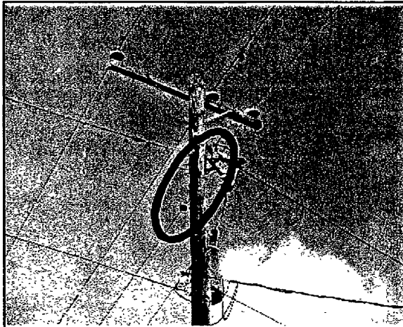
SobriNo No. 17: Failed lightning arrester on Dirksen Dr. and Fredricka Road.
