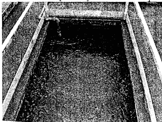
Aeration Tank [ 1 of 3 ] : Thin Mixed Liquor
