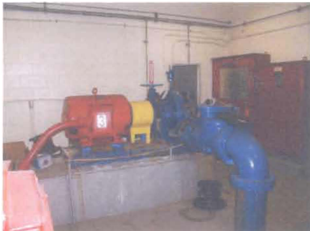
Dedicated Fire Pump and Controls
