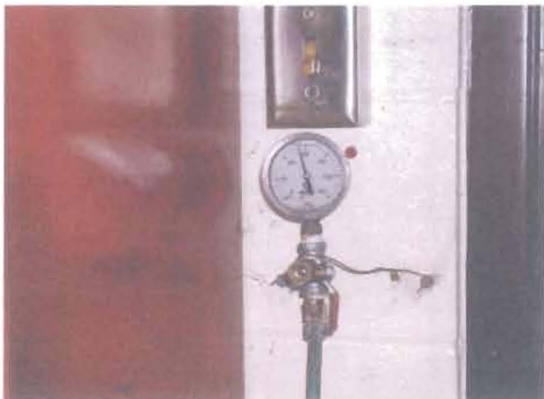
Fire System pressure at pump building 137 PSI
