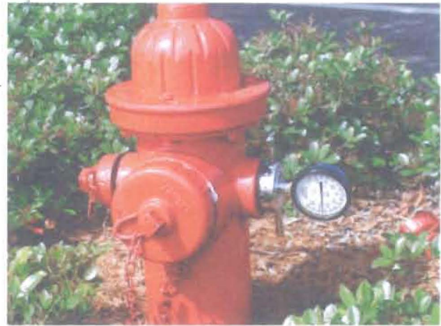
On-site Fire System Pressure Reading 135 PSI Hydrant was flushed prior to reading.
