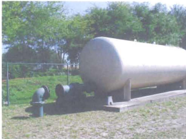
Potable system severed
