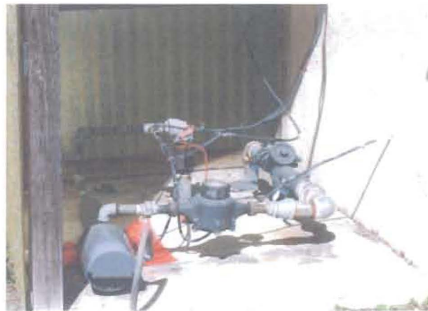
Fire System Jockey Pump
