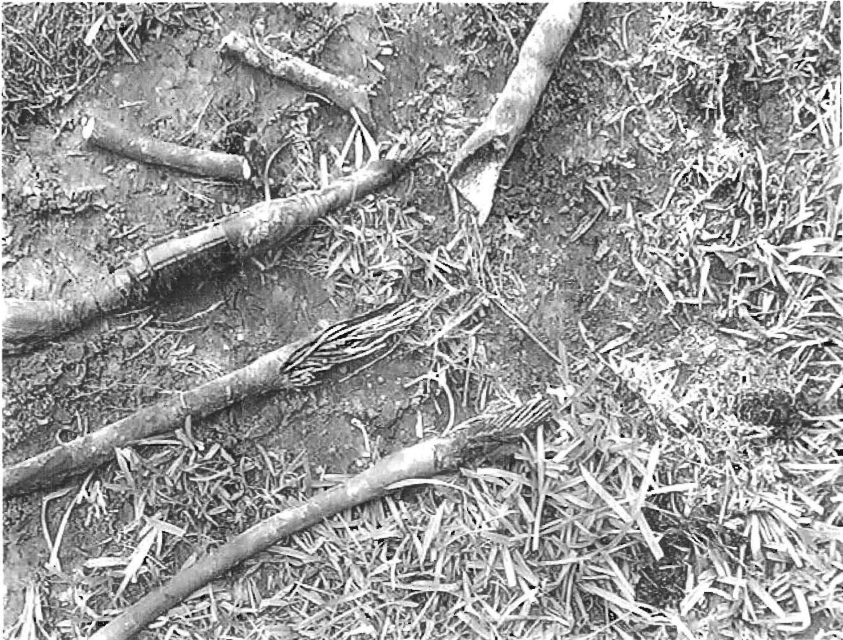
8.27.09 Front of Bldg. 6 – 3 splices from repair made by Progress Energy in 2006.
