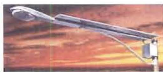
Figure 4-1 Solar Powered Streetlight
