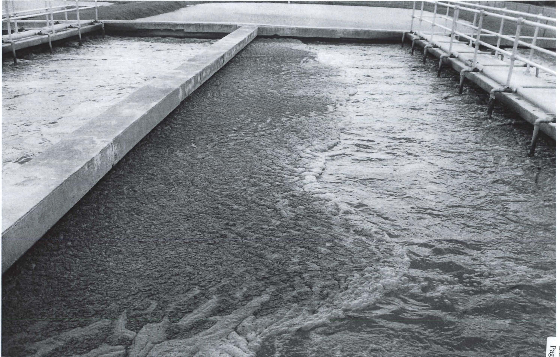
Photo above of the MLSS in the aeration tanks
