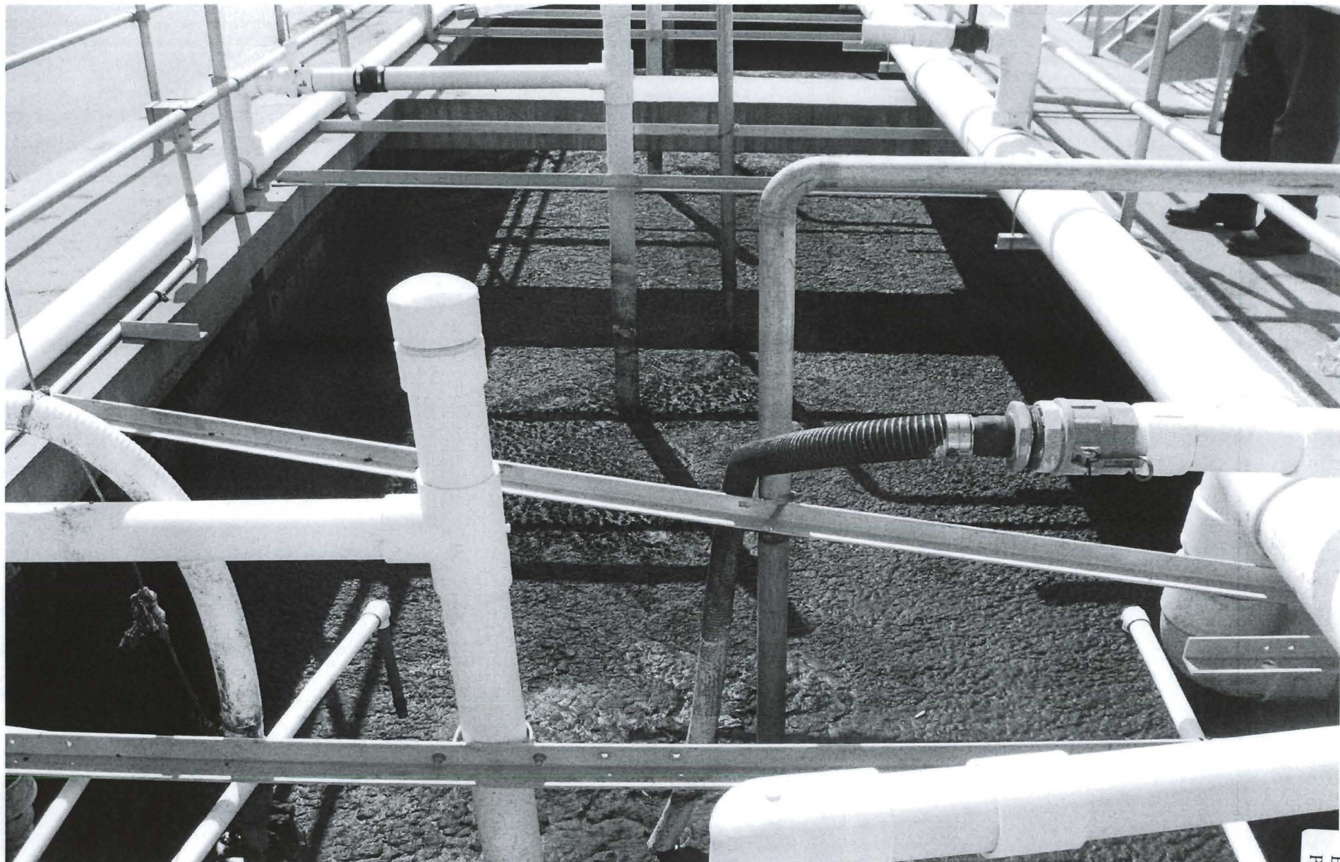
Photo of the biosolids in the sludge holding tank.
