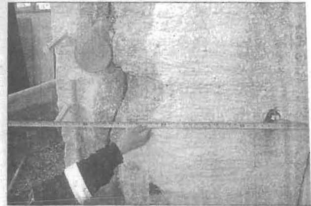
After Progress cut a hole in the containment building to install new generators, the walls separated.
