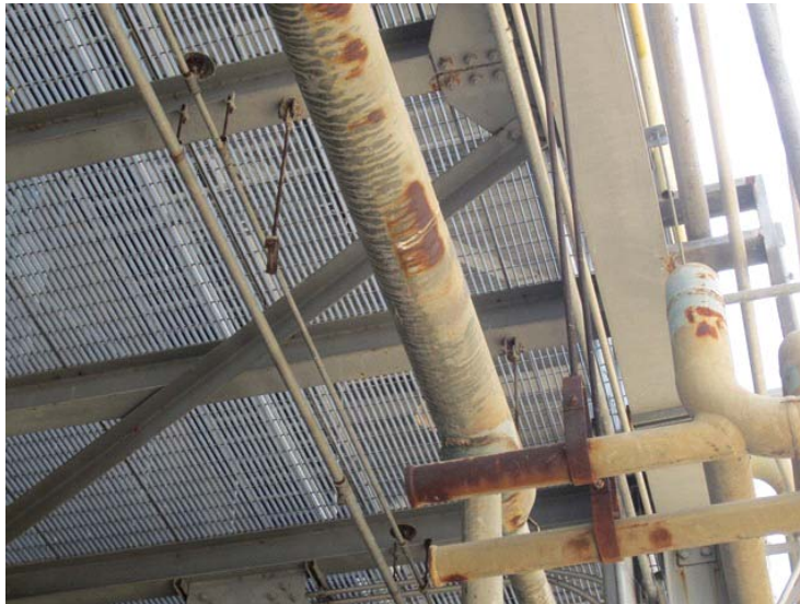
Corrosion on piping
