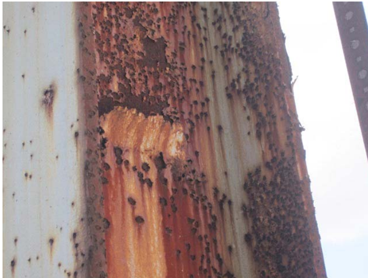
Severe corrosion on structure
