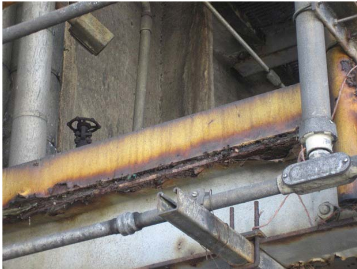
Heavy corrosion occurring
