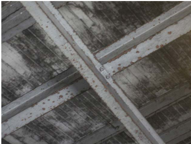
View of corrosion on structure
