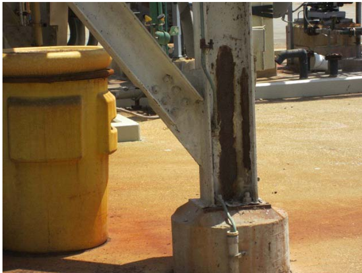
Corrosion on structure
