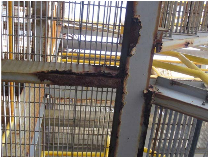
View of corrosion on structure
