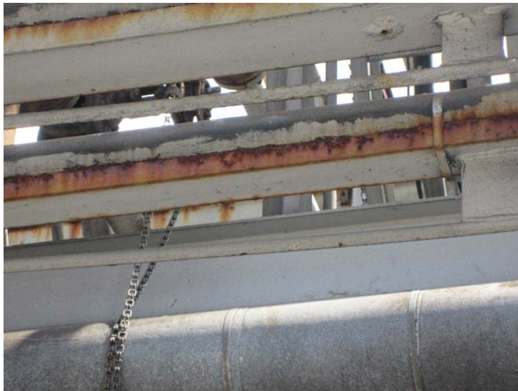
Corrosion on structure
