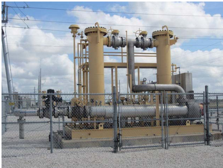
View of pump station
