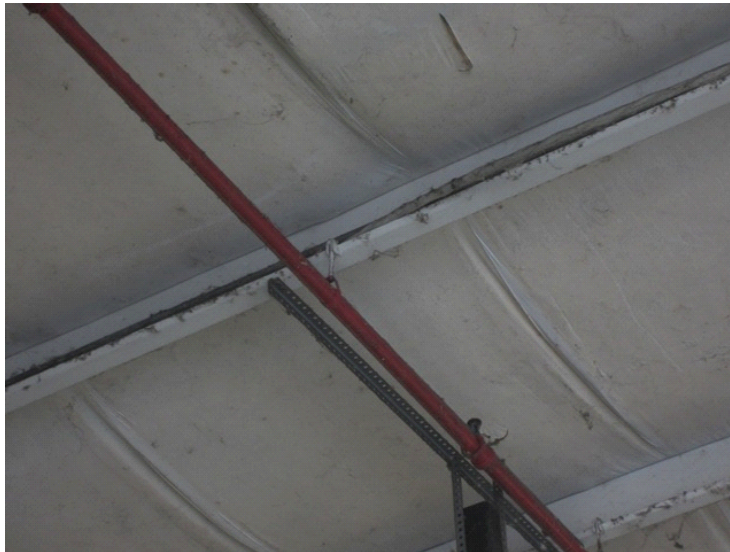
Slight corrosion inside warehouse
