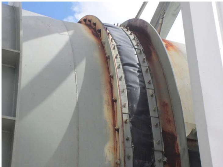
Corrosion at joints
