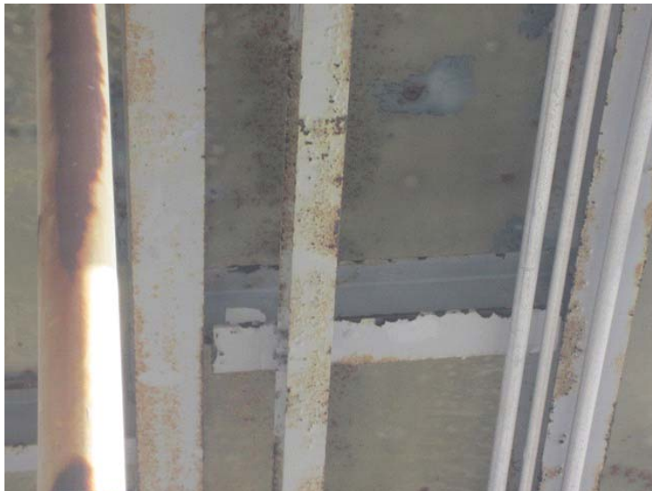
Corrosion on structure
