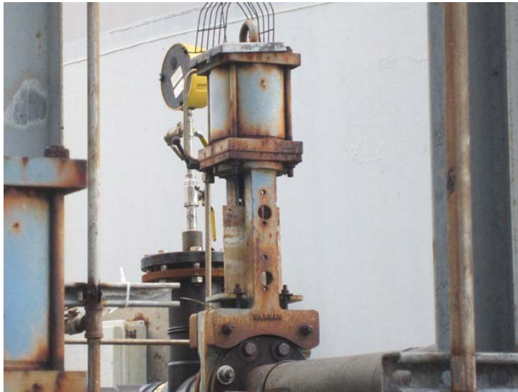
Corrosion on equipment
