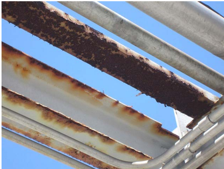
Heavy corrosion on piping and structure
