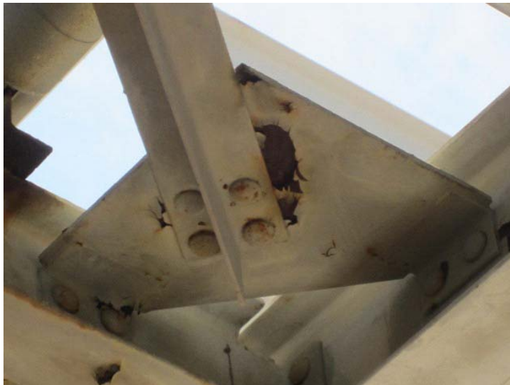
Corrosion on structure
