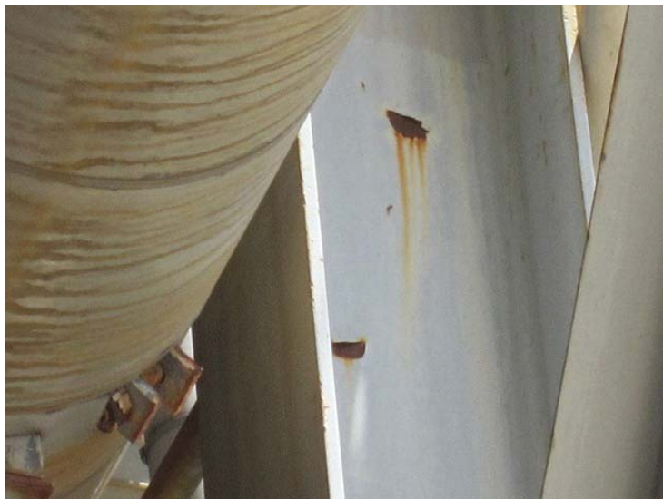
Corrosion on structure
