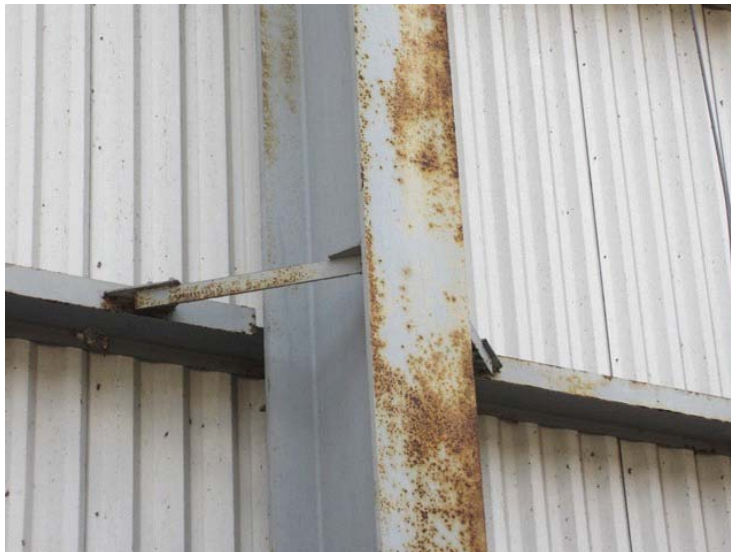
Corrosion on structural steel
