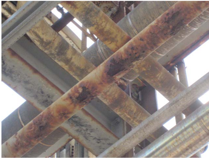
Corrosion on piping
