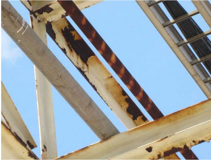
Corrosion in section
