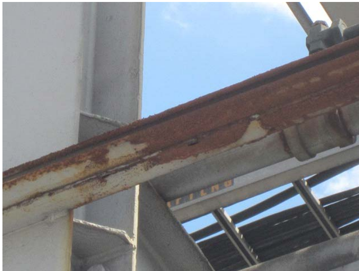
Corrosion on structure
