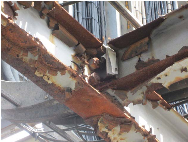
Undercutting rust on structure
