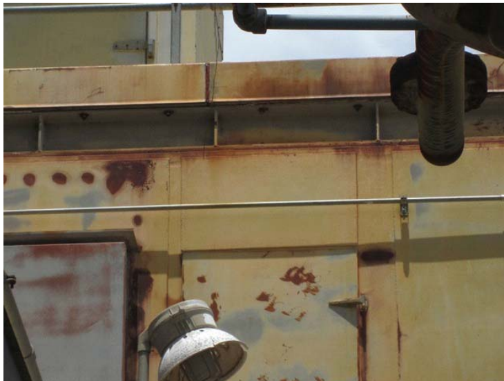
View of corrosion on building
