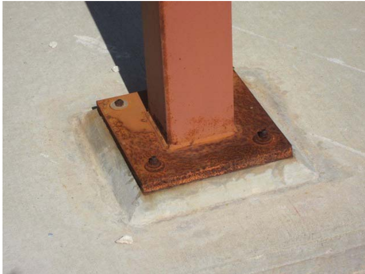
Corrosion on supports
