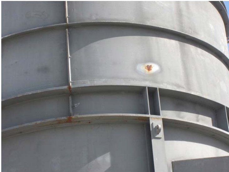
Corrosion on stack
