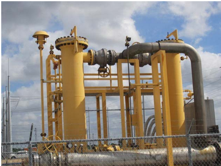
View of pump station
