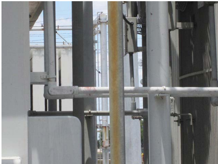
Minor corrosion on structure
