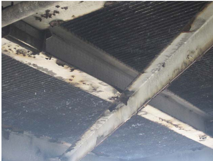
Close up view of corrosion
