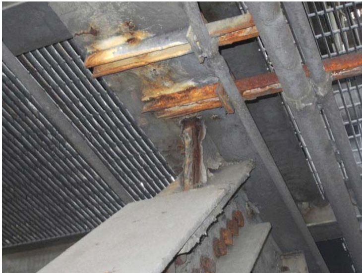
View of corrosion on structure
