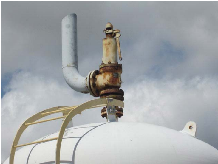
Corrosion on vent
