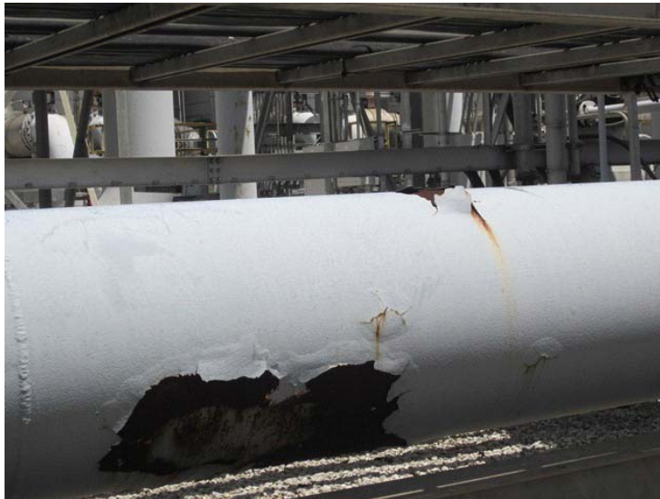
Undercutting on piping
