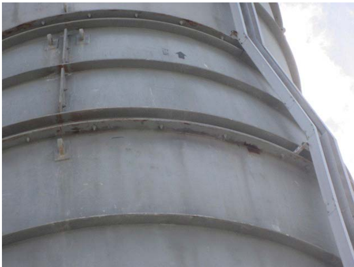
Edge corrosion on stack
