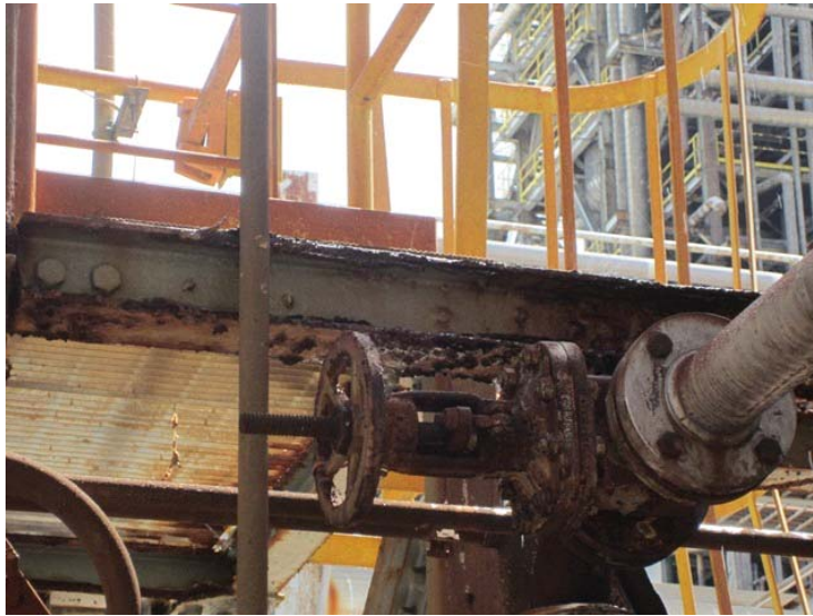
View of corrosion on structure
