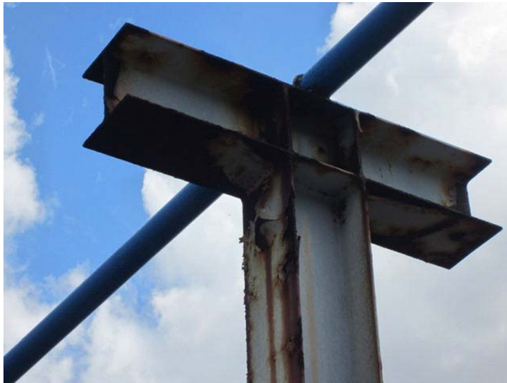
Corrosion on structure
