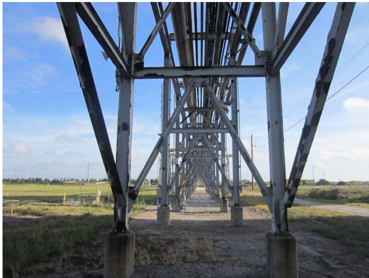
General view of piperack
