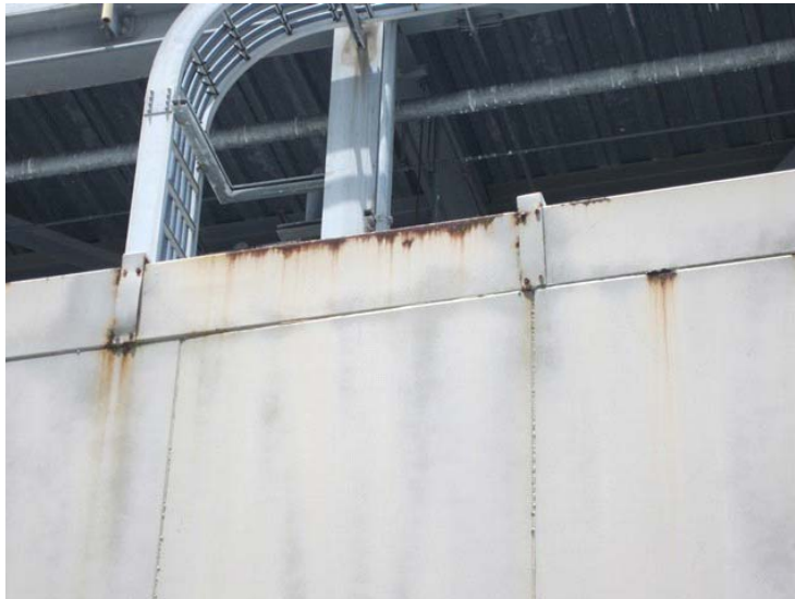
Edge corrosion on building structure
