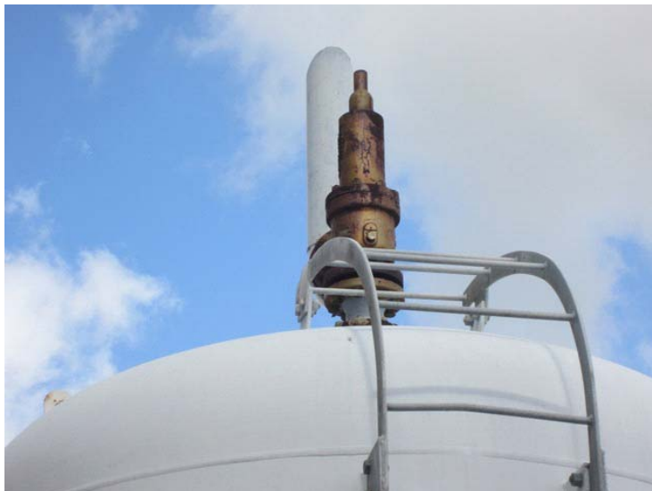
Corrosion on top of tank
