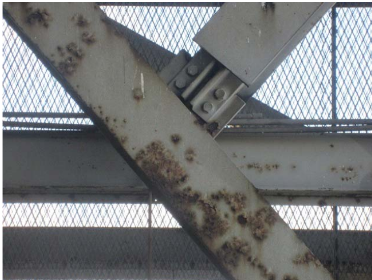
Corrosion on structure
