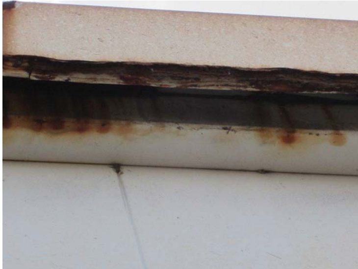
Severe corrosion on building structure
