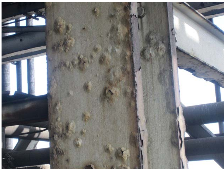
Rust nodules cover structure
