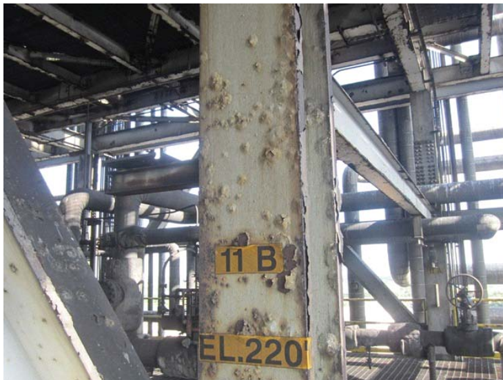
Rust nodules on structural steel
