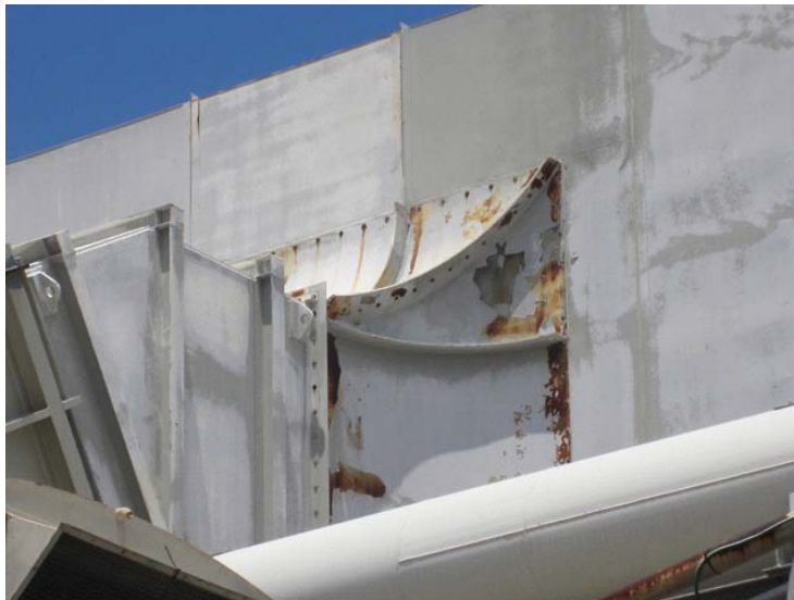
View of corrosion occurring
