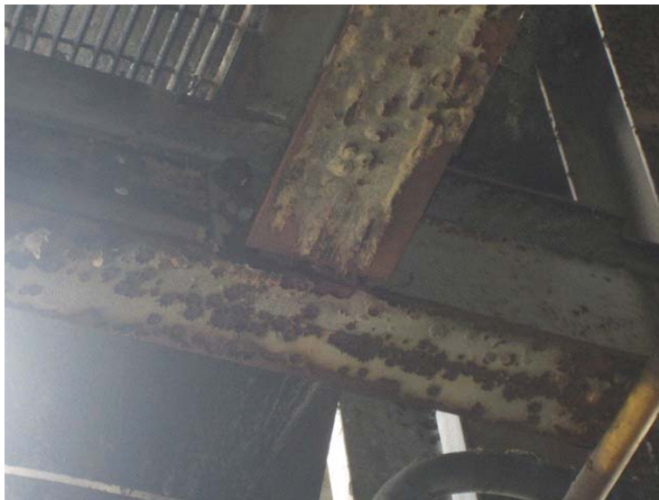
Heavy corrosion on structural steel
