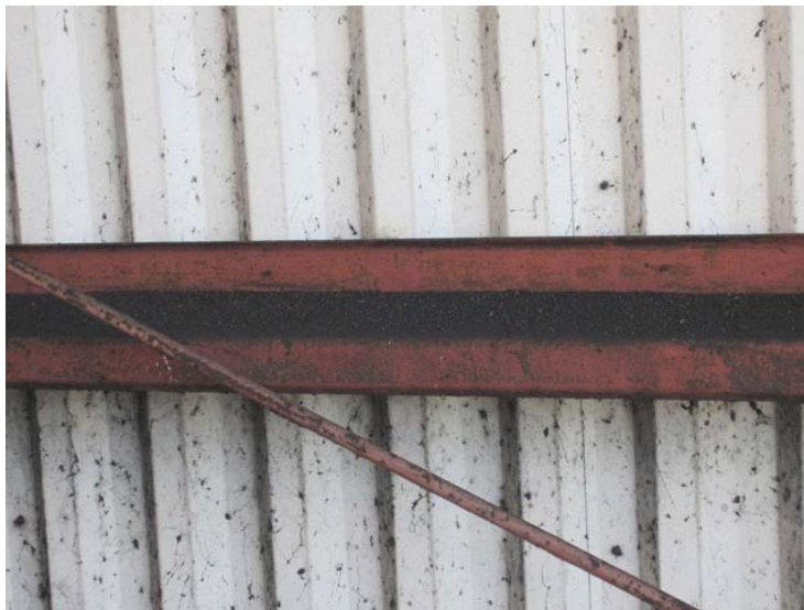
View of corrosion on structure
