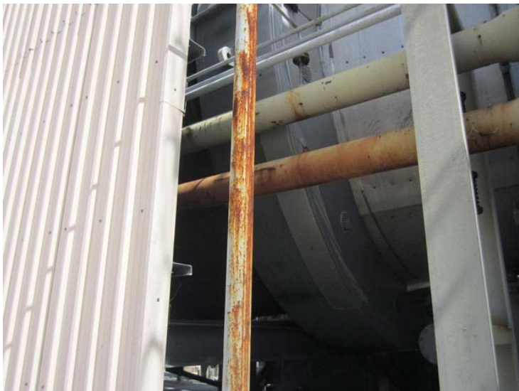
Corrosion on piping
