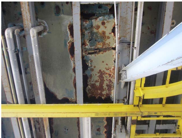
View of heavy corrosion
