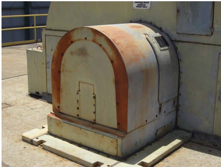
Corrosion on equipment
