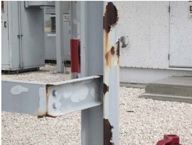
Heavy corrosion on structural steel
