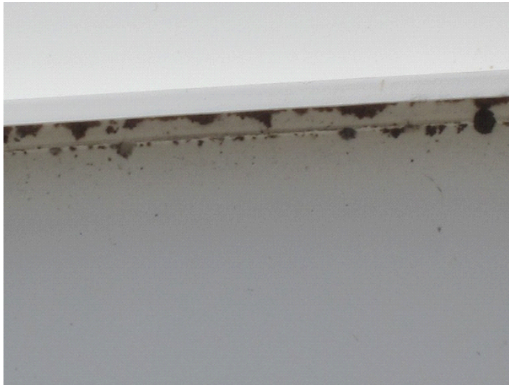
Minor coating wear
