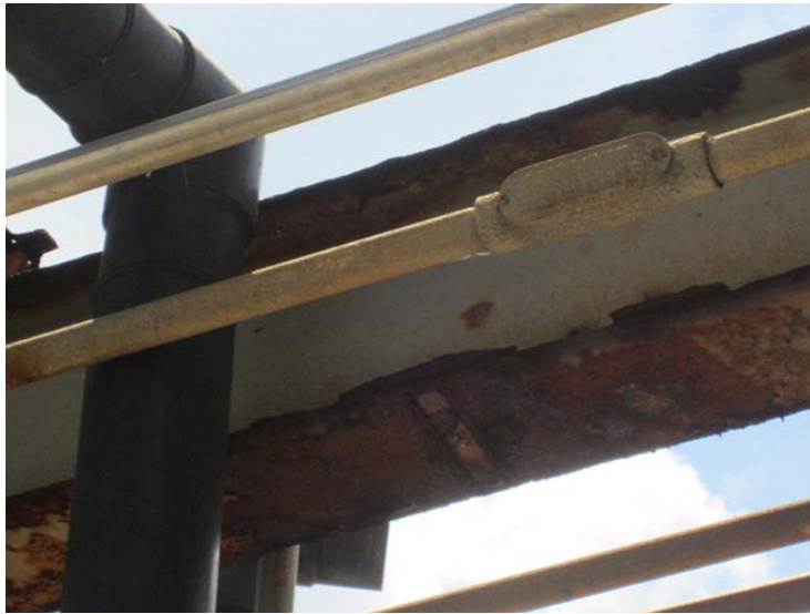
View of Corrosion
