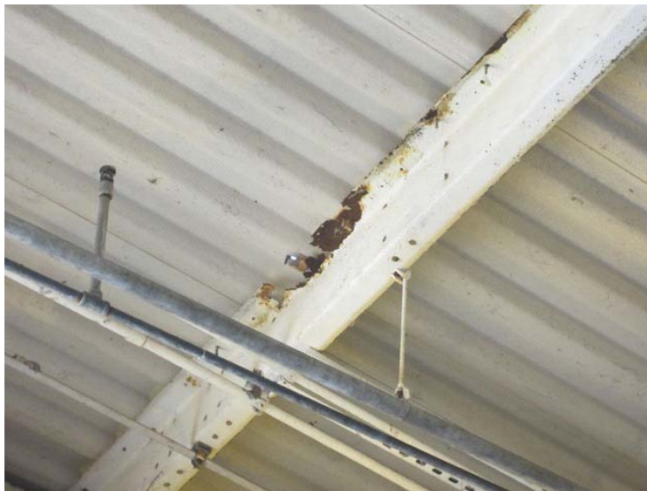
Corrosion on structure
