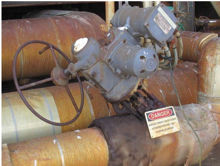
View of corrosion on valves
