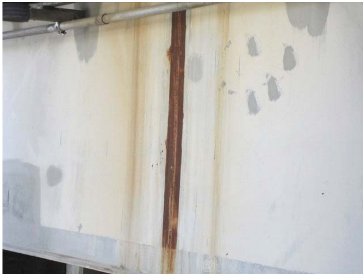
Coating wear and corrosion occurring
