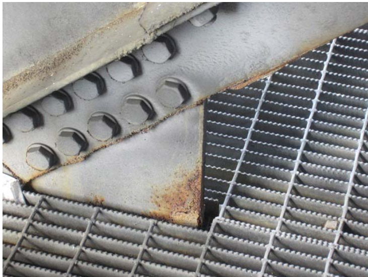
Corrosion on structural steel
