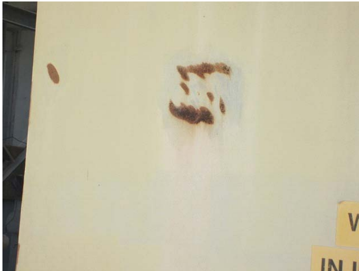
Minor corrosion on building structure
