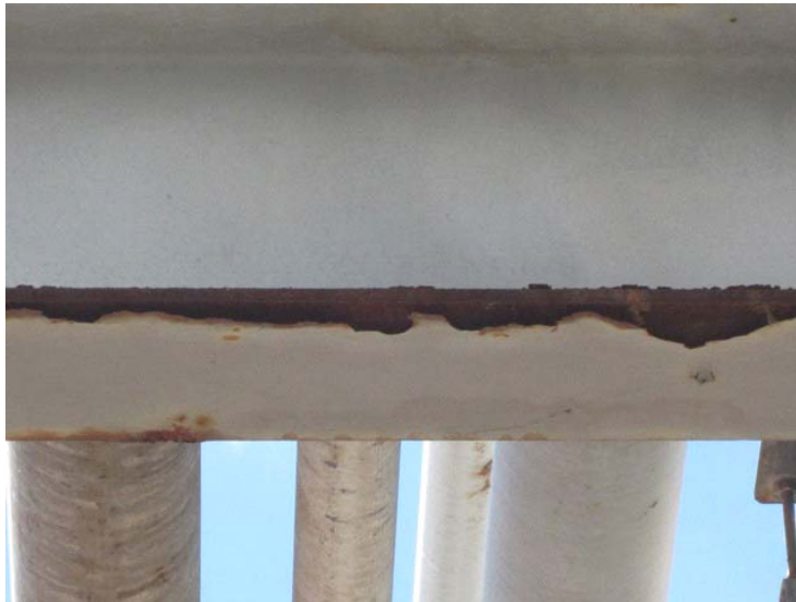
Corrosion on structure
