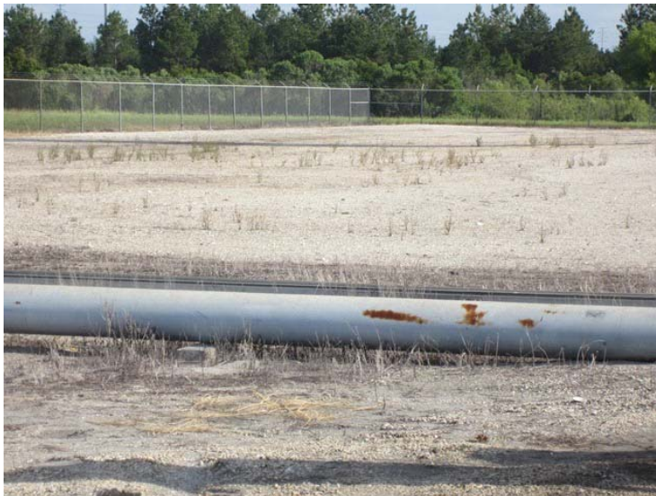
Corrosion on pipe
