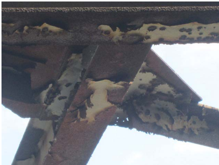
Heavy corrosion on structure
