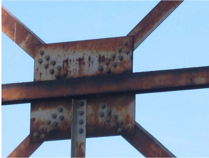
View of corrosion
