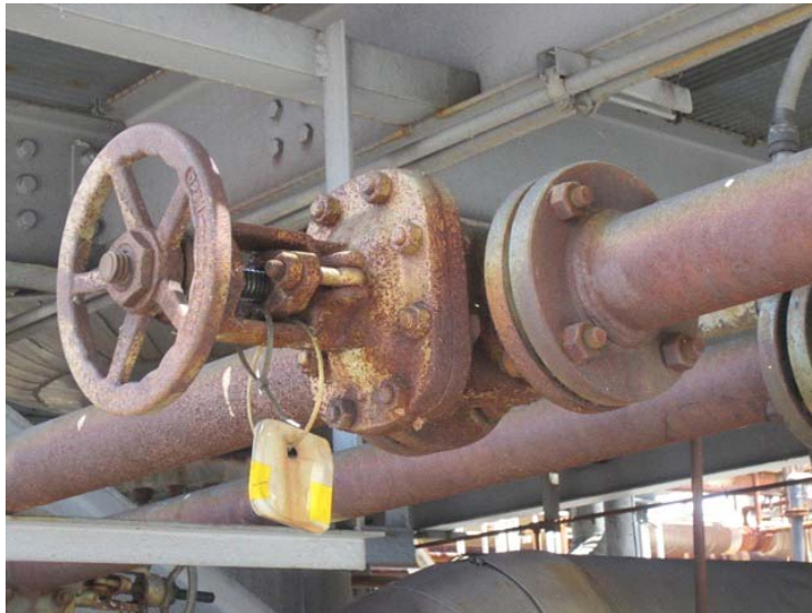
Corrosion on piping
