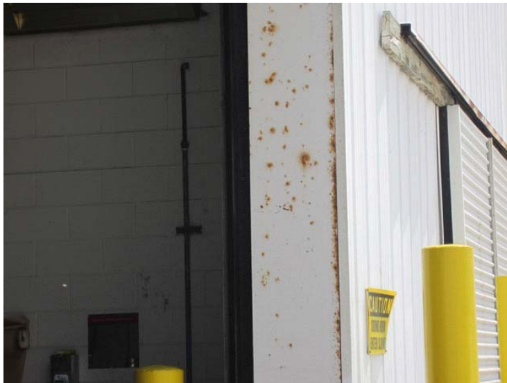
Minor corrosion on warehouse structural steel
