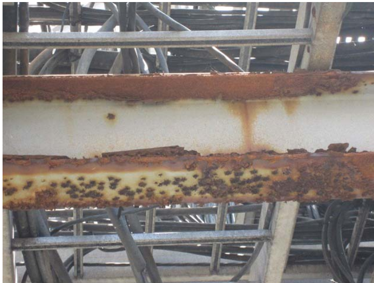
Corrosion on structural steel
