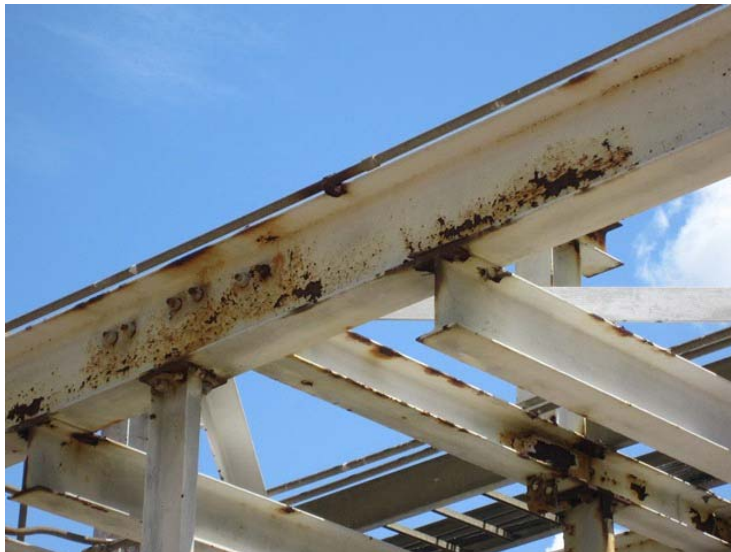
Corrosion on structural steel
