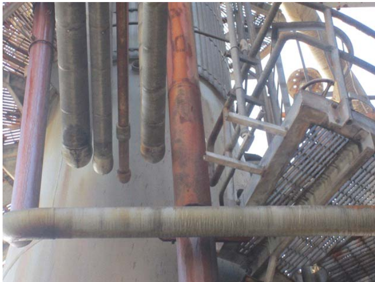
Corrosion on piping
