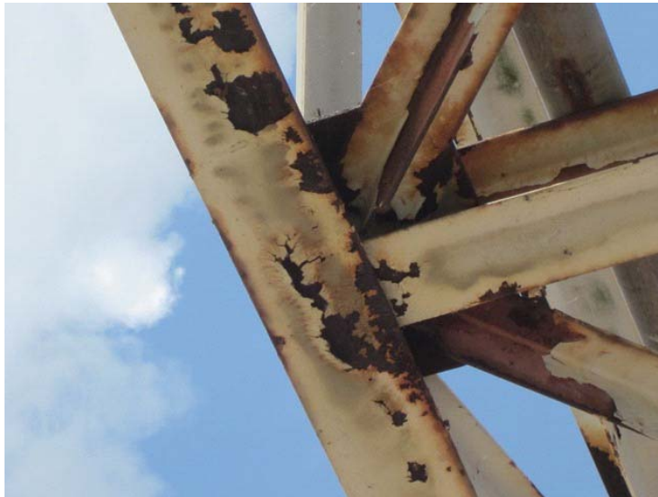
View of undercutting rust
