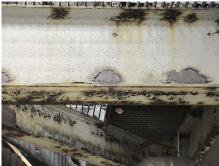
Heavy corrosion on structure
