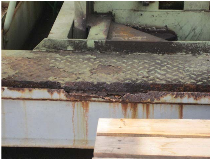
Metal loss on structure
