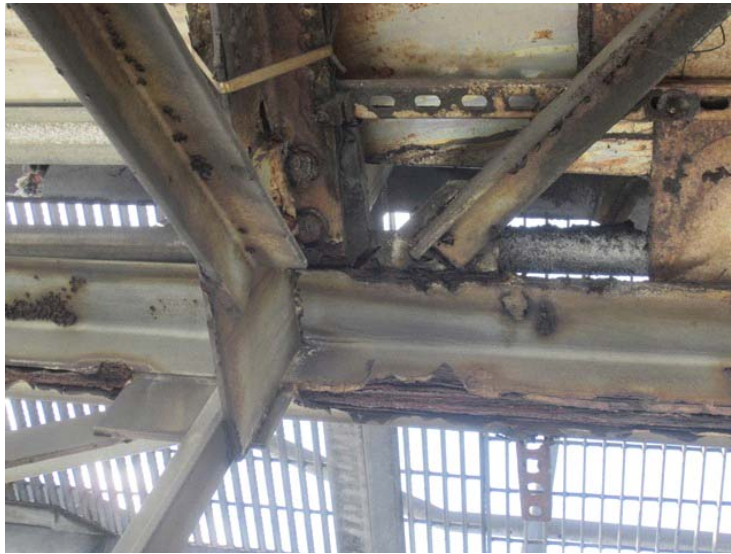
Corrosion on structure
