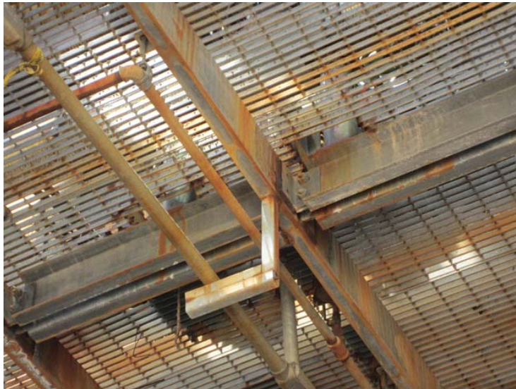
Corrosion on structure in section
