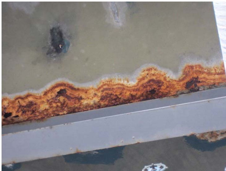
Severe corrosion on structural steel
