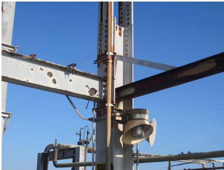
View of corrosion on support structure
