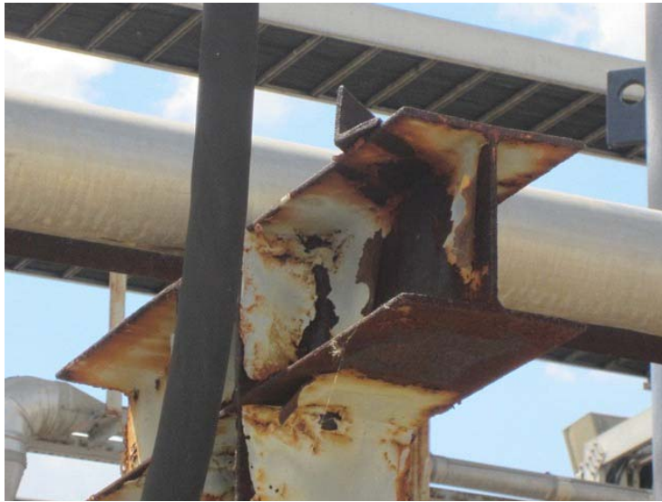
Corrosion on structure
