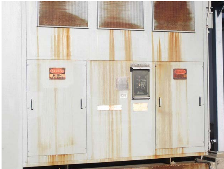
View of surface rust
