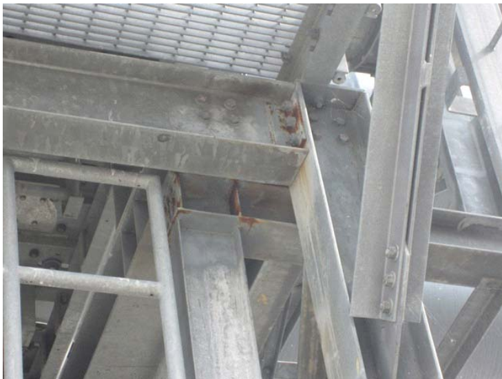
Minor corrosion on structure
