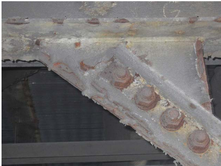
Corrosion on structure
