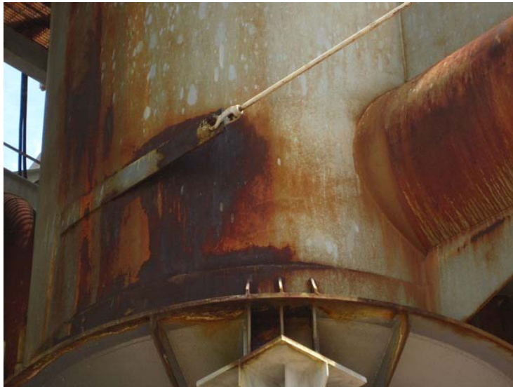
Close up view of corrosion
