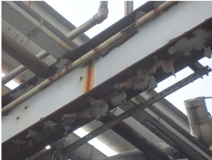
Heavy corrosion on structural steel
