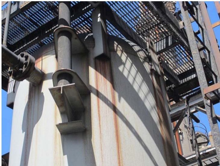
Corrosion on tower structure
