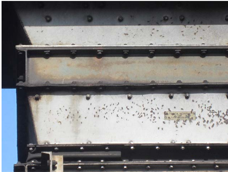
Corrosion on equipment
