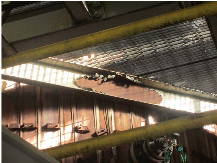
Corrosion in section
