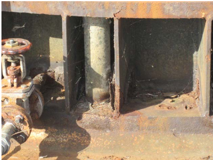
Corrosion on stack
