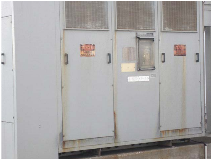
View of corrosion
