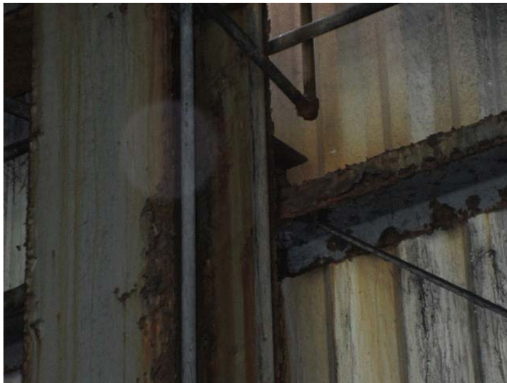
Corrosion on structure
