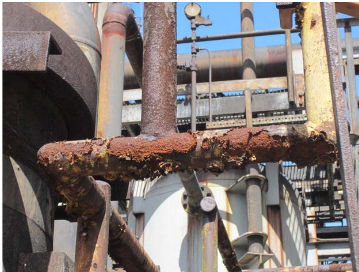
Heavy corrosion on piping
