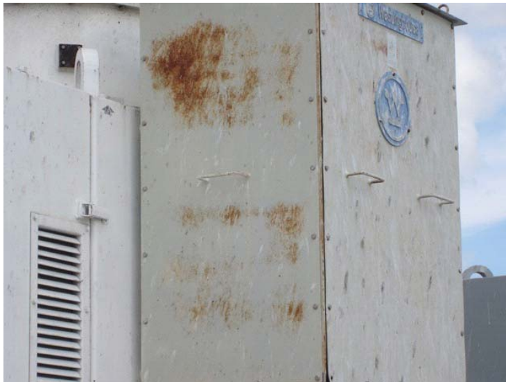
Minor surface corrosion
