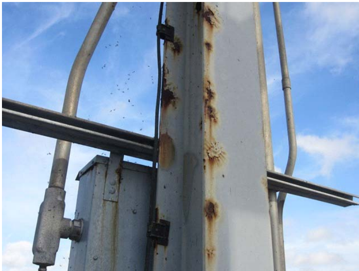
Corrosion on structure
