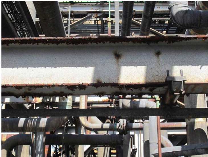
Corrosion on structure
