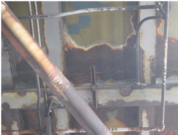
General view of corrosion in section
