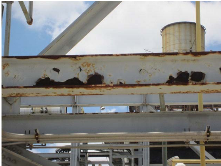
Corrosion on structure
