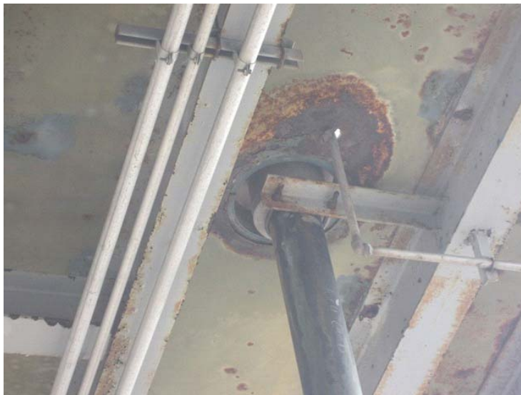
Severe corrosion occurring
