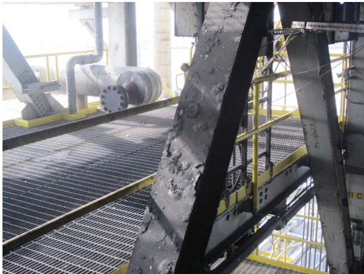
Rust nodules on structure
