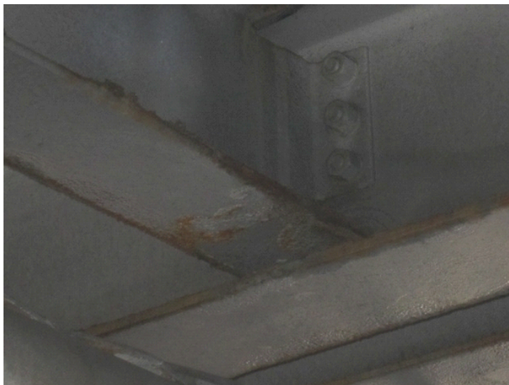
Corrosion on structure
