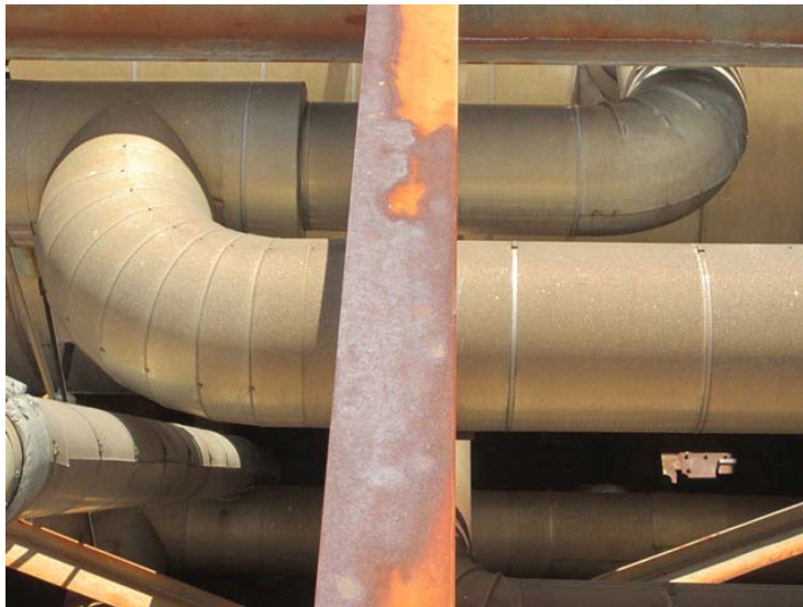
Corrosion on structure in section
