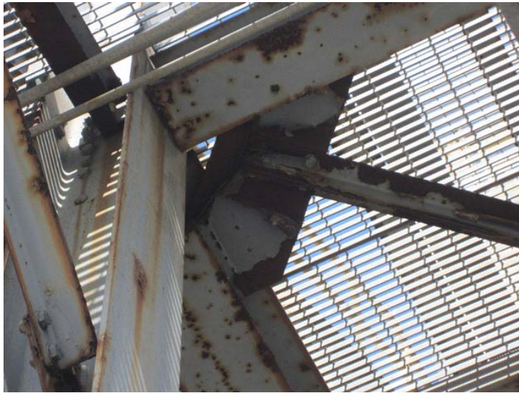
Corrosion on structure
