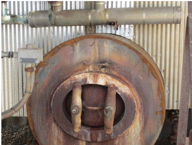
Corrosion on equipment
