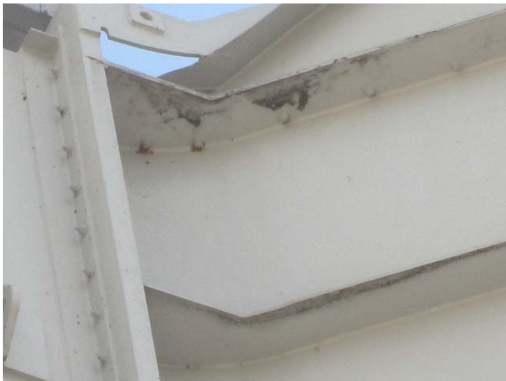
Minor corrosion in section
