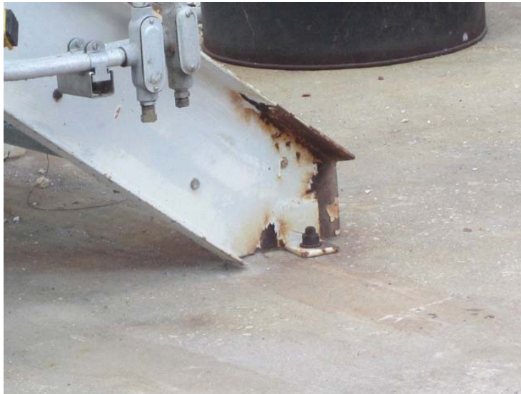
View of corrosion
