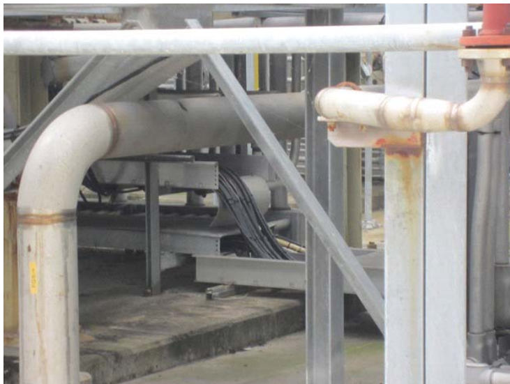
Slight corrosion in section
