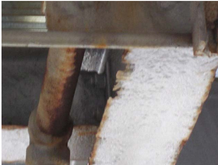
Corrosion on structure
