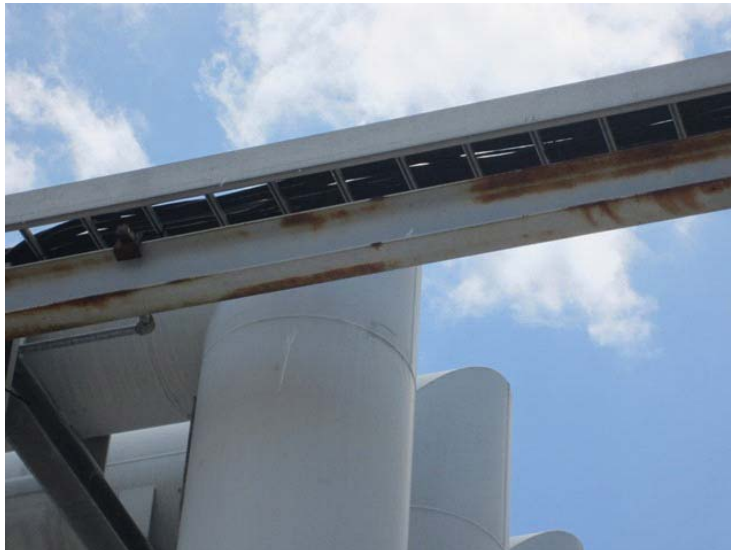
Corrosion on rack structure
