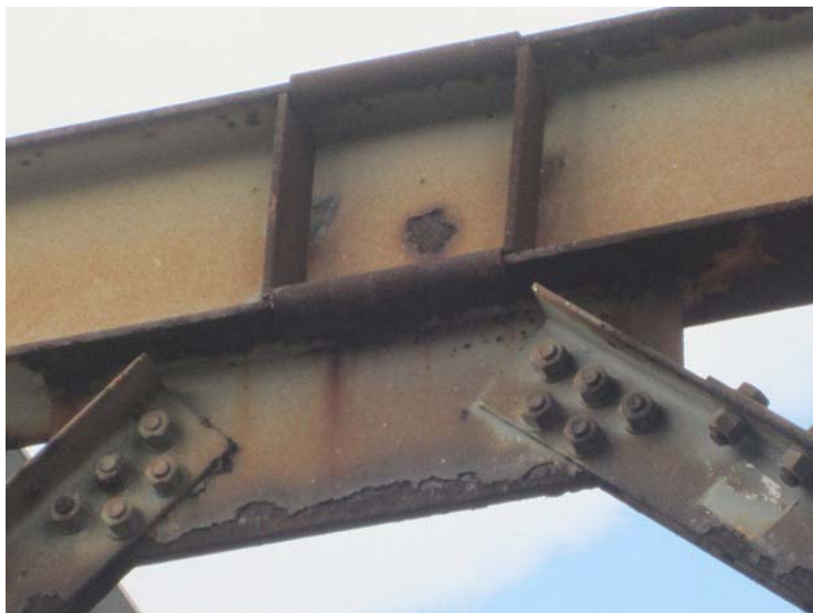
Corrosion on structural steel
