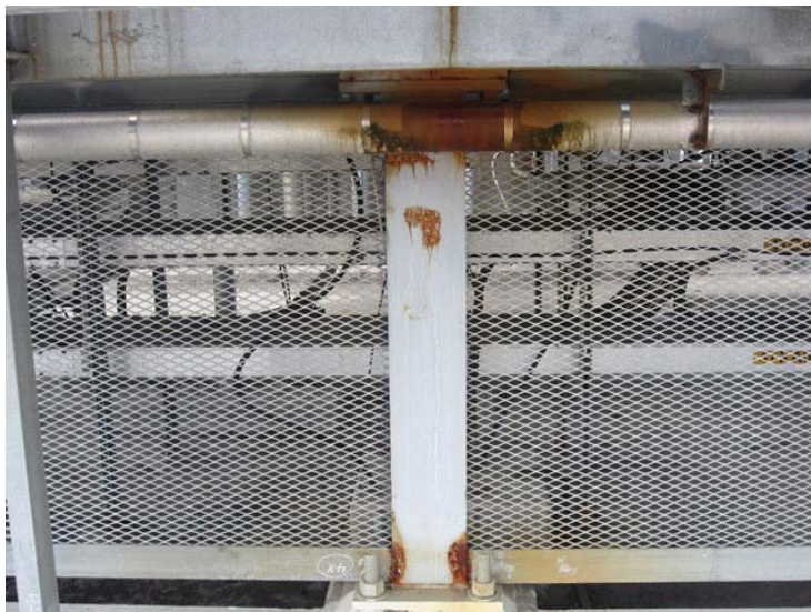
Corrosion on structure
