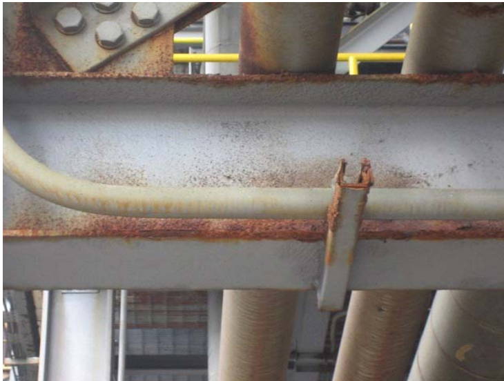
Pin hole and edge corrosion occurring
