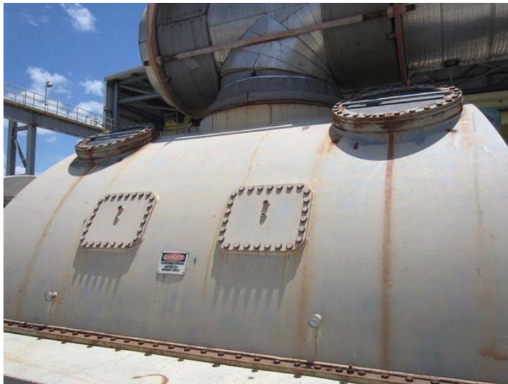
Corrosion on turbine structure
