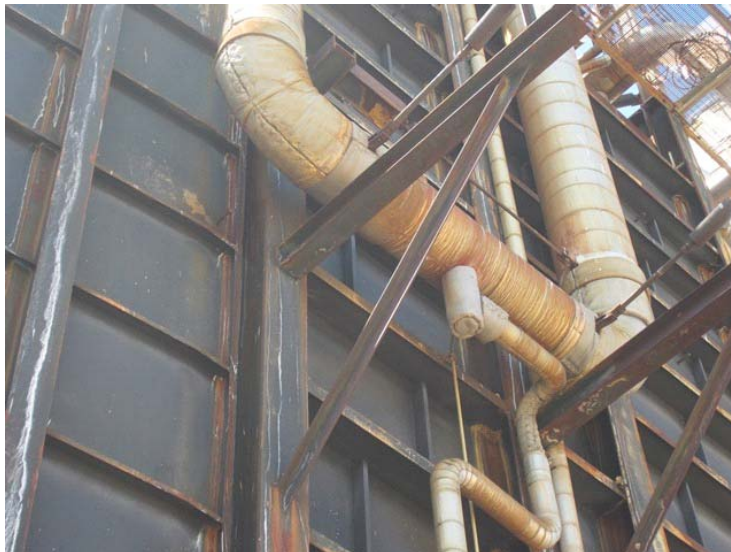
View of corrosion on pipe supports
