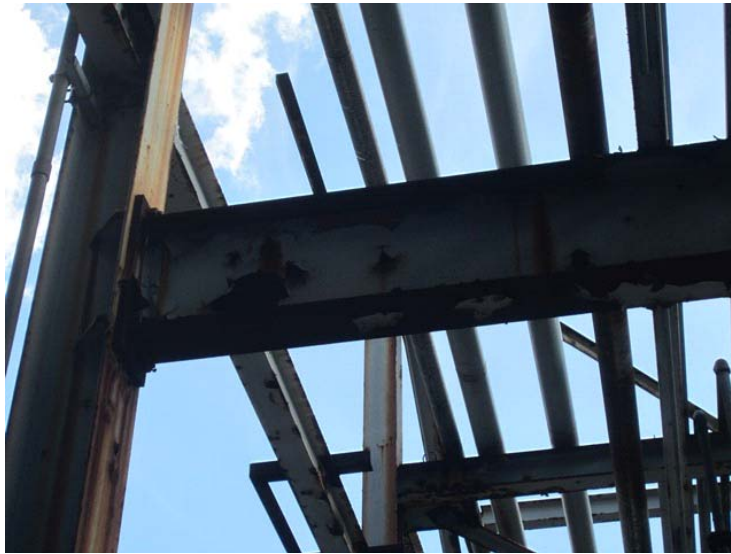
Corrosion in piperack
