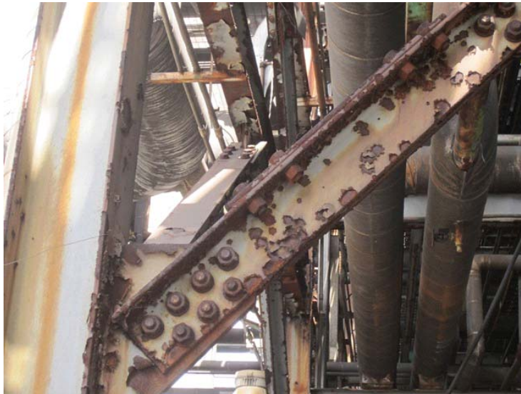
Corrosion on support structure
