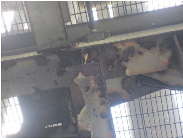
Heavy corrosion on structure
