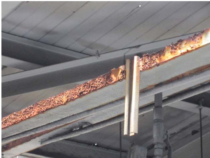
Corrosion on structure
