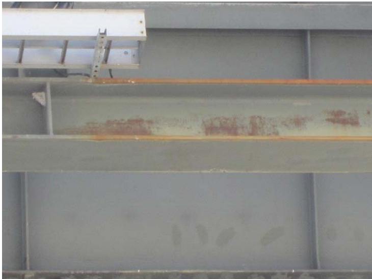
Corrosion on stack structure
