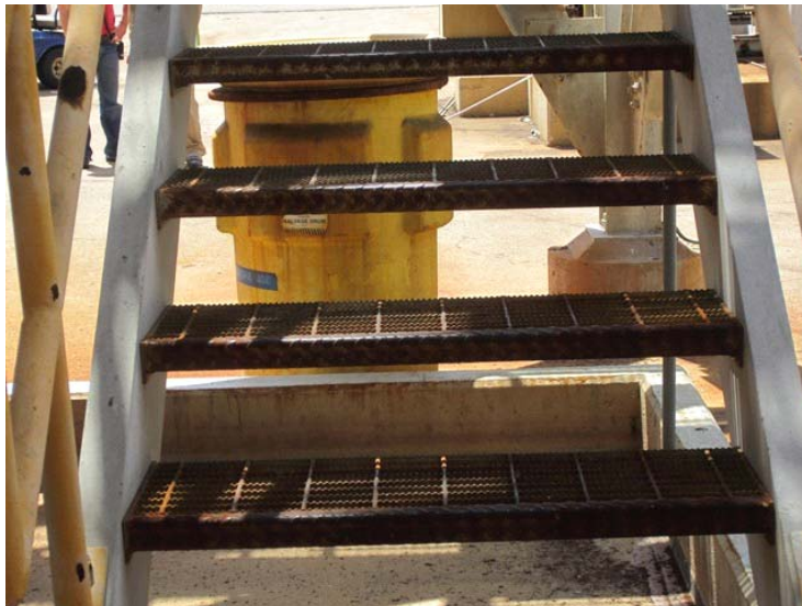
Corrosion on stairs
