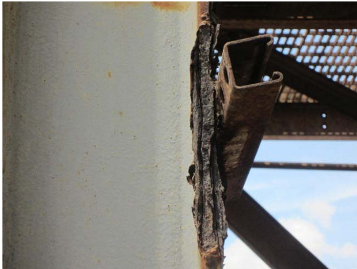
Metal loss on structure
