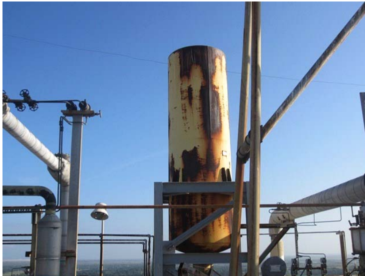
Heavy corrosion occurring
