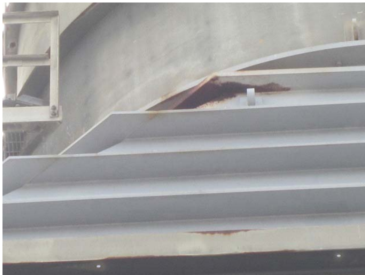
Corrosion on stack
