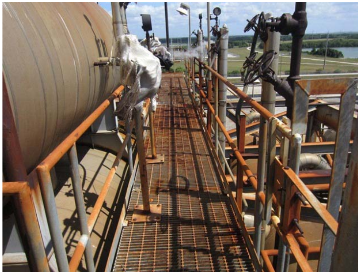
Corrosion on handrails and valves
