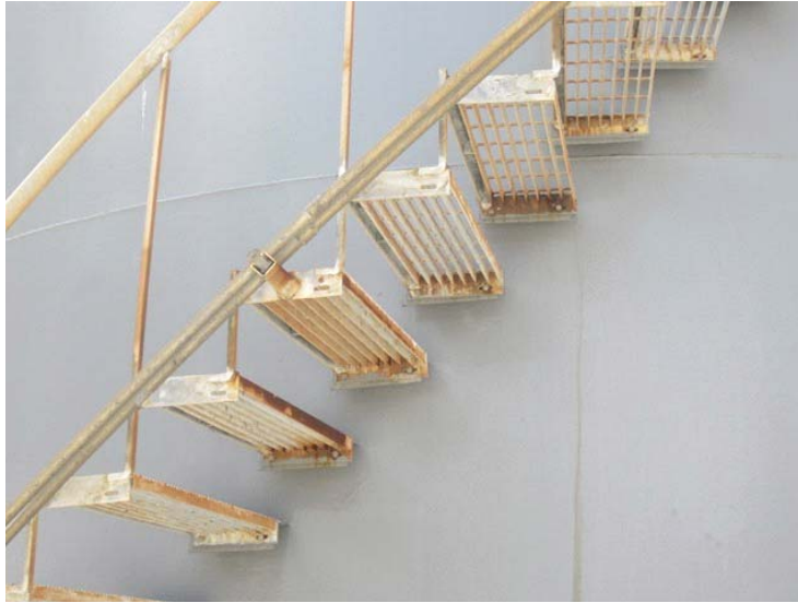
Corrosion on tank stairs
