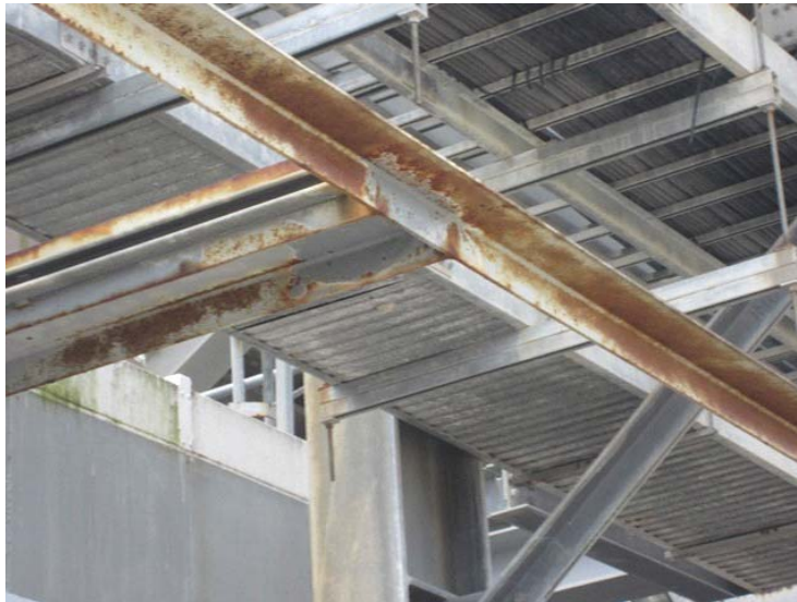
Corrosion on structure
