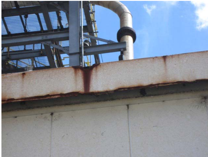
Heavy corrosion on building structure
