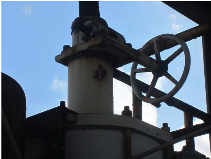
View of corrosion on valve
