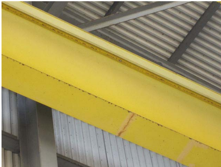
View of minor corrosion on crane rail
