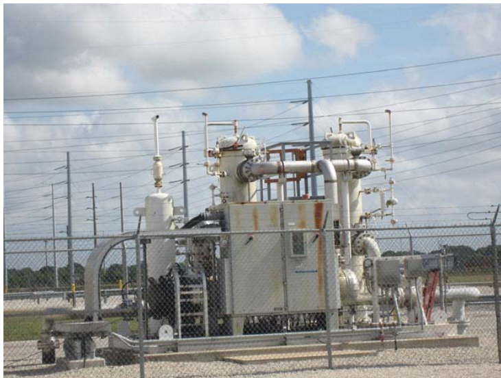
General view of equipment in section
