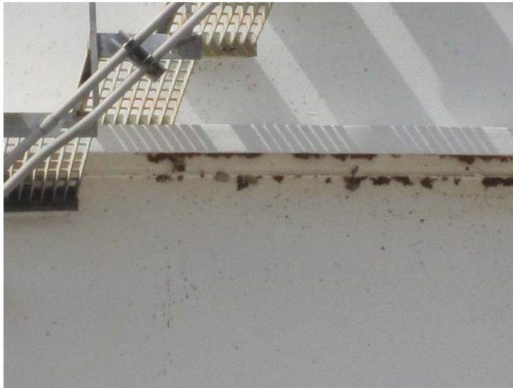
Coating wear visible
