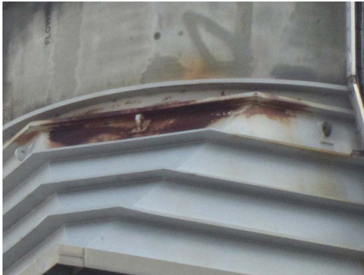
Corrosion on stack structure
