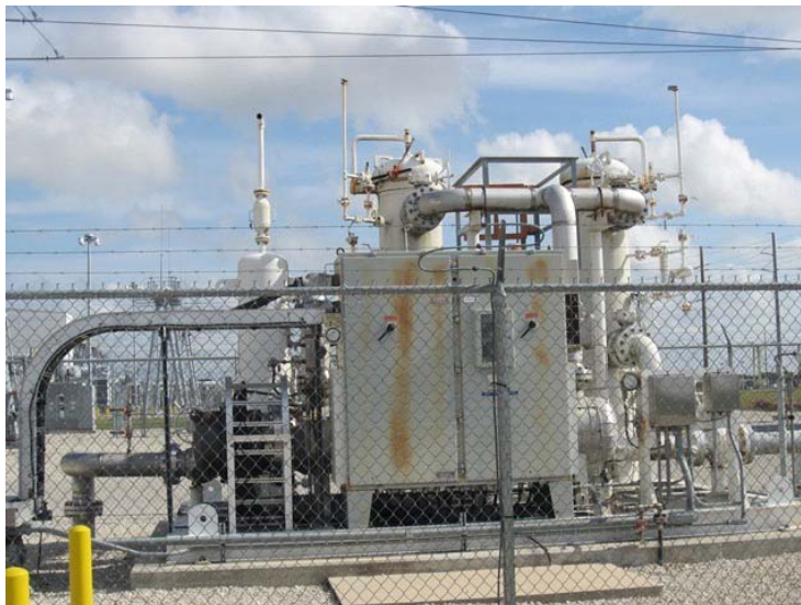
General view of equipment in section
