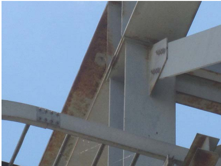
Corrosion on structure
