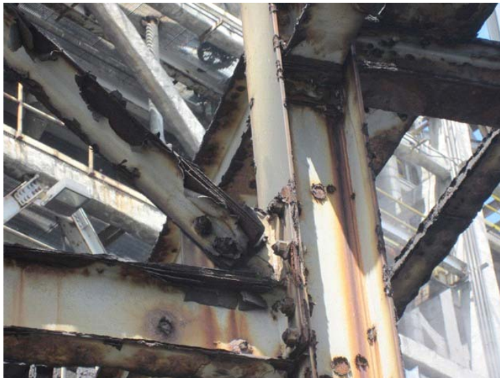
Heavy corrosion on structure
