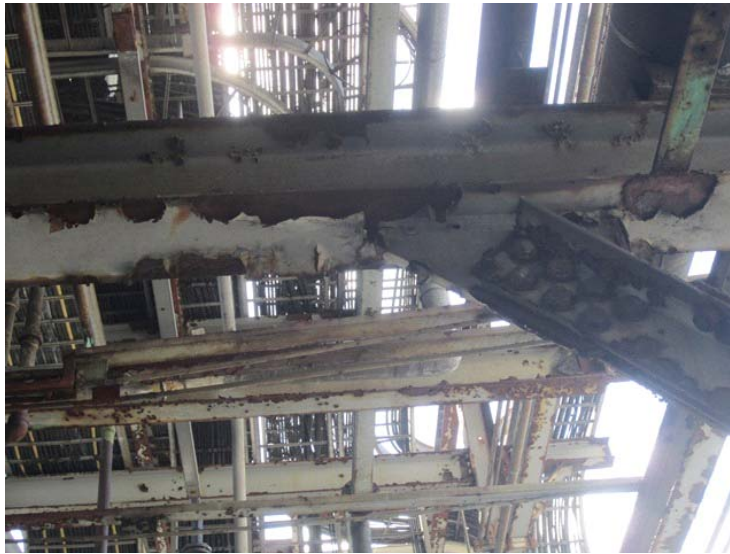
Corrosion on structure
