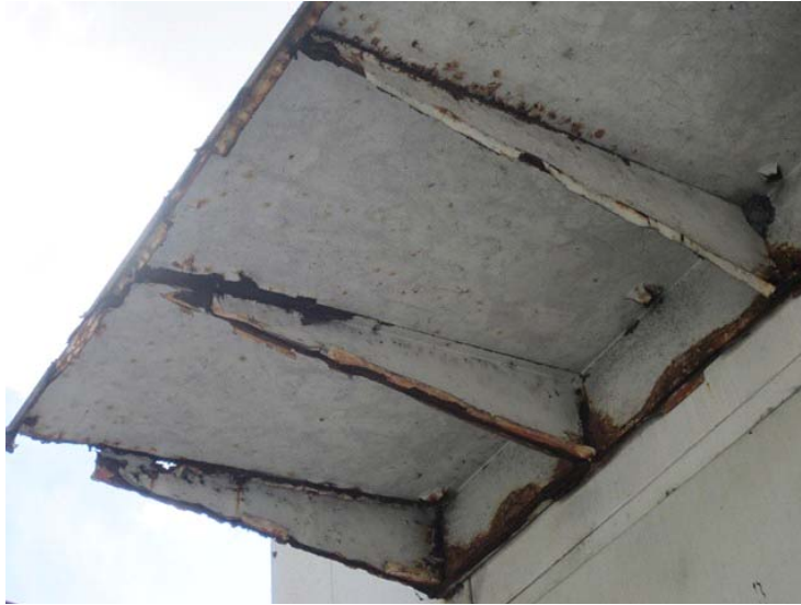
View of corrosion on building
