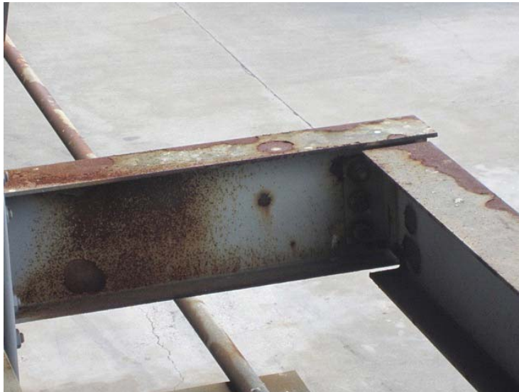
View of corrosion on structure in section
