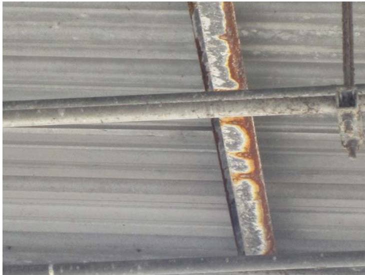
Corrosion on structural steel
