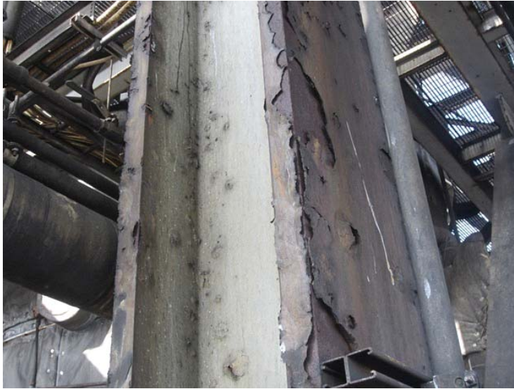
Corrosion on structure
