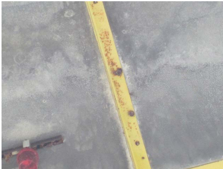
Pin hole rust on structure
