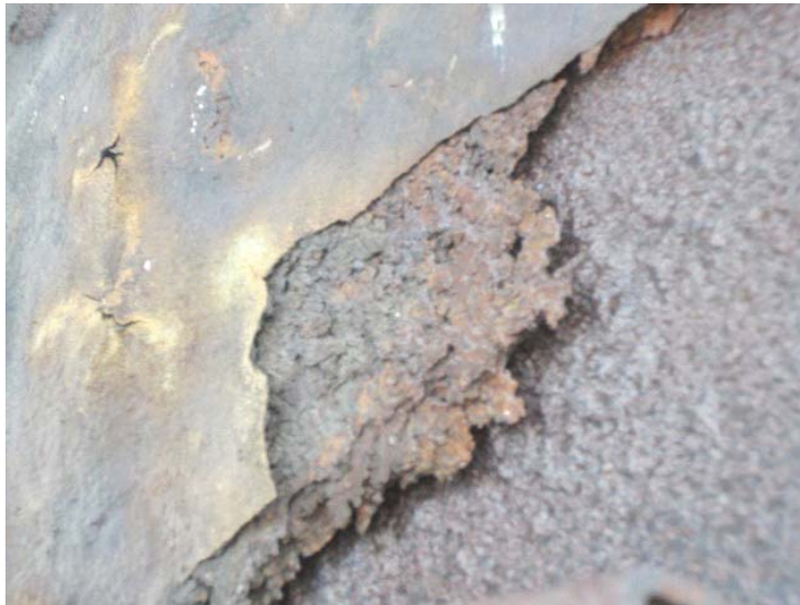
Close up view of metal loss
