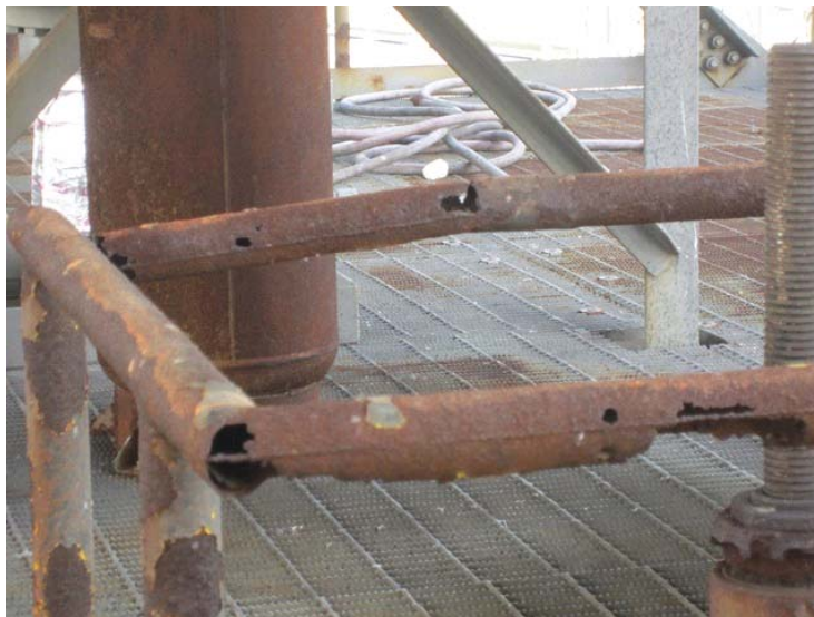
Metal loss on rails
