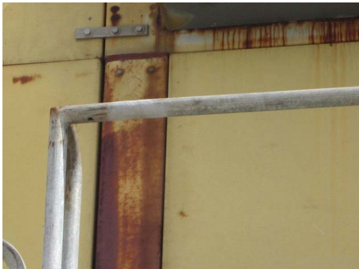
Corrosion on building
