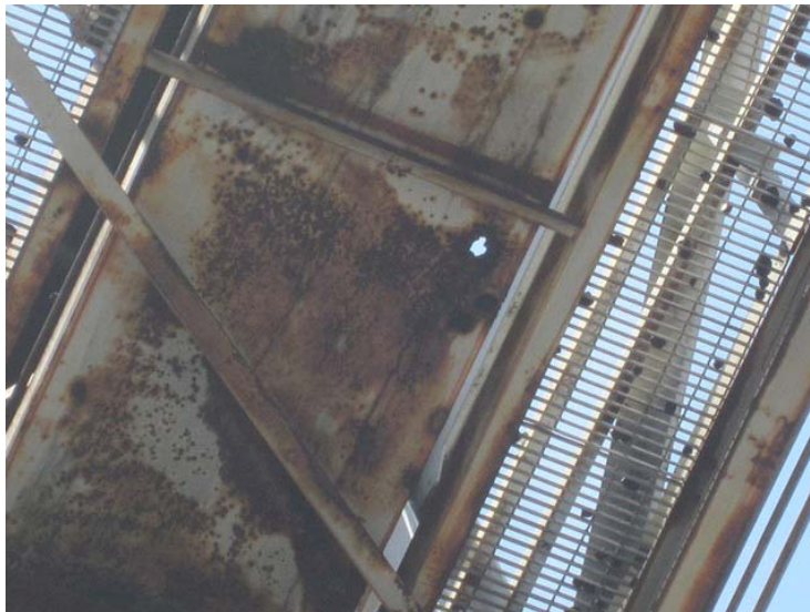
View of corrosion on structure
