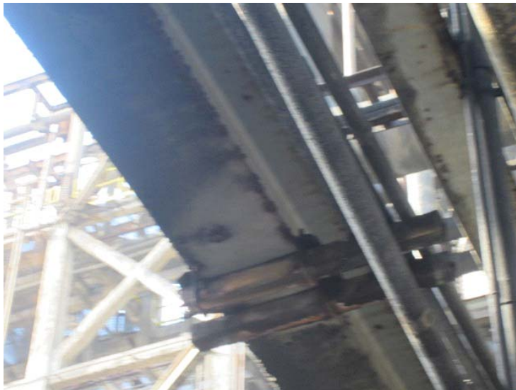
Corrosion on structure
