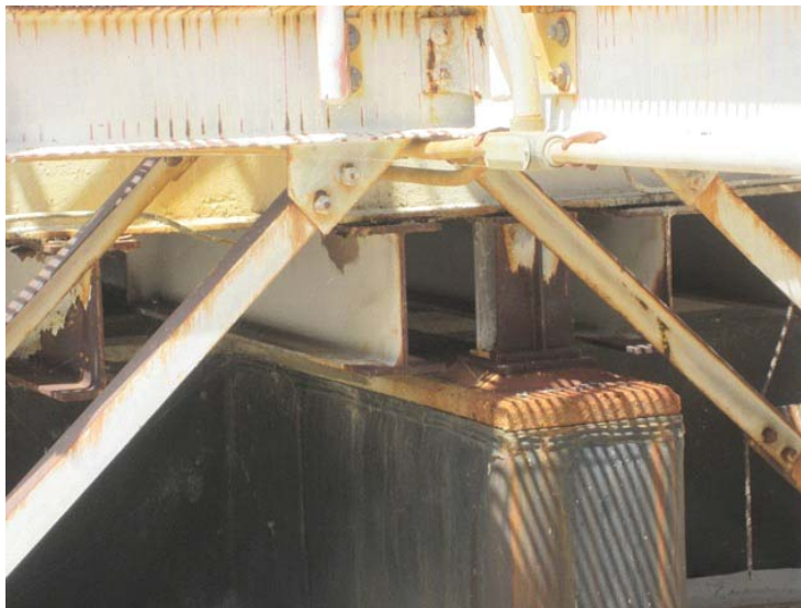
Corrosion on structure
