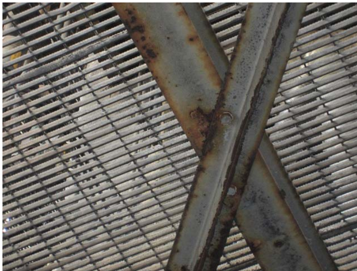
Corrosion occurring on supports
