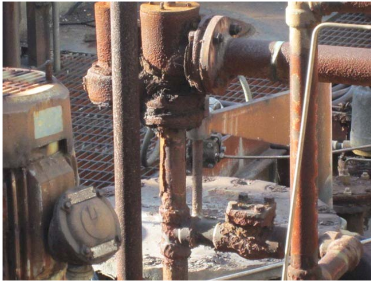
Corrosion on piping
