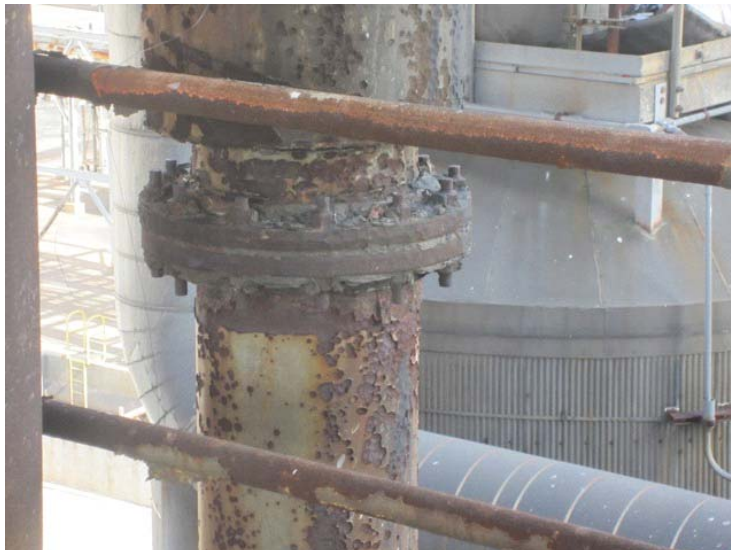
Heavy corrosion on pipe
