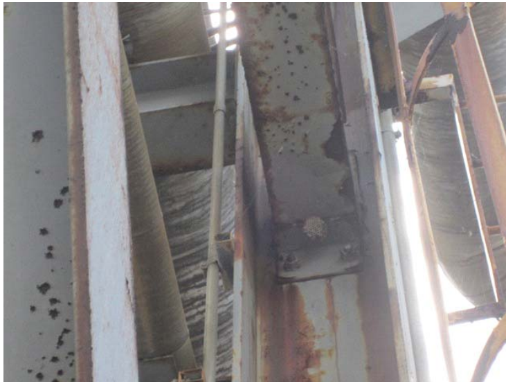
Corrosion on structure
