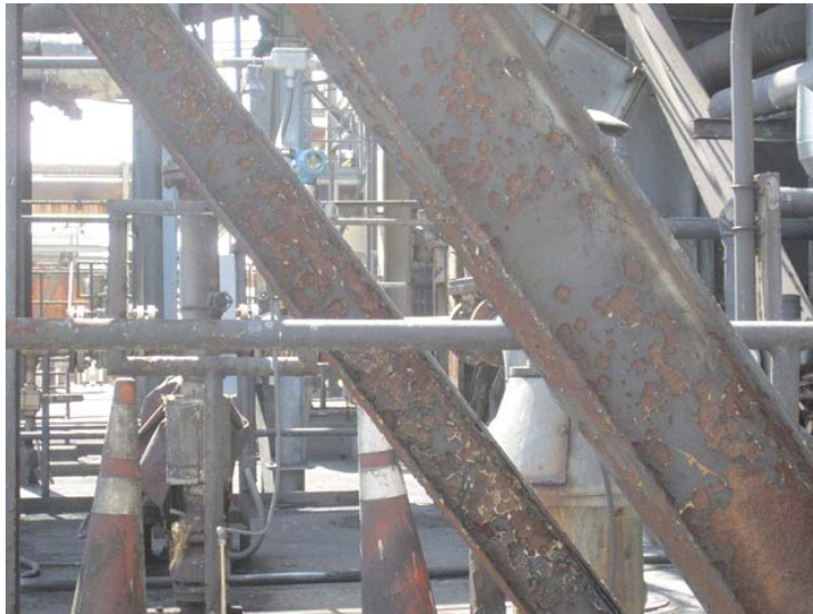
Heavy corrosion on structure
