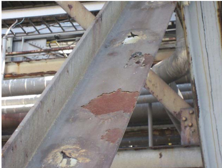
Visible undercutting on structure
