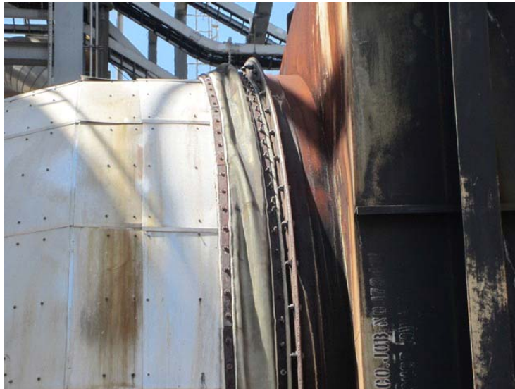
Corrosion in section
