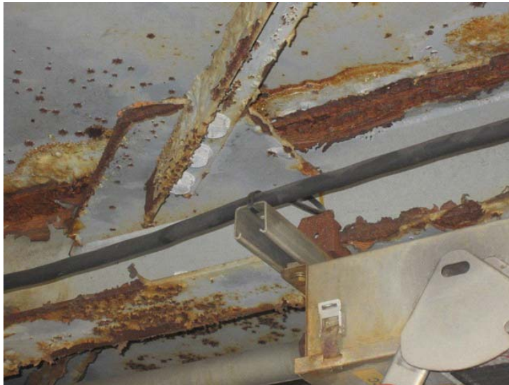
Heavy pitting rust
