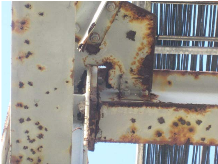
Heavy corrosion on structure
