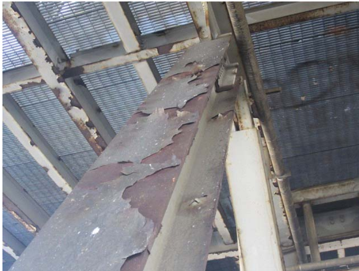
View of corrosion on structure
