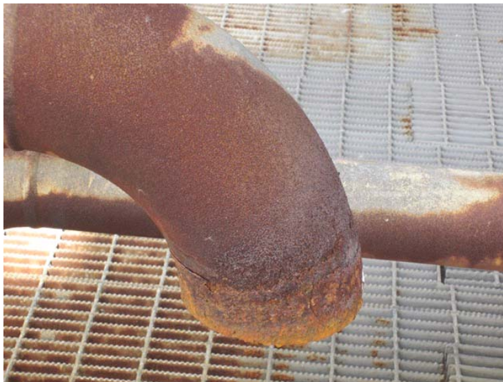
Corrosion on piping in section
