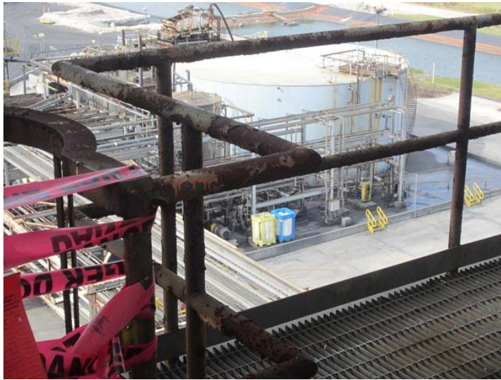
Corrosion on handrails
