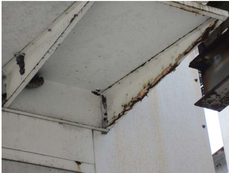
Corrosion on building structure
