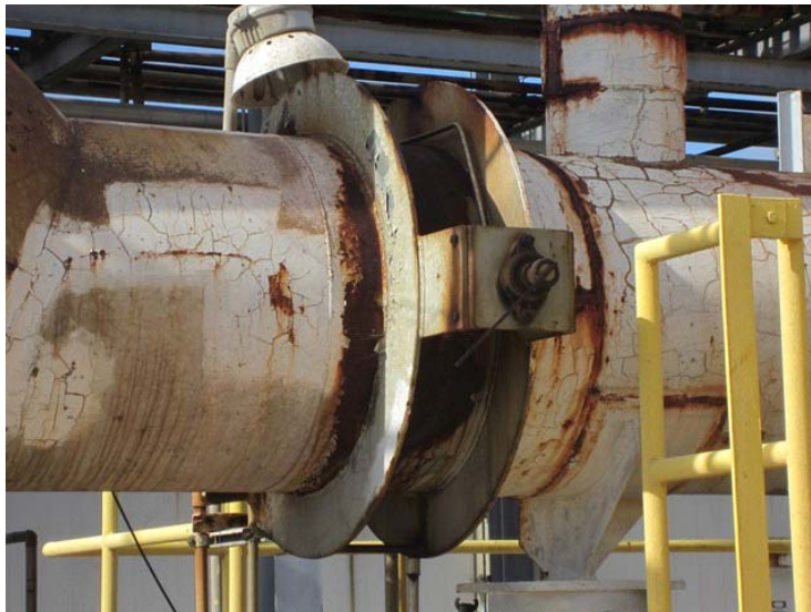
Corrosion on pipe
