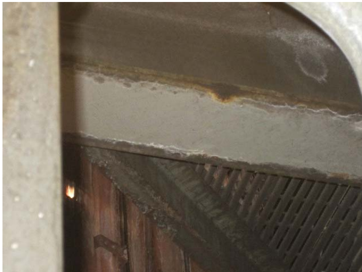
Corrosion on structure
