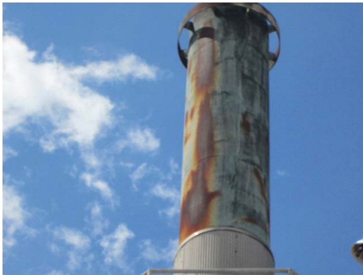
Corrosion on stack
