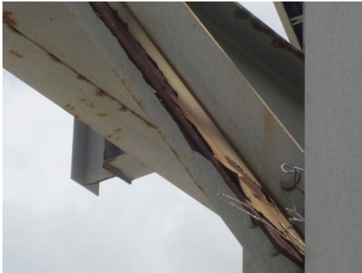
Corrosion on support structure
