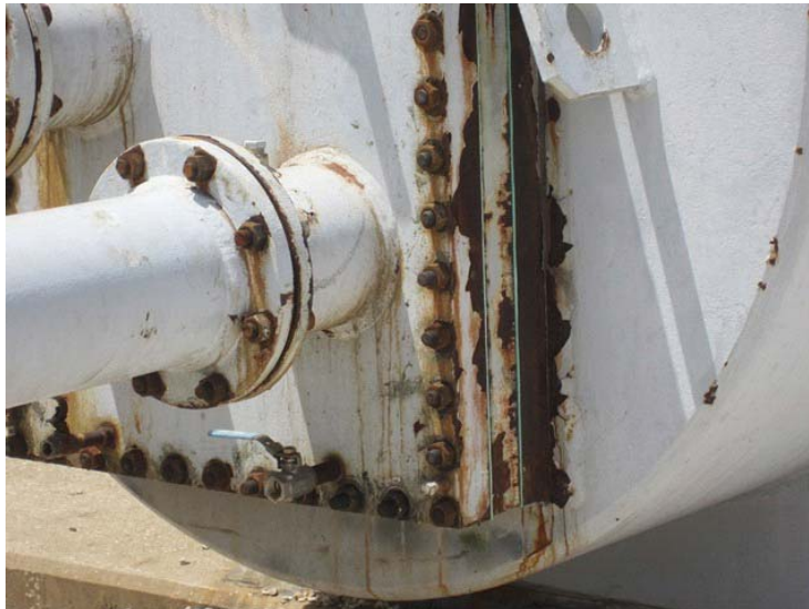
Corrosion on vessel
