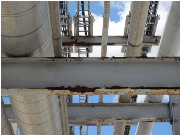
Corrosion on structure
