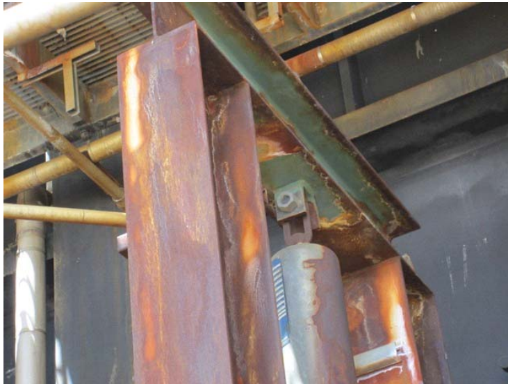
Heavy corrosion on supports
