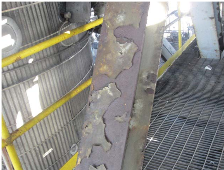
Undercutting visible on structure
