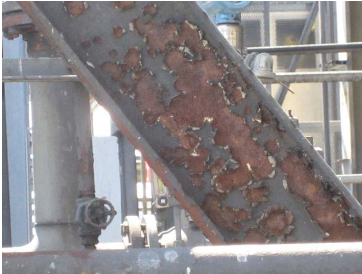
View of corrosion on structure
