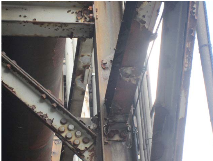
Corrosion on structure
