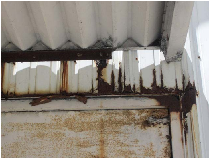
Corrosion on structure
