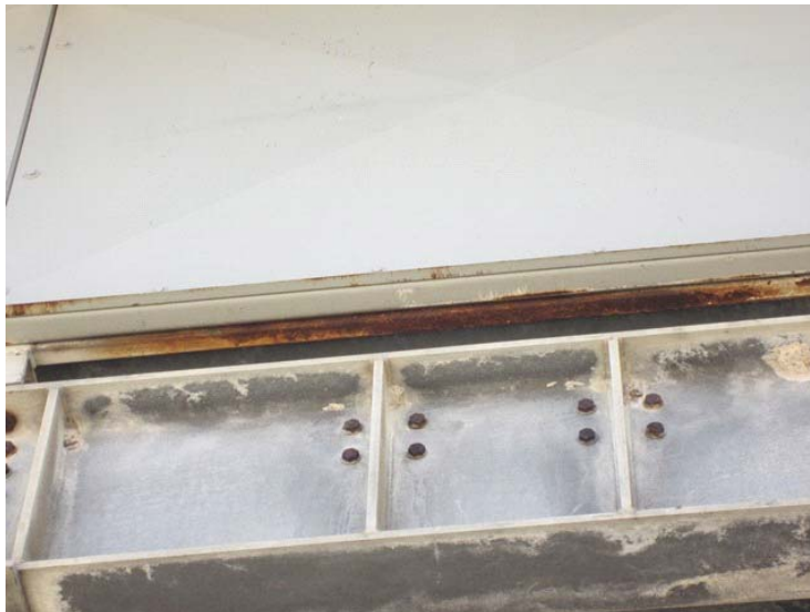
Corrosion on filter structure
