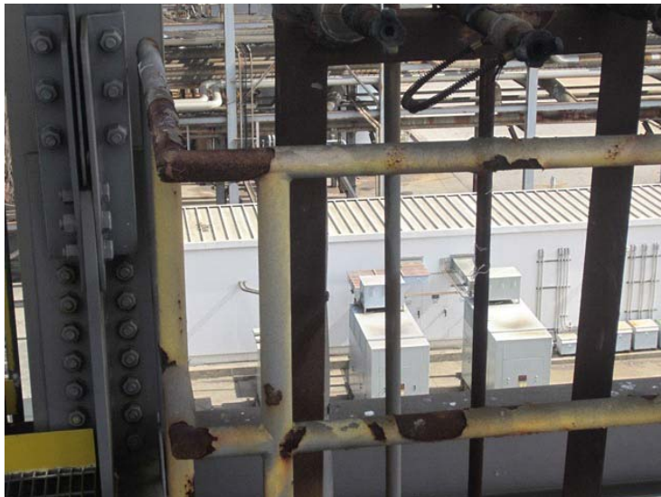
Corrosion on handrails
