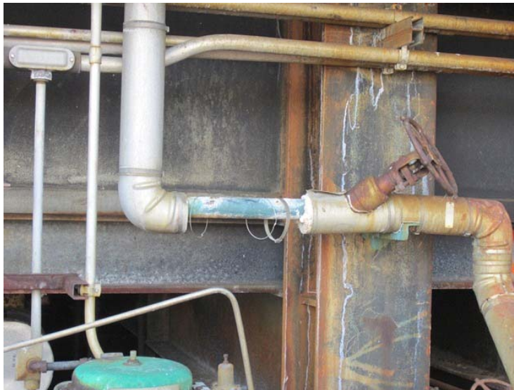
Corrosion on piping in section
