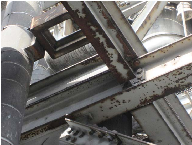
Corrosion on structure
