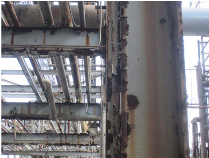
Corrosion on structure
