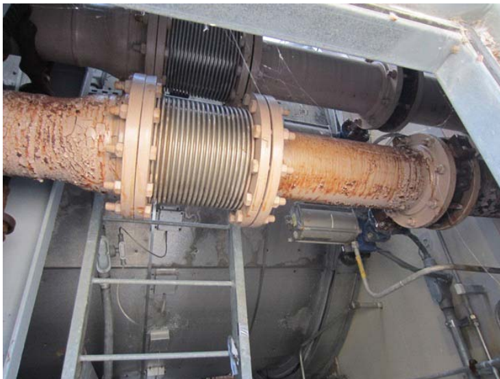
Heavy corrosion on piping
