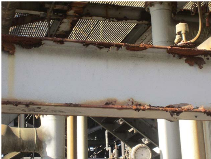
Corrosion on structure
