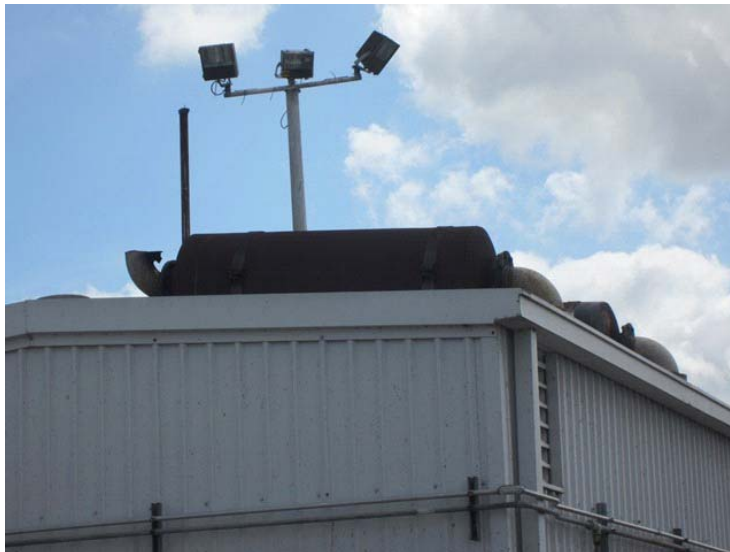
Corrosion visible on vessels
