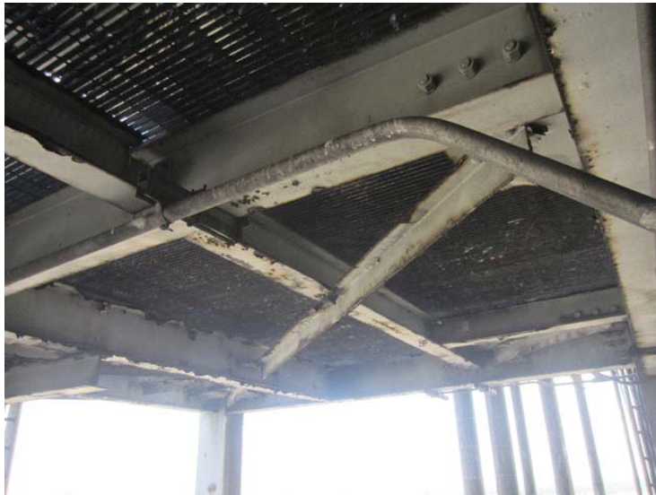
Corrosion on support structure
