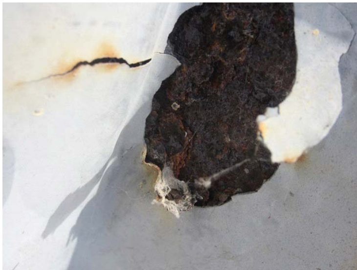
Close up view of corrosion
