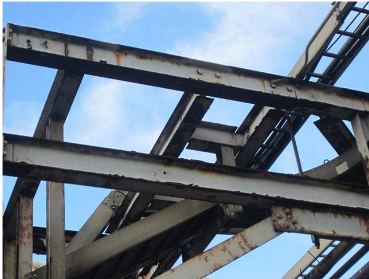
View of corrosion on structure
