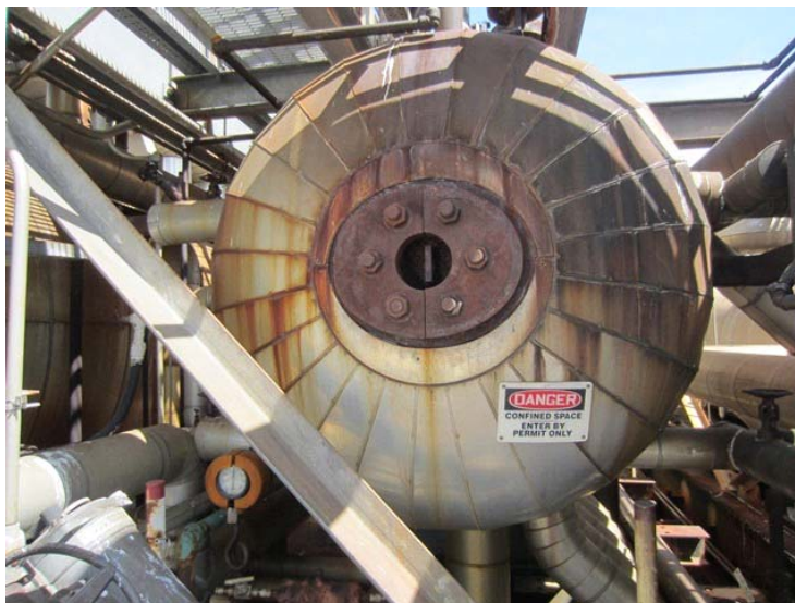
Corrosion on equipment
