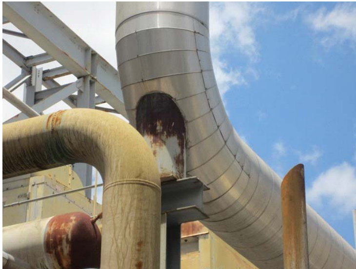
Corrosion on supports
