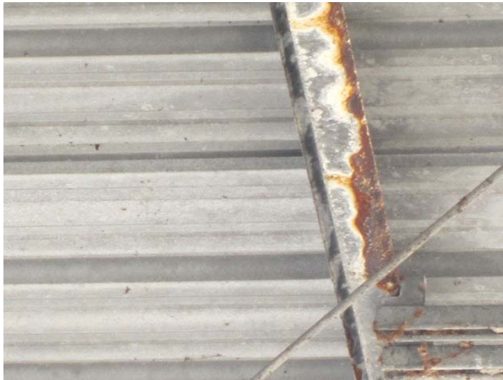
Corrosion on structure
