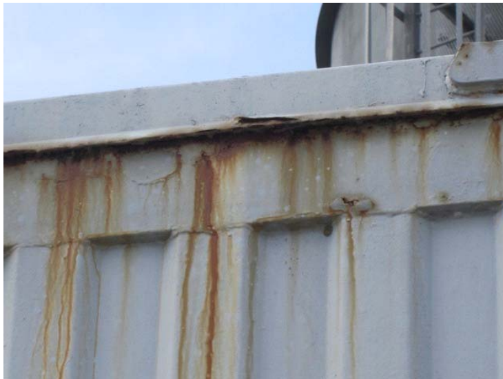
Heavy corrosion on structure
