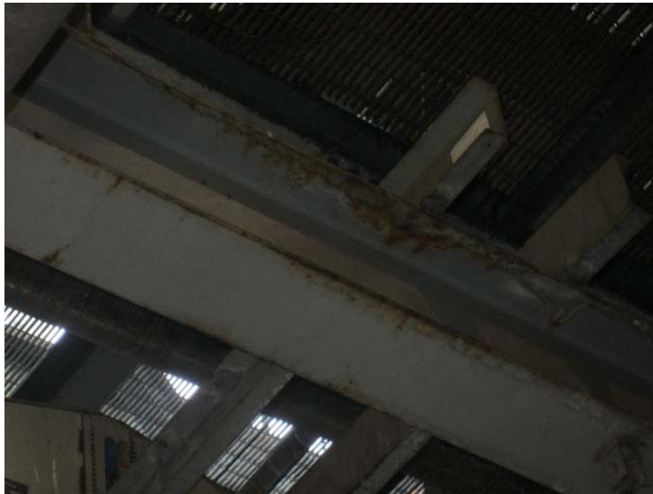
Edge corrosion occurring
