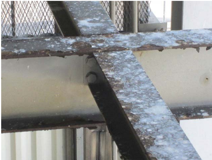
Corrosion on support structure
