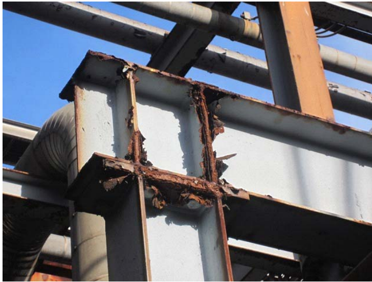
Corrosion on structure
