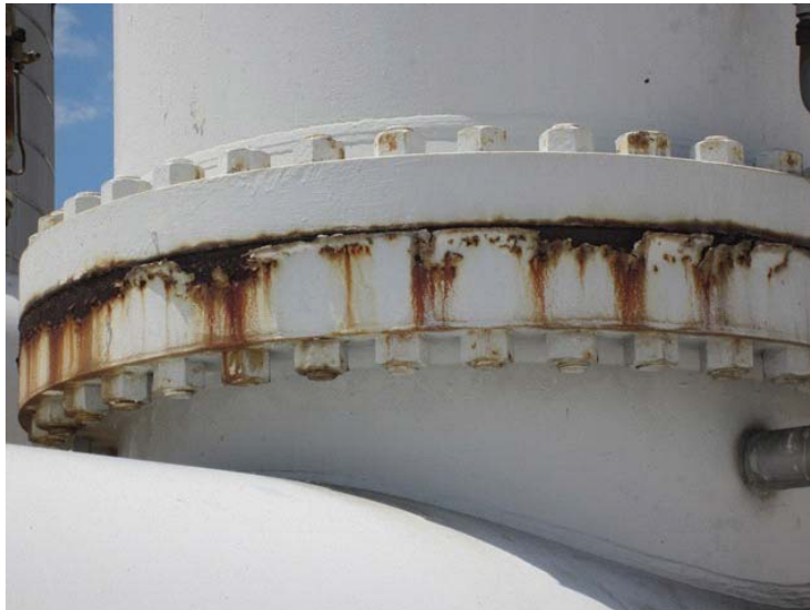
Corrosion on flange
