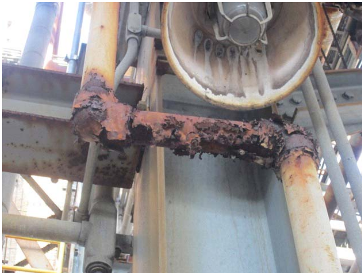
Severe metal loss due to corrosion
