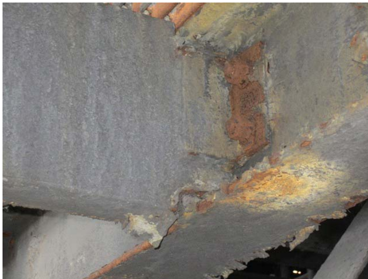
Corrosion on structure
