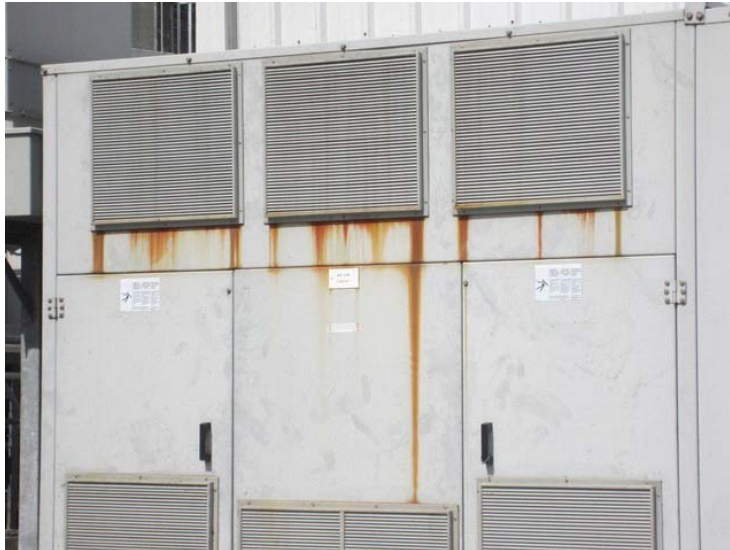
Corrosion on electrical boxes
