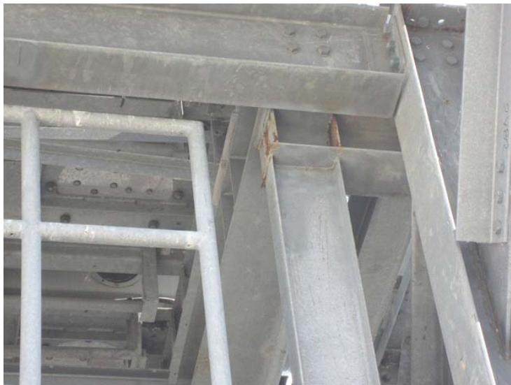
Minor corrosion in section
