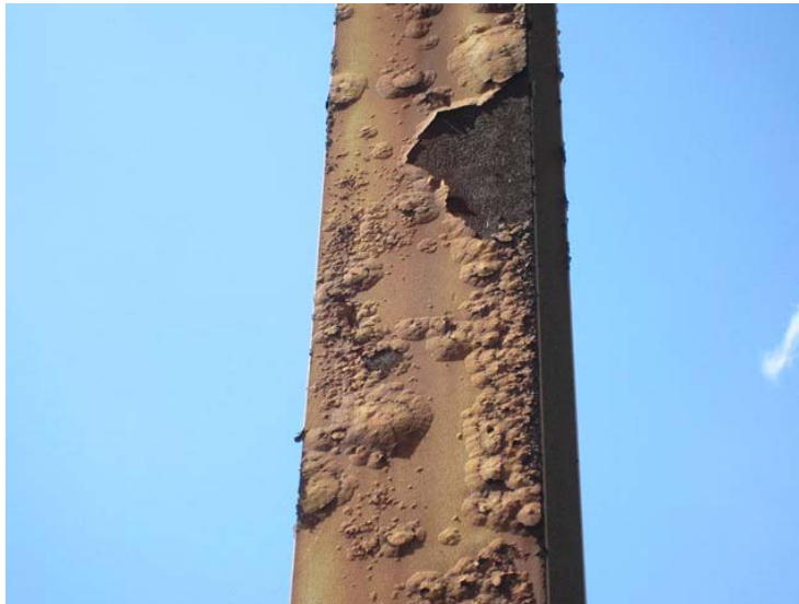
Severe corrosion on structure
