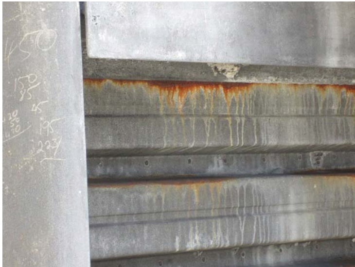
Corrosion on siding
