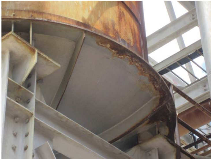
Corrosion on structure
