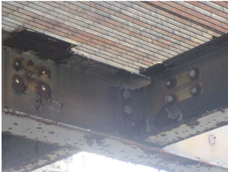
Corrosion on structure in section
