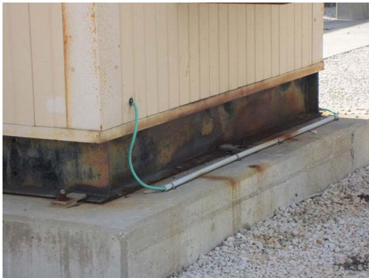
Heavy corrosion on building structure
