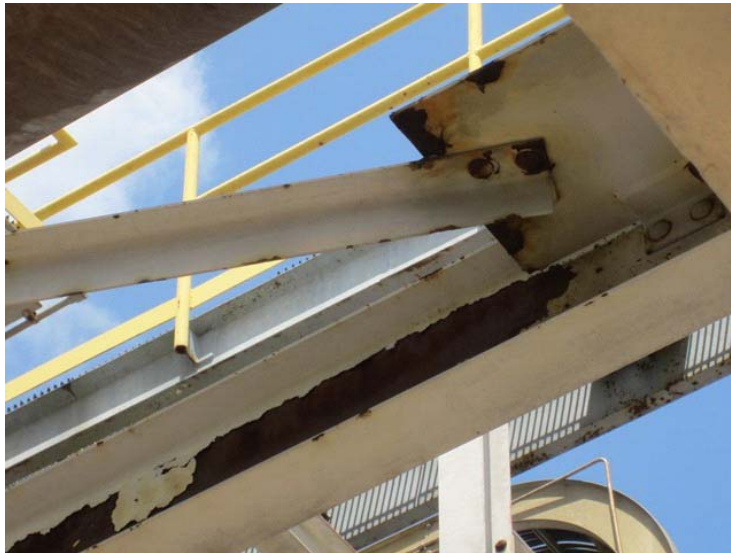
Corrosion on structure
