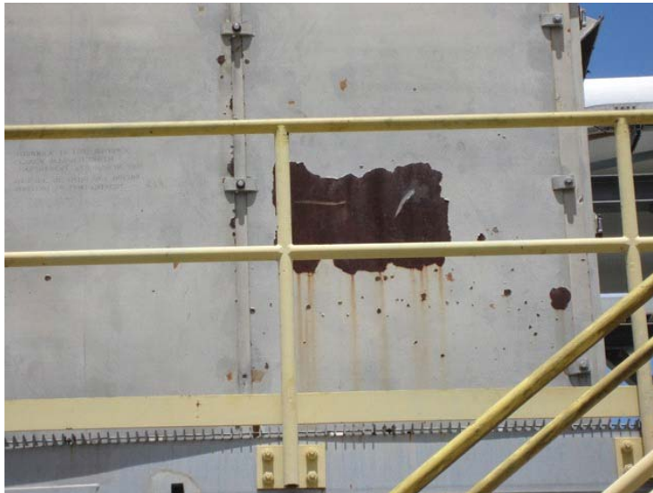
Corrosion on equipment structure
