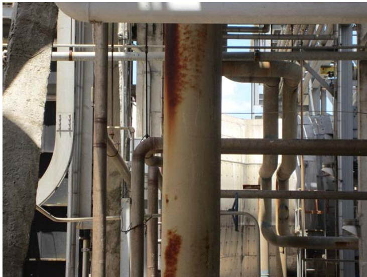
Corrosion on piping in section
