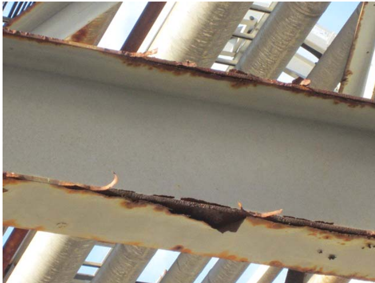
View of corrosion occurring on structure
