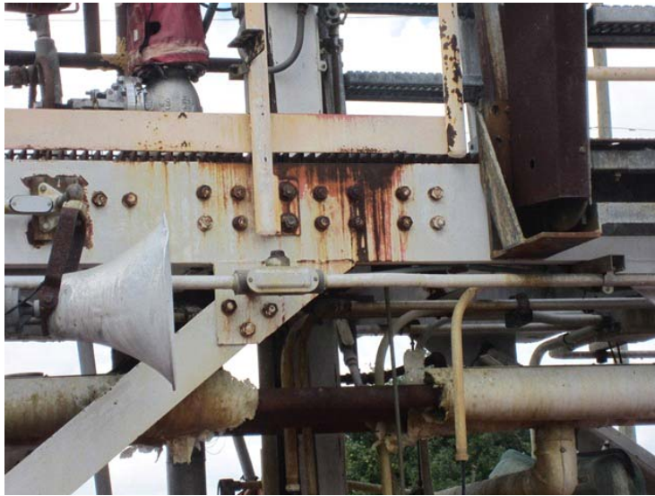
Corrosion on structure
