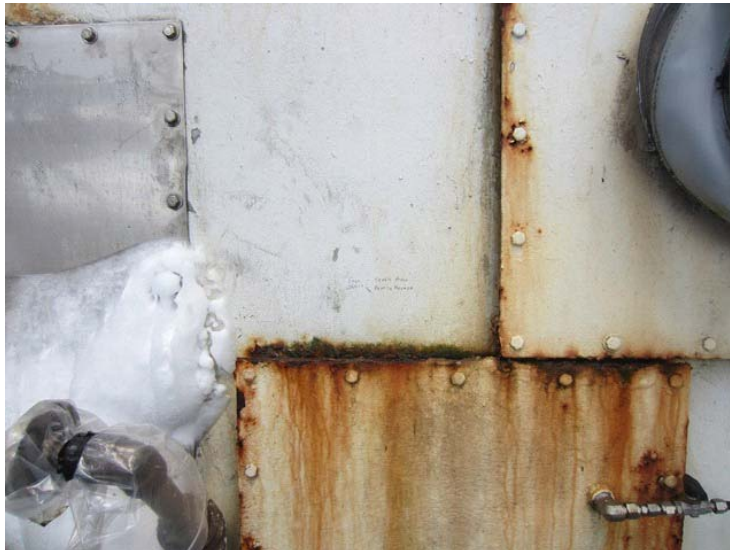
Corrosion on cold box
