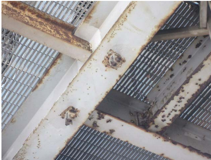
Corrosion on support structure
