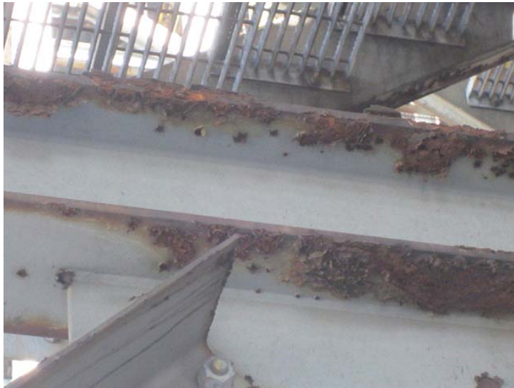
Heavy corrosion on structural steel
