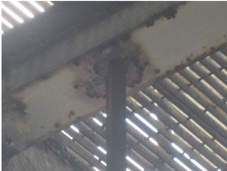
Heavy corrosion on structure
