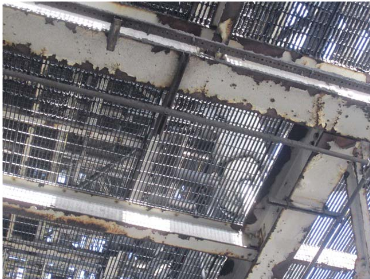
Heavy corrosion on structure
