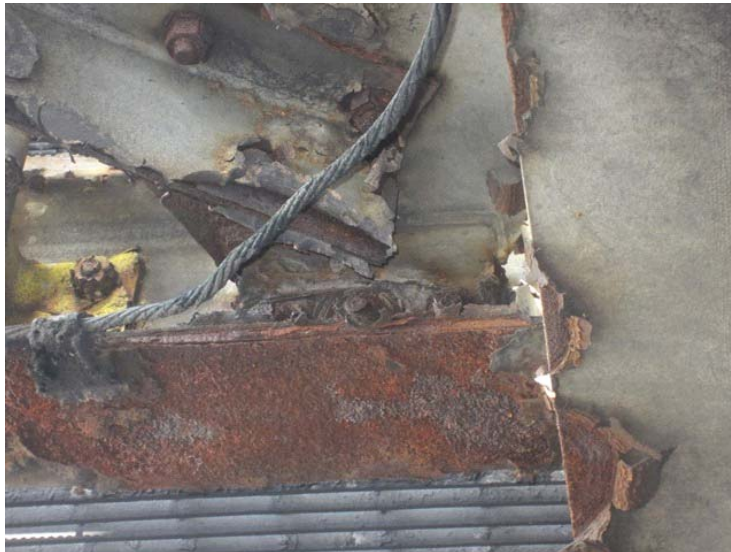
Heavy corrosion occurring on structure
