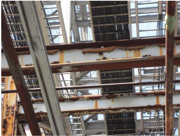
Heavy corrosion on structural steel
