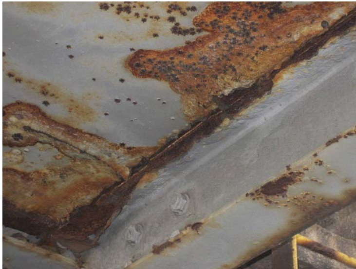
Pitting rust occurring
