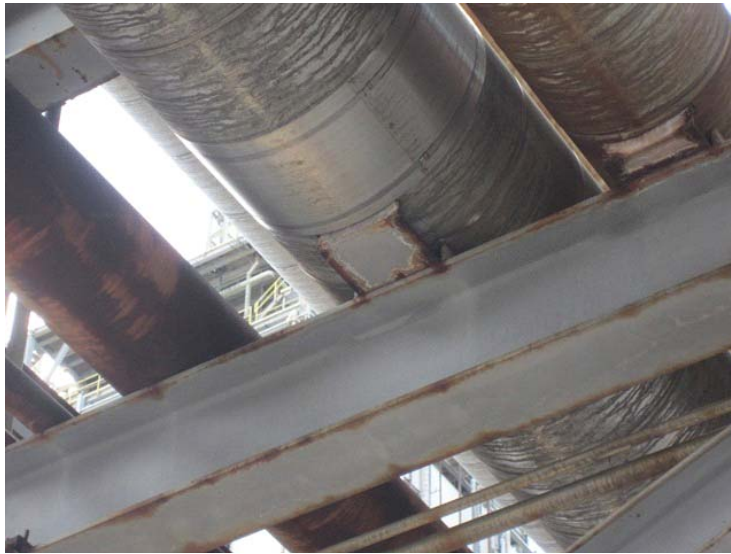
View of corrosion in section
