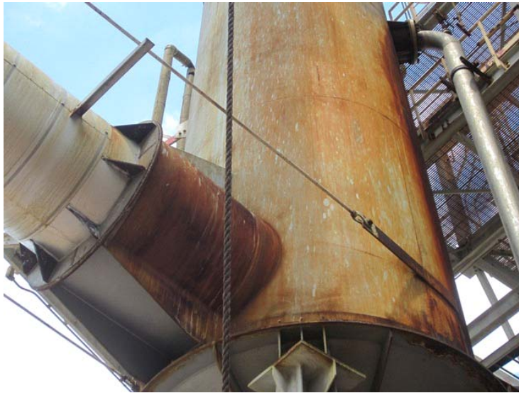
Corrosion on stack
