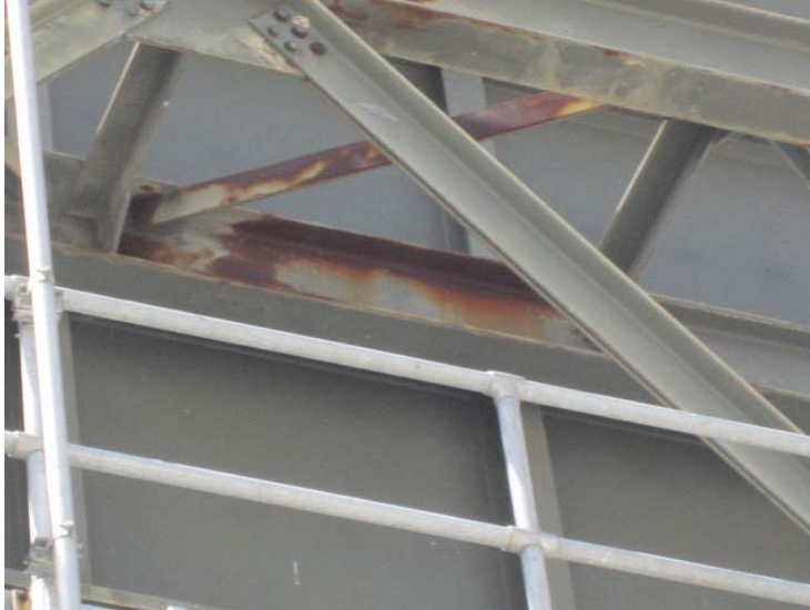
Corrosion on structure
