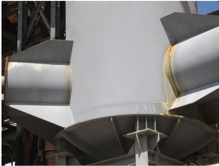
minor corrosion on stack
