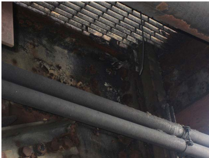
View of corrosion on support structure
