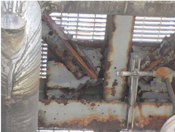
Severe corrosion on structure
