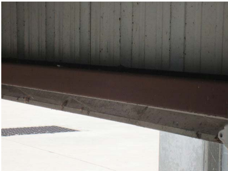
Corrosion on structure
