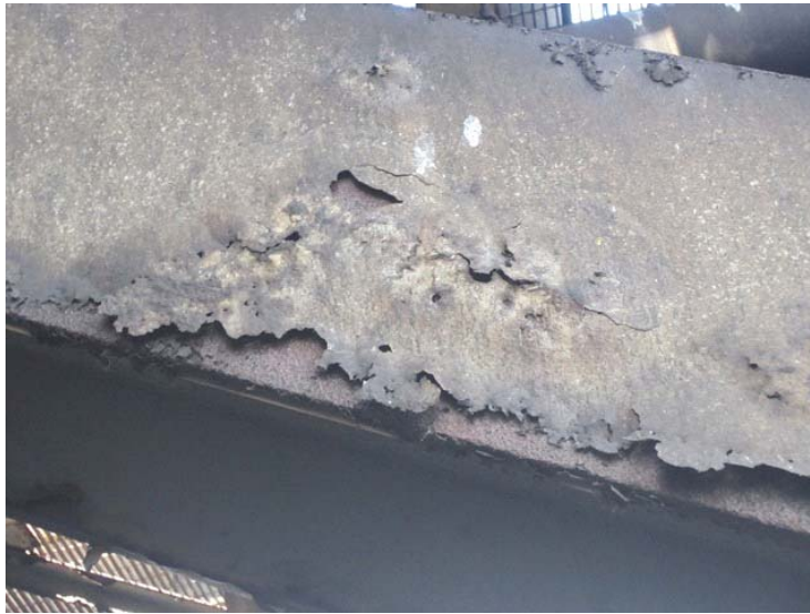
Severe corrosion occurring
