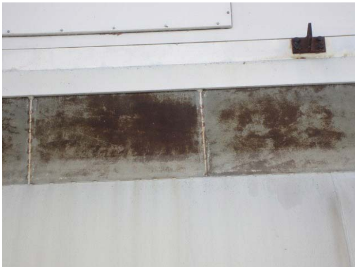
Corrosion on generator
