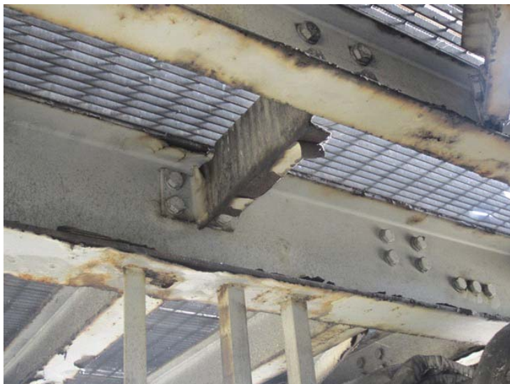
Edge corrosion on structure
