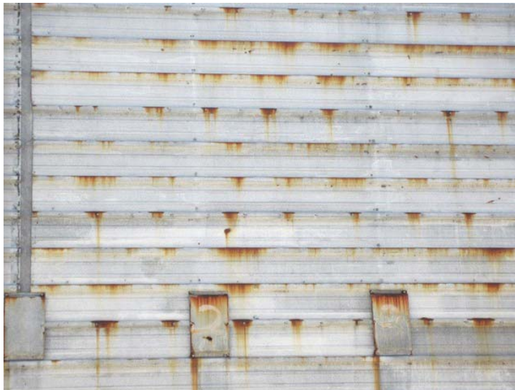
Uniform corrosion on siding
