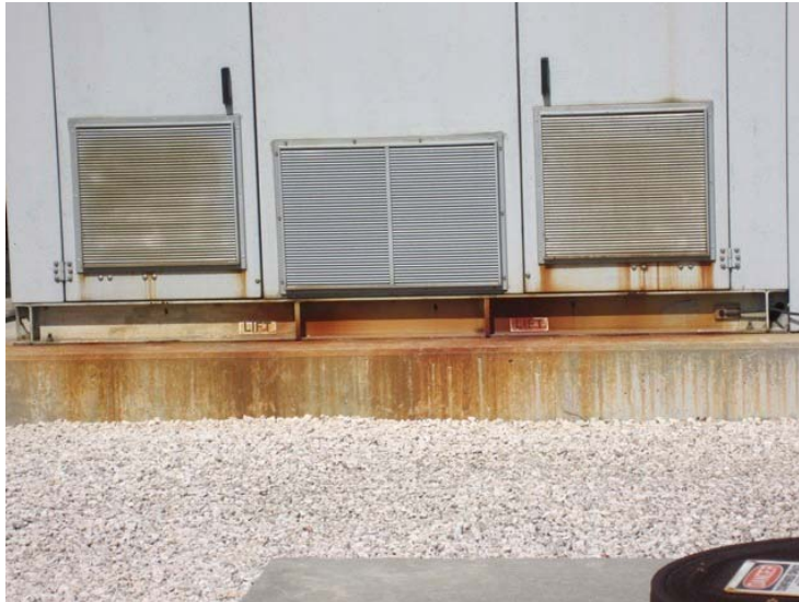
Corrosion on building structure
