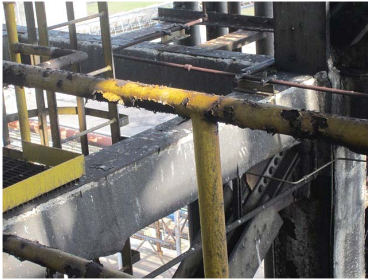
Corrosion on handrails
