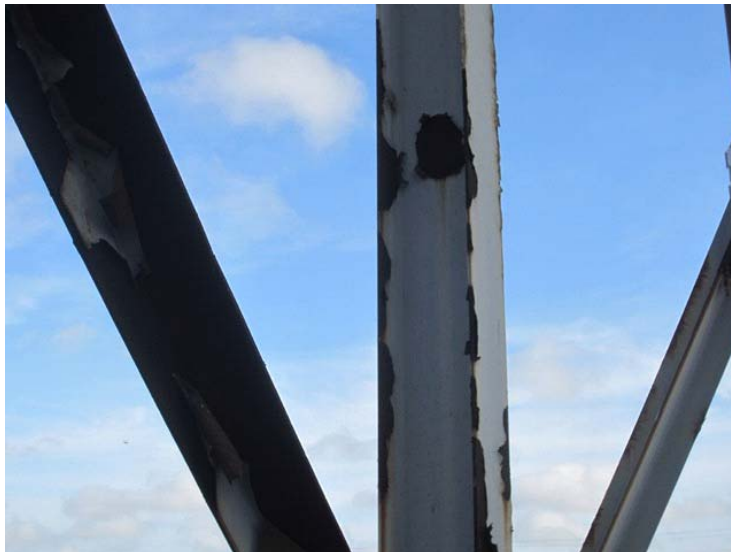
Corrosion on structure
