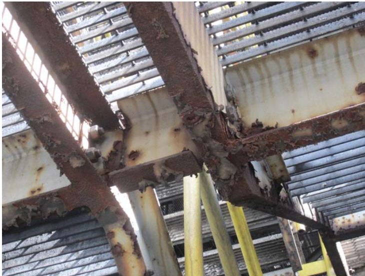
Severe corrosion on structure
