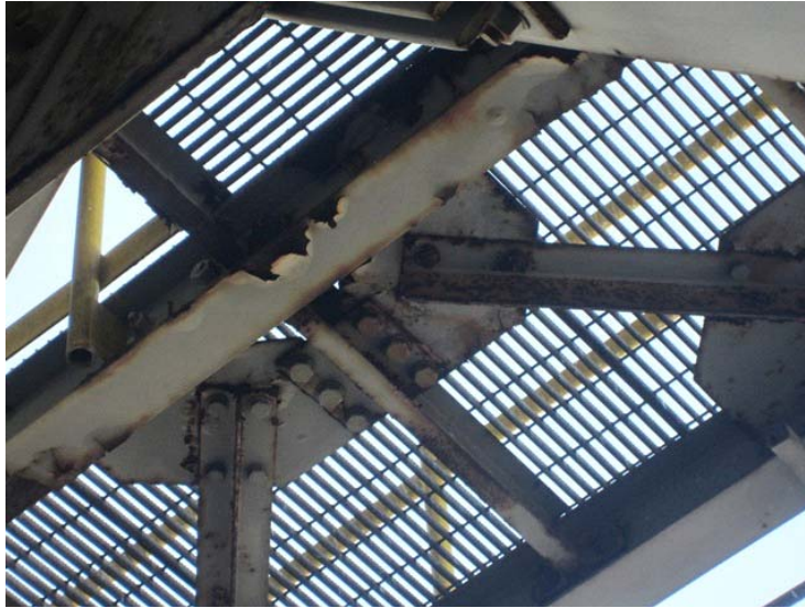
Undercutting visible on structure
