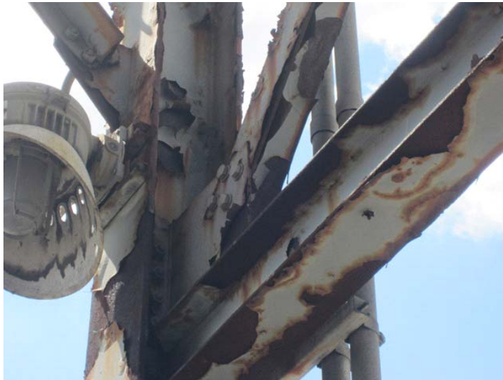
View of corrosion in section
