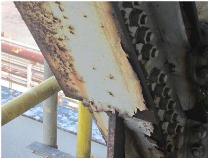
Close up view of corrosion
