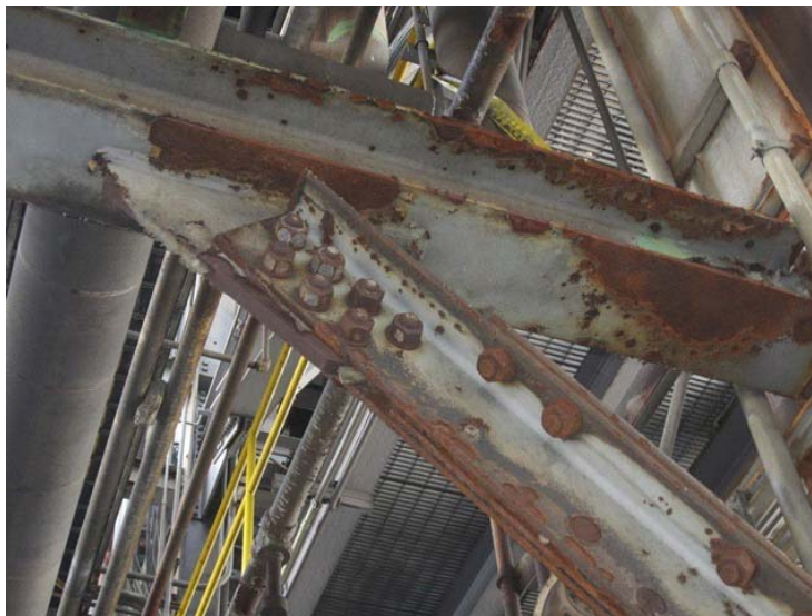
Corrosion occurring on structure
