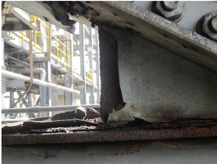
Metal loss visible
