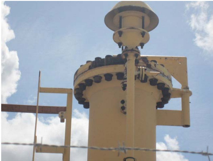
Corrosion on flange
