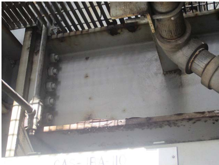
Corrosion on structure
