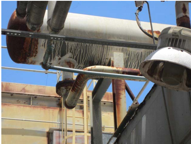
Corrosion on piping and structure
