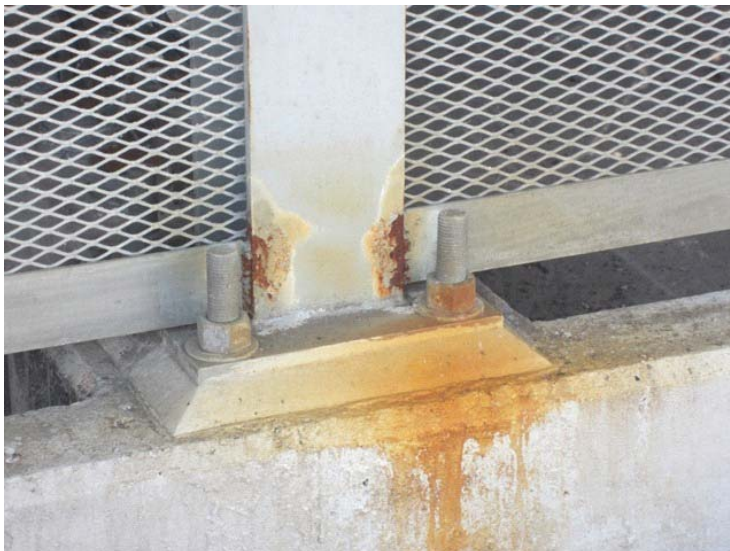
Corrosion on structure
