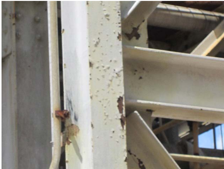
Corrosion visible on structure
