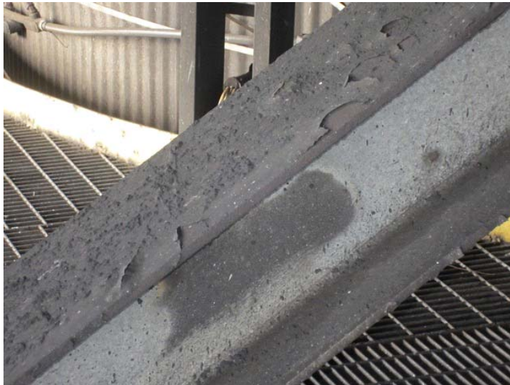
Undercutting visible on structure
