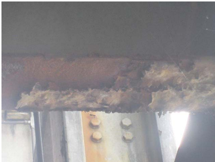
Heavy corrosion on structural steel
