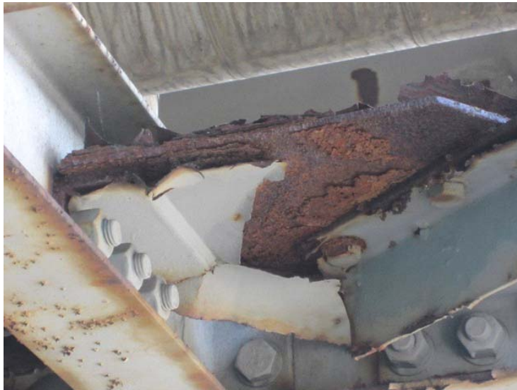
Heavy corrosion on supports
