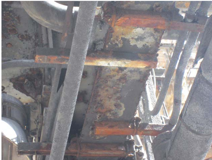
Corrosion occurring on structure
