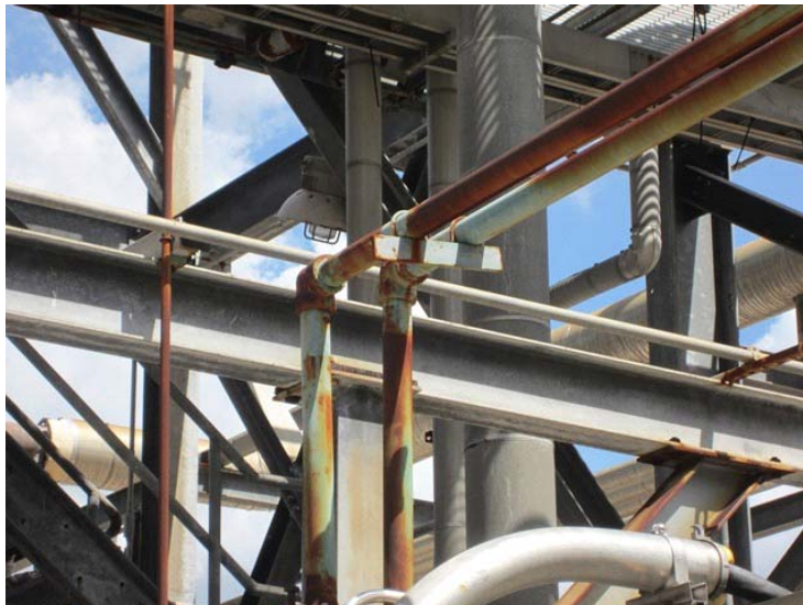
View of corrosion on piping
