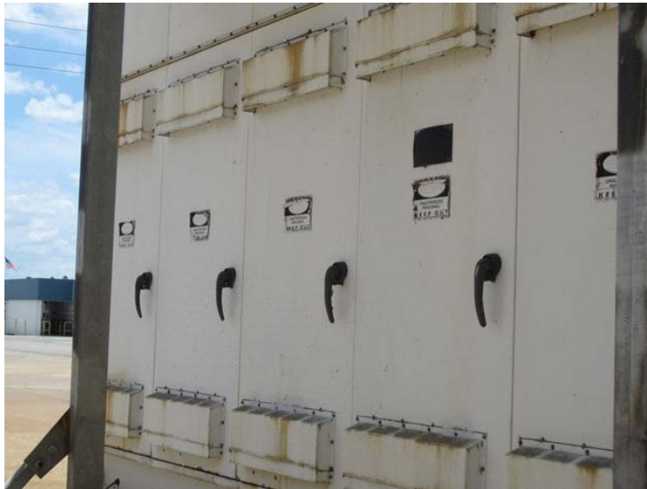
View of minor corrosion on electrical boxes
