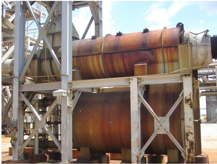
Corrosion on equipment
