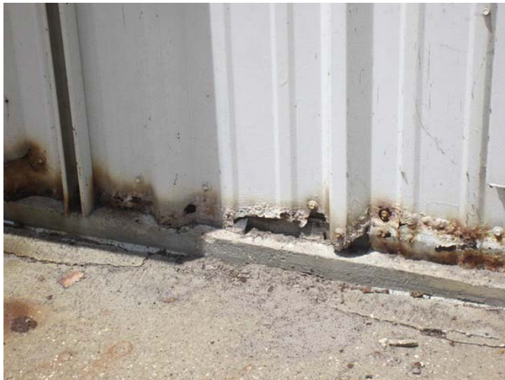
Corrosion at base of siding
