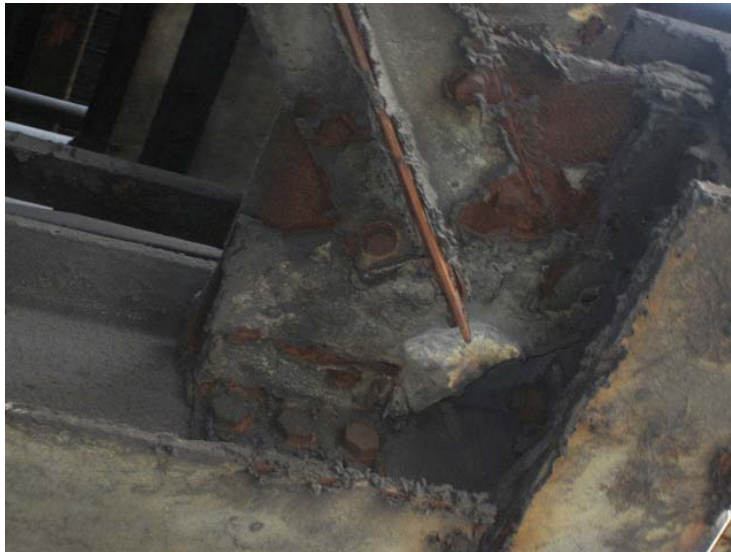
Heavy corrosion on structural supports
