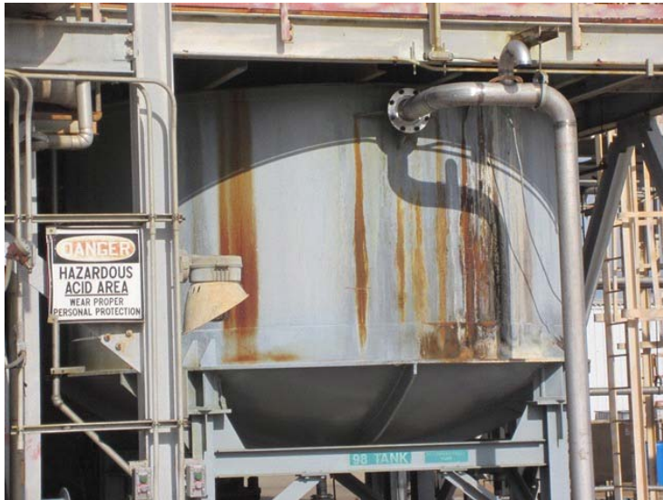
View of corrosion in section
