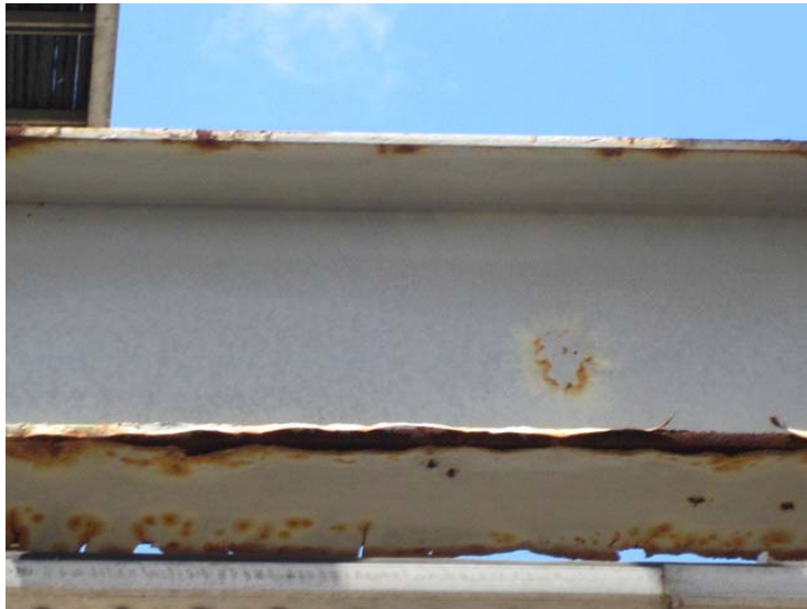
Corrosion on structure
