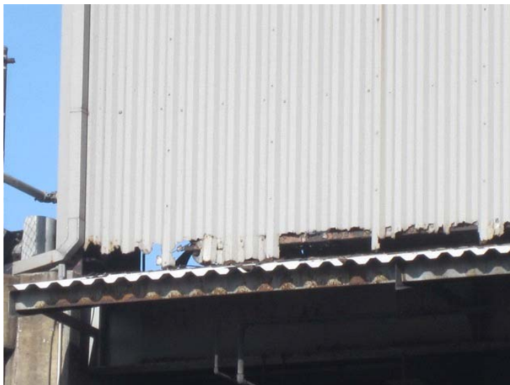
Corrosion on siding
