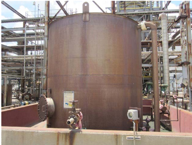
Corrosion on tank
