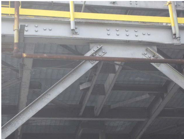
Corrosion on pipe
