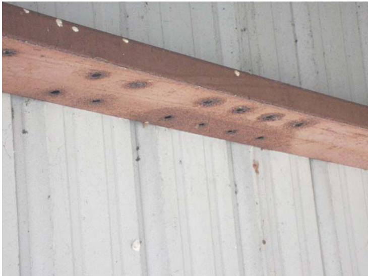
Corrosion on structure
