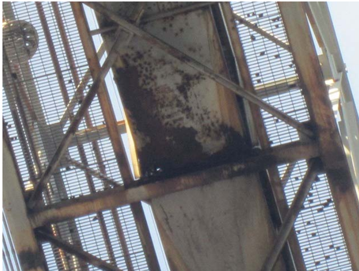
View of corrosion on structure
