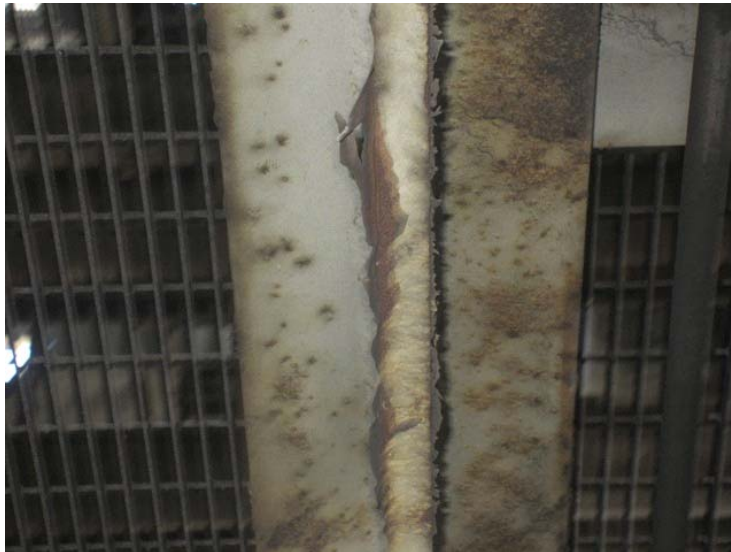
Corrosion on structure
