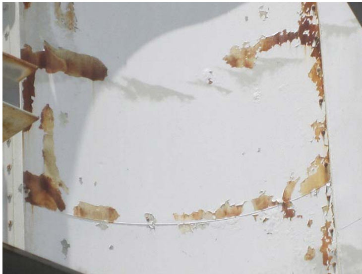
Delamination of coating with corrosion occurring
