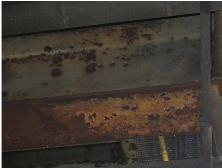
Pitting rust on structure
