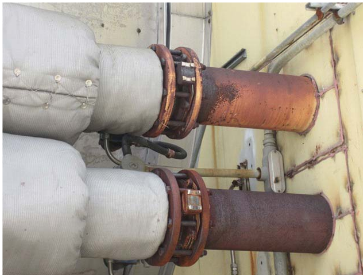
Corrosion on piping
