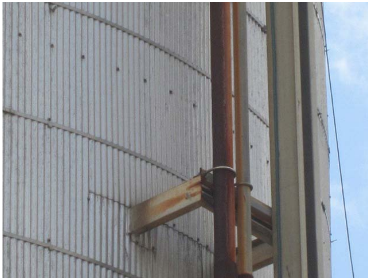
Corrosion on structure and pipe
