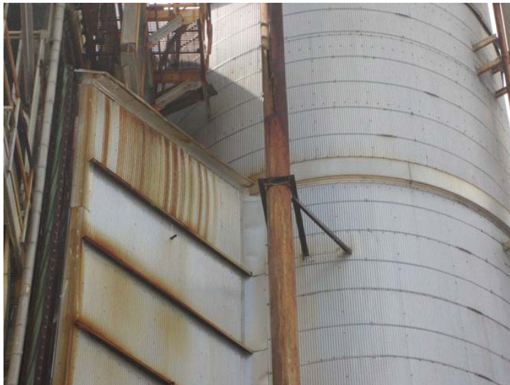
Corrosion on stack structural supports
