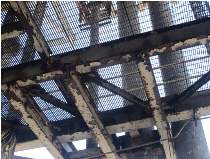
Heavy corrosion on structure
