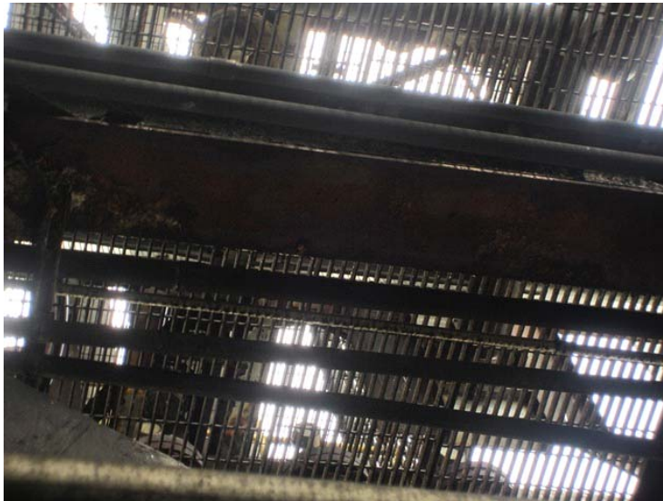
Heavy corrosion on support structure
