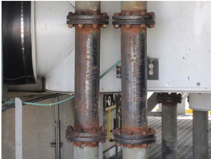
Corrosion on piping
