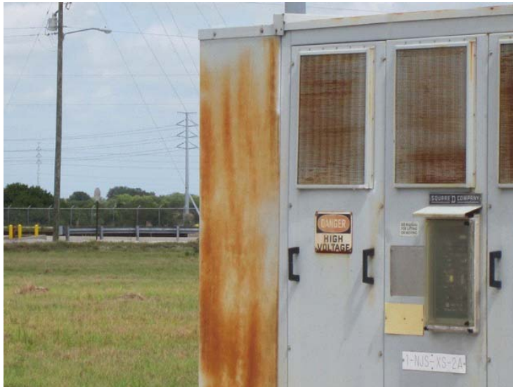
Minor surface rust on electrical boxes
