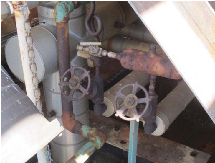
Corrosion on piping
