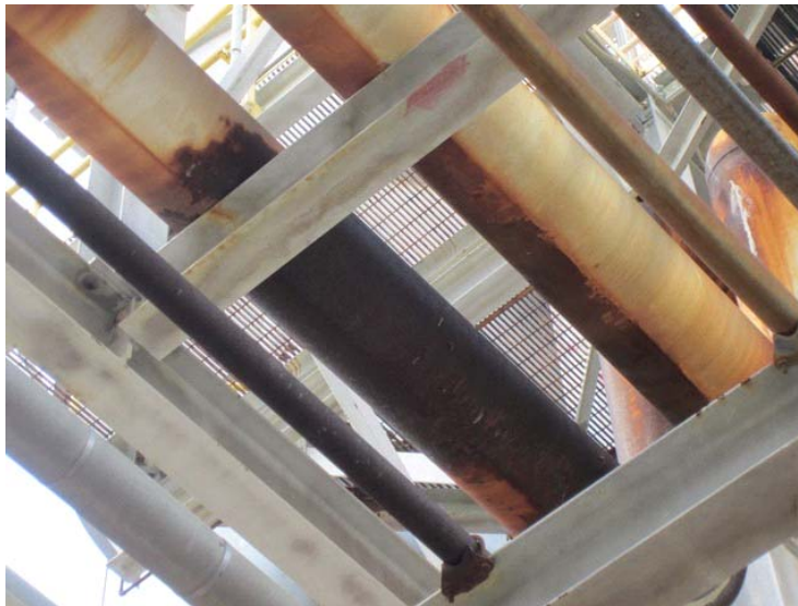
Corrosion on piping
