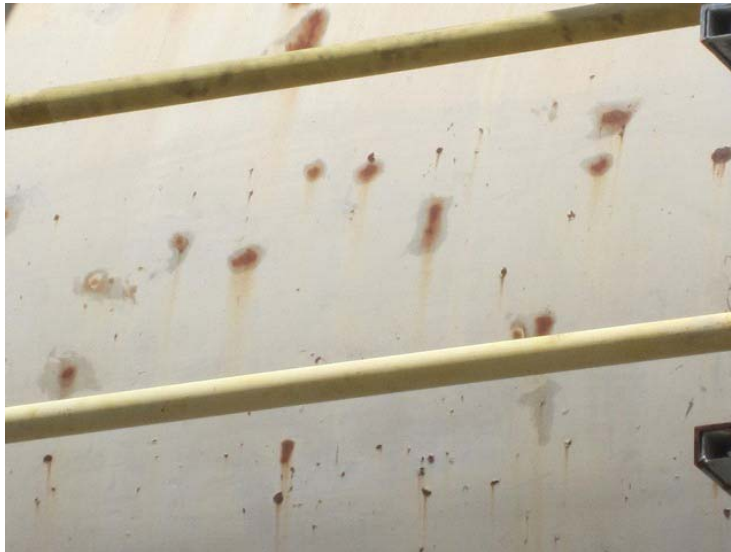
View of corrosion
