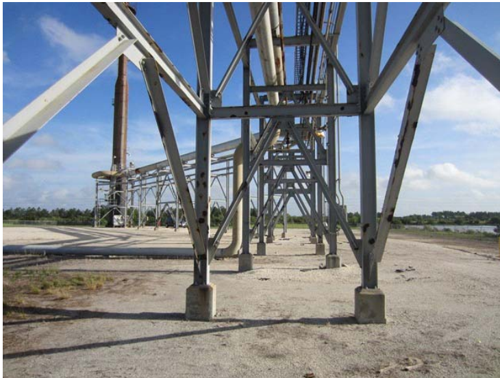
General view of piperack
