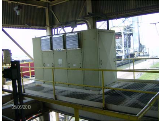
500kVA Transformer at T2
