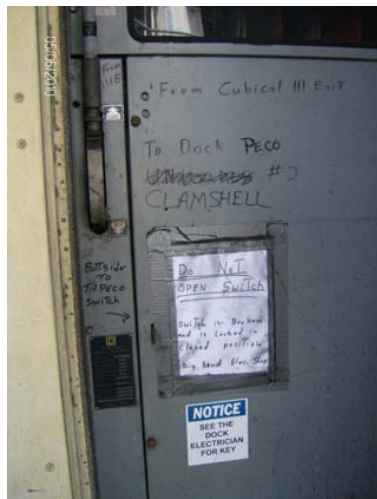
PECO Disconnect in T2 (not working)
