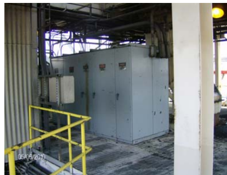
5kV Switchgear at T2 mid-level
