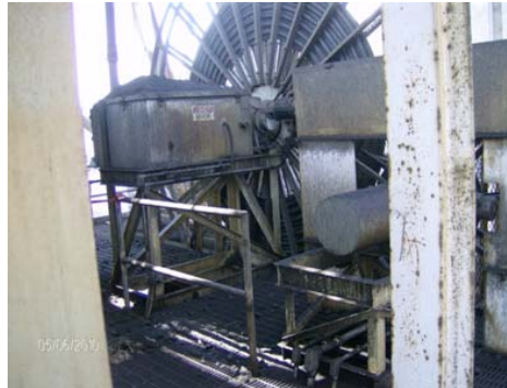
North Stacker/Reclaimer Cable Reel
