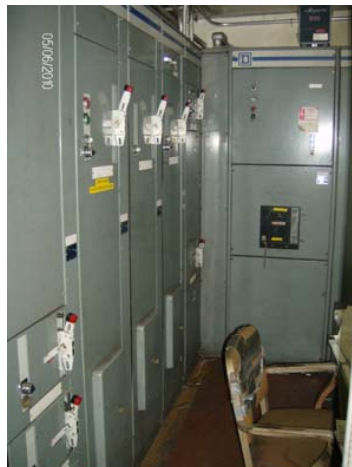
Elect Room in North Stacker/Reclaimer
