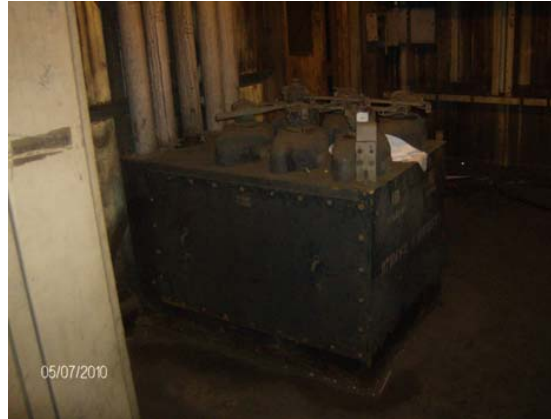
Manual Xfr Sw for L Conveyors
