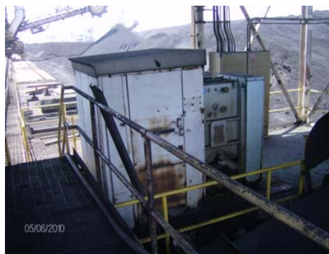
112.5kVA Transformer at T3
