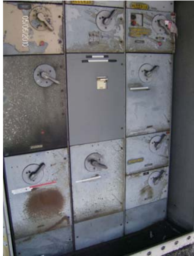
480V MCC at T2
