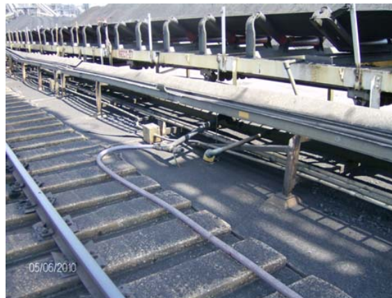
Conduits on north of P conveyor
