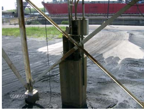
Ductbank at T4 with broken conduits
