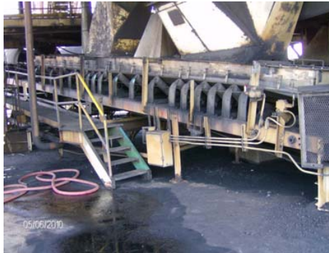
W1 Conveyor (tail end)
