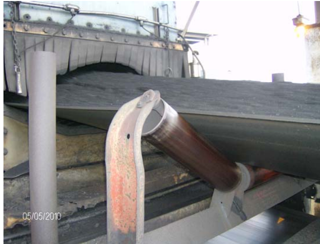
Idler Roller on Shaft
