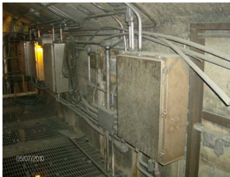
K Feeder Control Cabinets and starters
