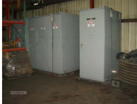
New 5kV Switchgear for coal yard
