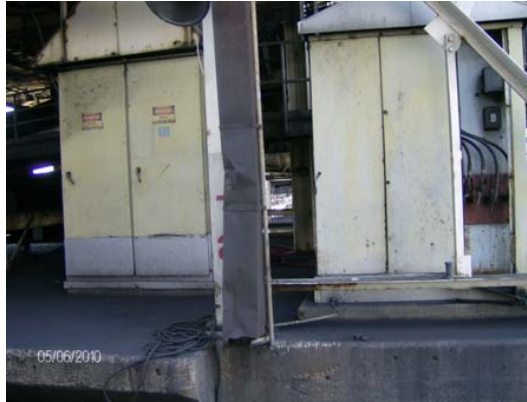
5kV Switchgear at base of T2 (gear on right is dead)
