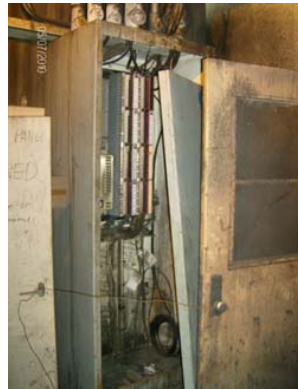
PLC Cabinet for L Conveyors
