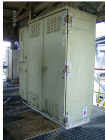
5kV Switchgear at T2
