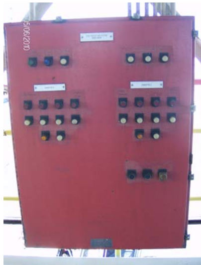
Fire Suppression Cabinet at T2
