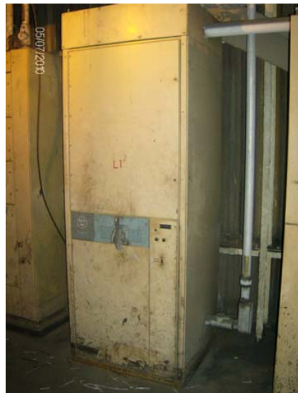
L1 Conveyor Motor Starter
