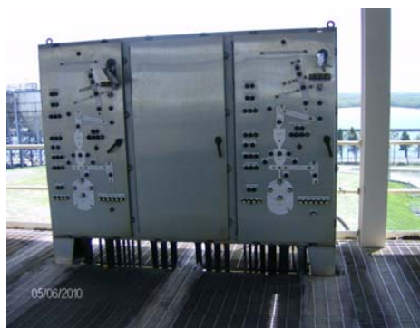
Sampling System Controls
