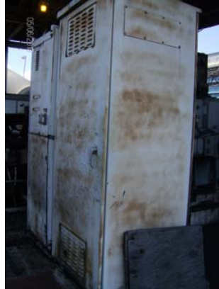
5kV Switchgear at T3
