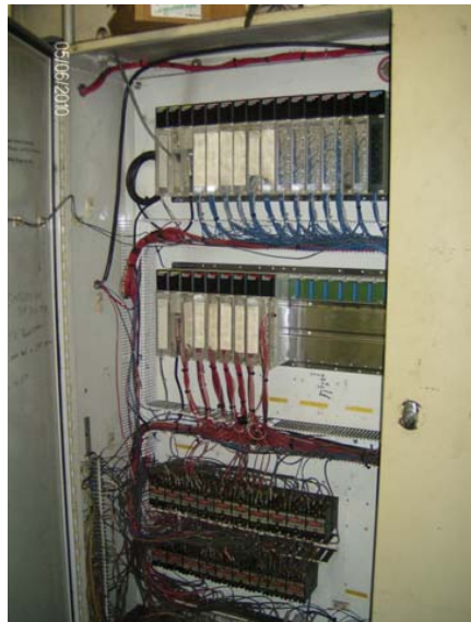
North Stacker Reclaimer Quantum™ PLC
