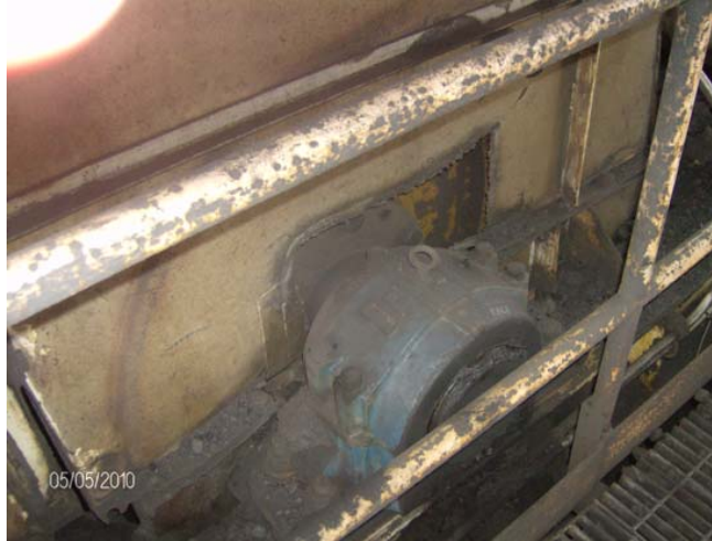
Penetration at Head Chute
