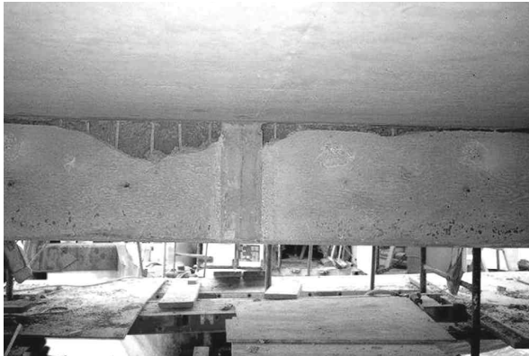
Effects of not filling the cavity.
