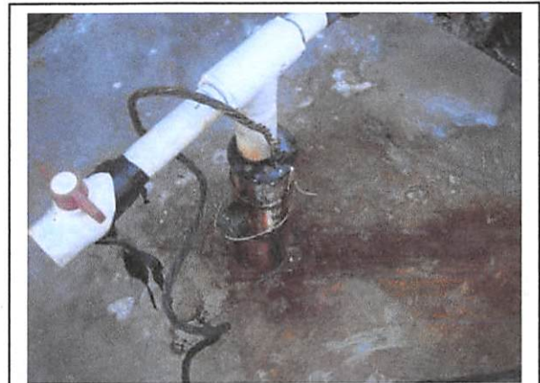
Water leaking around well head.
