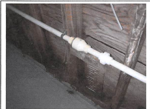
Deterioration of the wood along lower wall of the plant.
