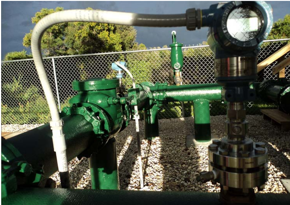
PRESSURE SENSOR ON JBW INFLUENT LINE.
