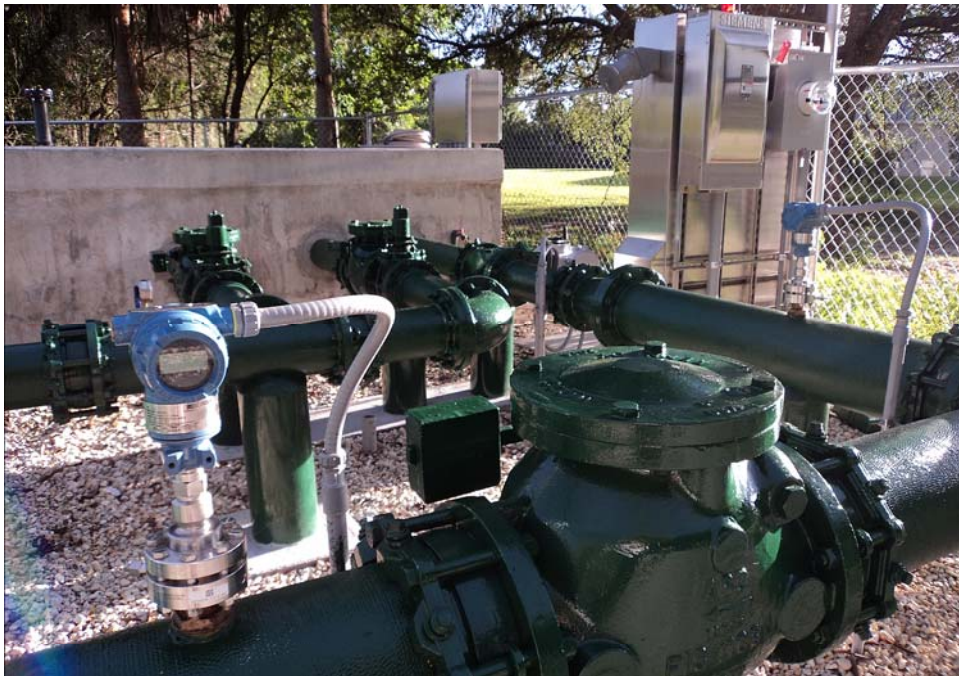
FOREST UTILITY SYSTEM PRESSURE SENSOR
