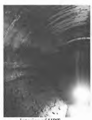
Interior of HPT
