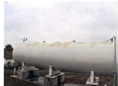
Rust on pressure tank
