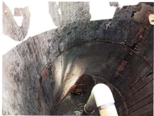
2 Indication of possible infiltration
