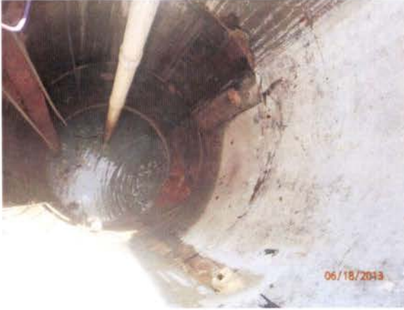
1 Leakage at lift station seam
