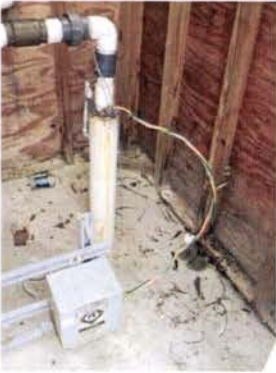
Well AAH9008 wiring and well seal.
