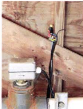
Pump room wiring
