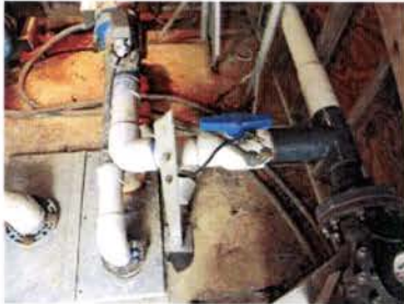
Pump room wiring
