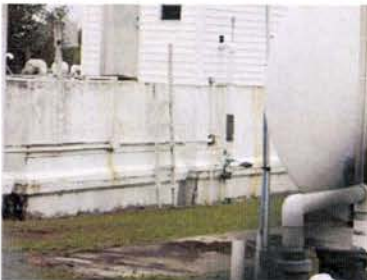
Ladder that needs to be replaced
