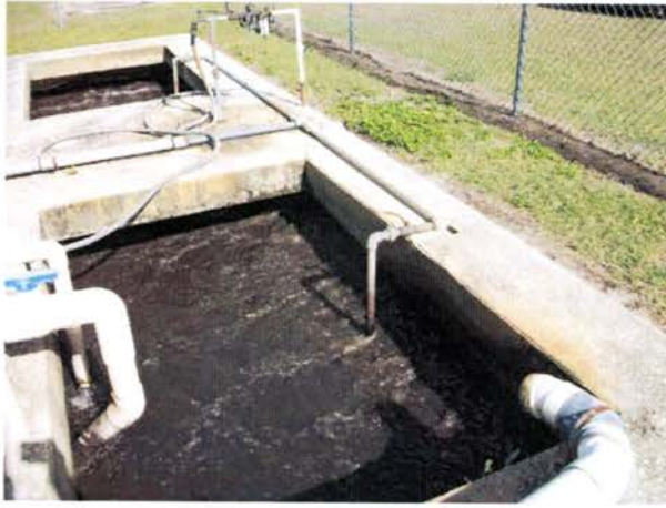
1 Uneven mixing in aeration tank
