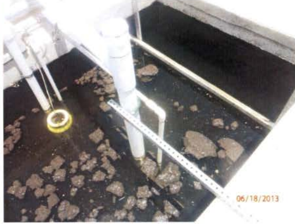
2 Pop ups in clarifier
