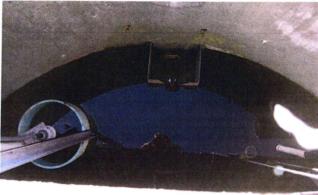
Final Effluent in CCC, Ultrasonic Flow Sensor and V-Notch Weir
