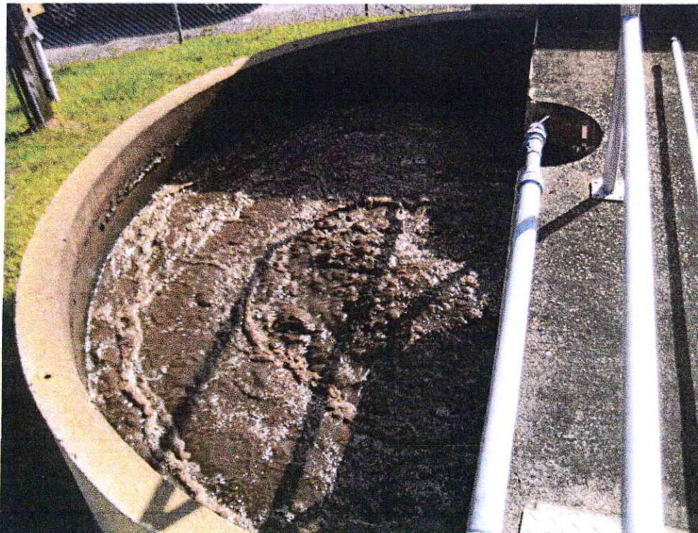
One of Five Aeration Basins
