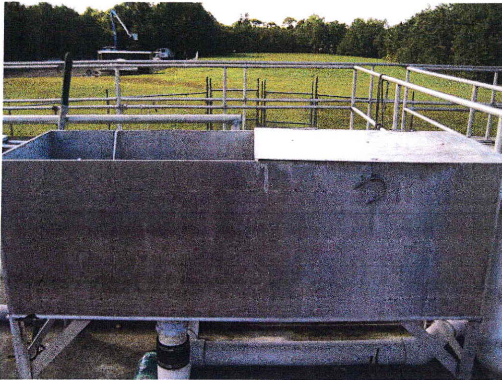
Splitter Box with Bar Screen/ Background: Effluent Disposal System
