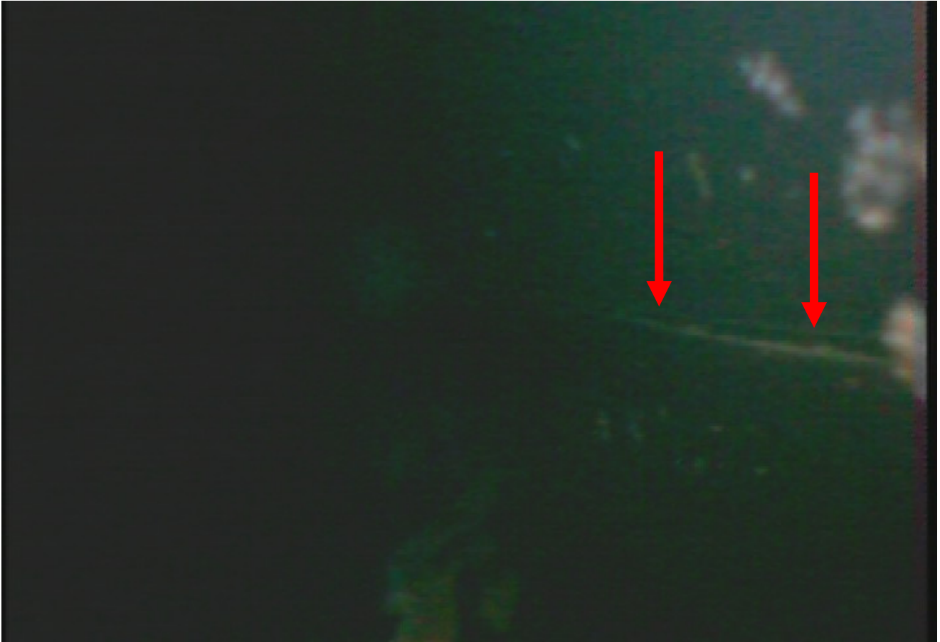
Figure 3: Boroscope photo of linear indication on 2A1 R74-T53 as taken during short notice outage in February 2015 (Interim Root Cause Report).
