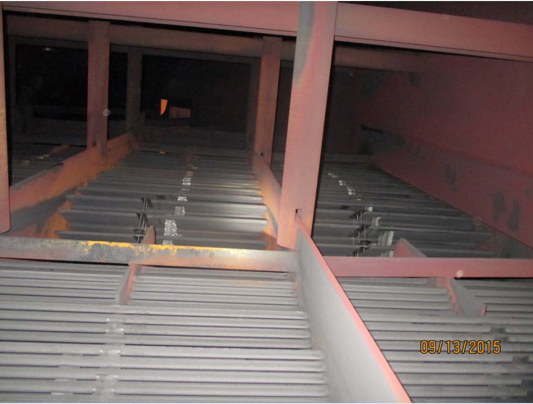
Figure 7: Illustration of the steam space of the Unit 2 Condenser, tube bundles, and tube baffle plates.
