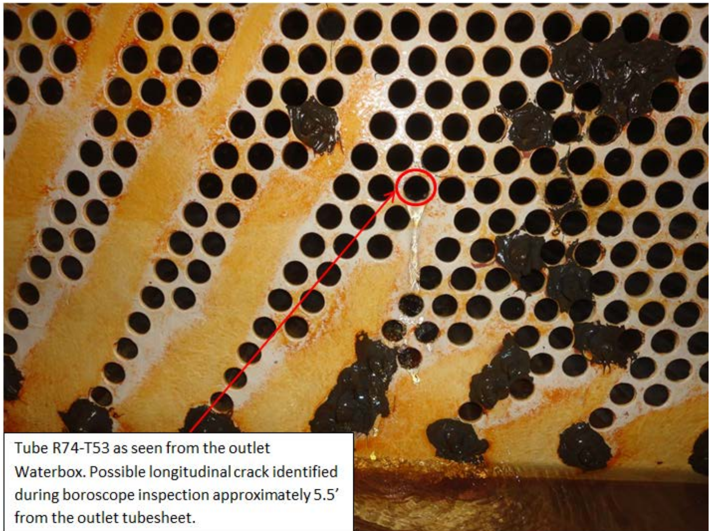
Figure 2: 2A1 lower bundle tube R74-T53 leaking during short notice outage hydrostatic test in February 2015 (Interim Root Cause Report).
