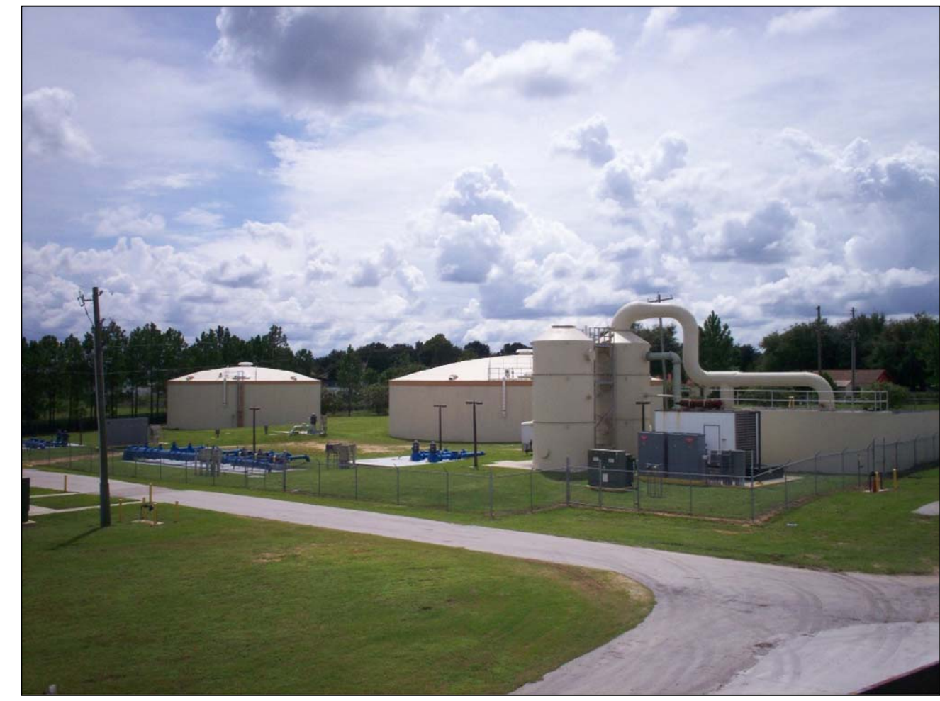
7 LAKE GROVES WATER TREATMENT PLANT
