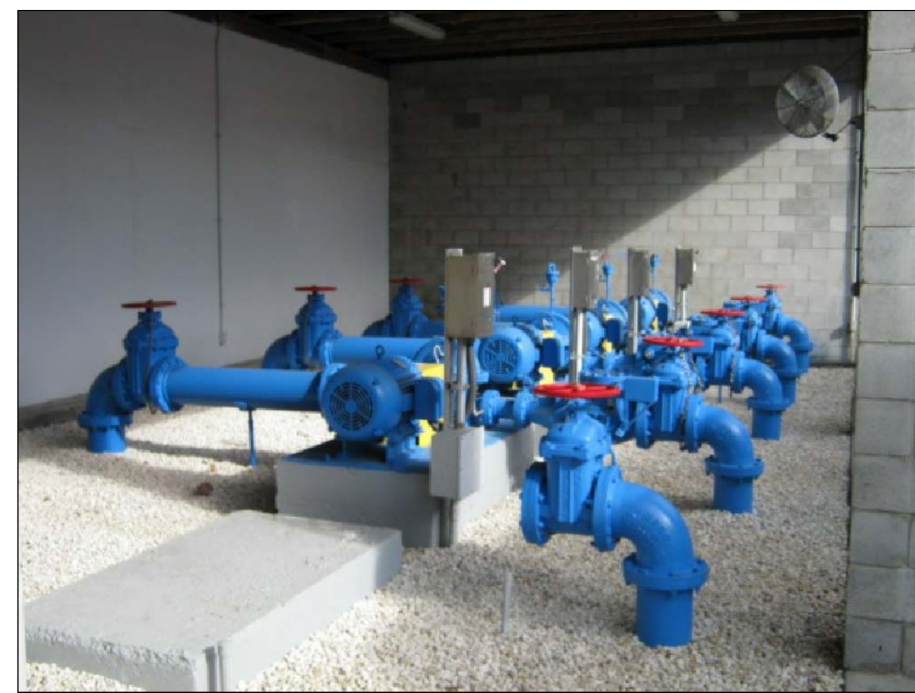
7 THE VISTAS - HIGH SERVICE PUMPS
