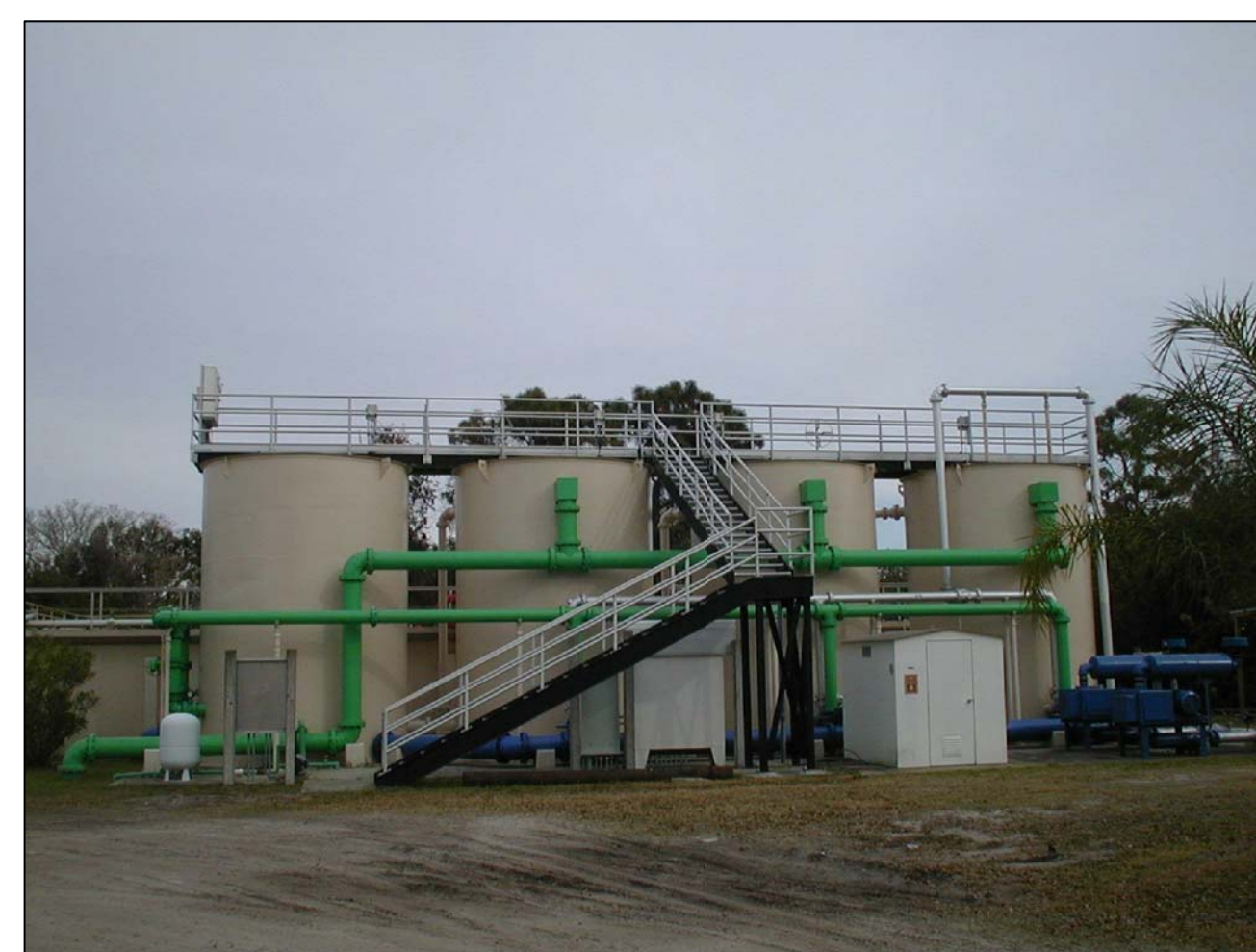
11 MID-COUNTY SERVICES DENITRIFICATION TANKS
