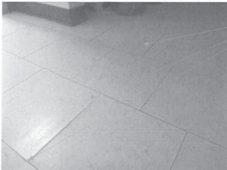
Photo 10. Damaged flooring outside of storage room
