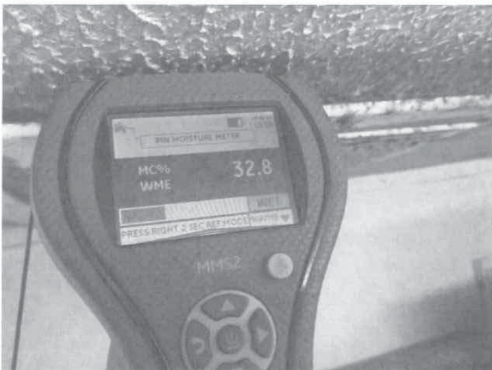
Photo 9. Elevated moisture level in ceiling material around lab AC vent seen in photo 8
