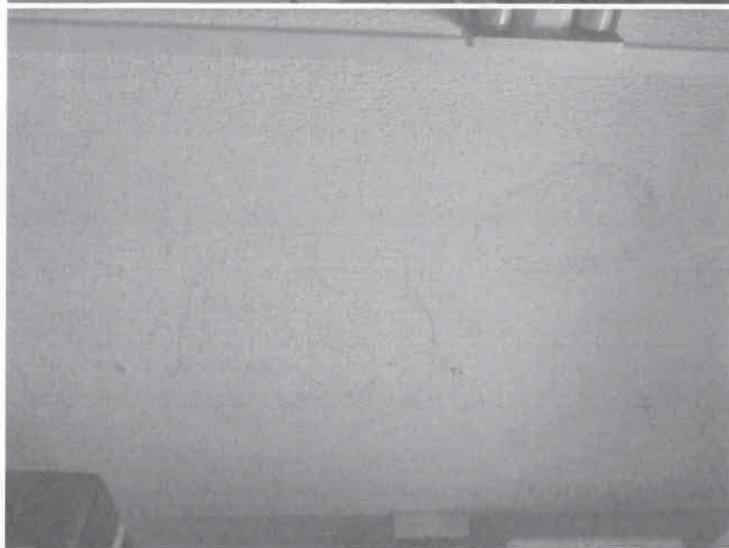
Photo 23. Water stains in ceiling of Kaitlin's office
