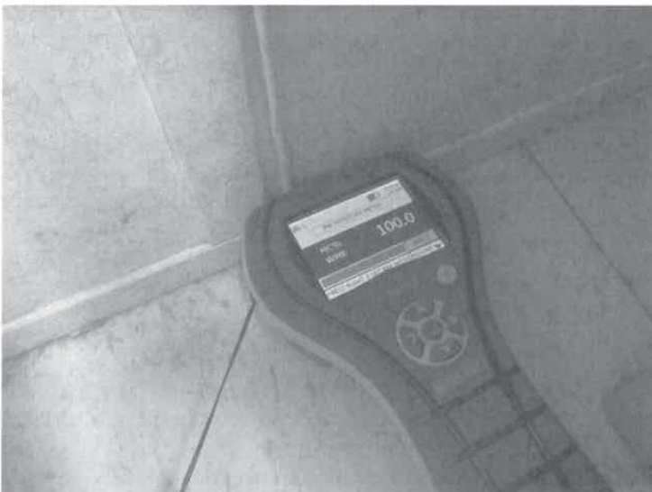
Photo 15. Elevated moisture level in base of wall under window on east wall just outside of women's restroom
