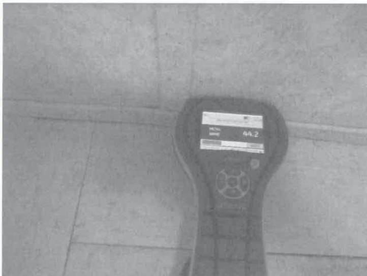
Photo 18. Elevated moisture level in the base of the south wall of the women's restroom
