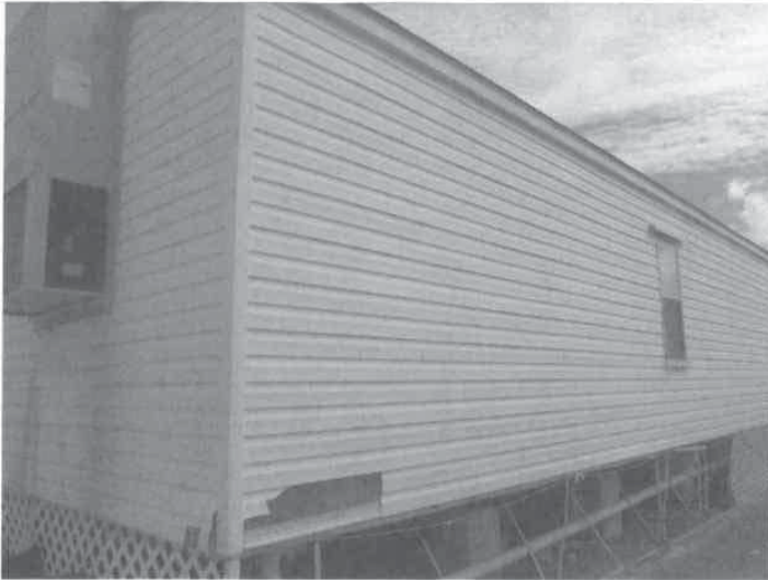
Photo 25. Damage to siding on west side of building
