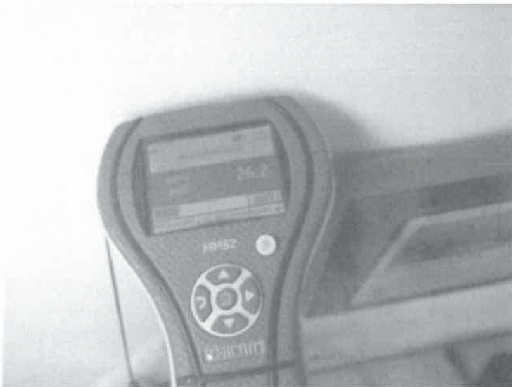
Photo 14. Elevated moisture level in south wall of conference room a few feet down from vent
