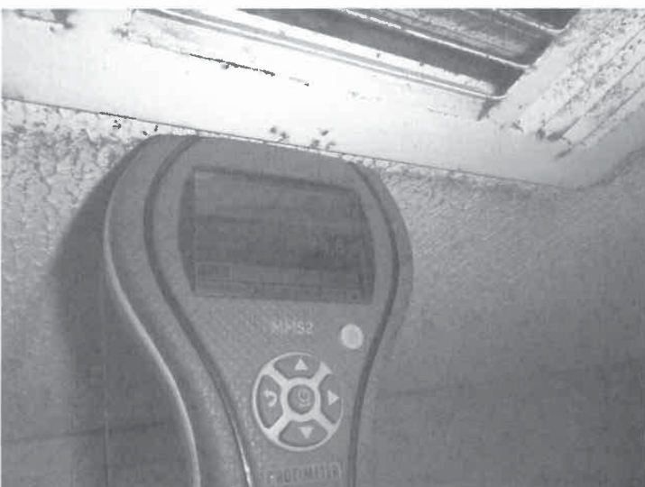
Photo 6. Elevated moisture level of 24.8% in ceiling material next to AC vent in men's restroom
