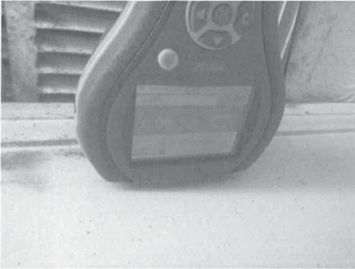
Photo 13. Elevated moisture level in south wall of conference room just under vent
