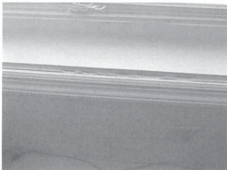
Photo 24. Damage to window frame in Kaitlin's office
