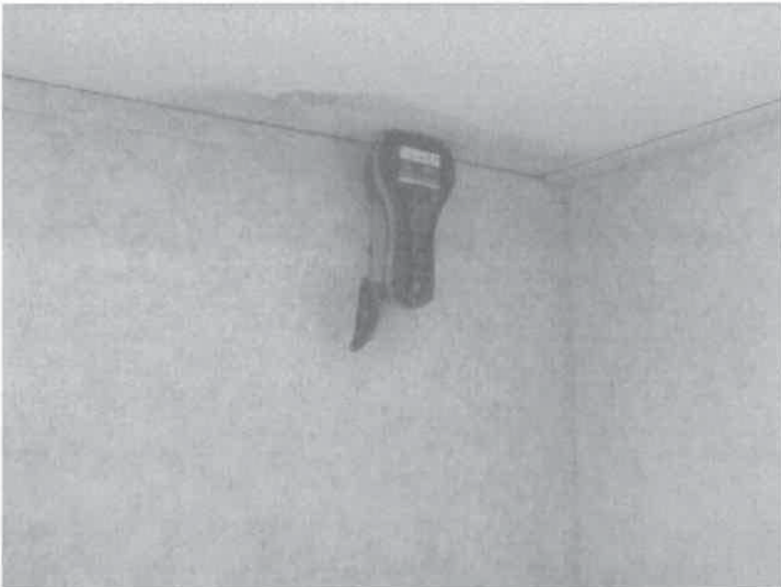
Photo 20. Water stain and elevated moisture level in south-west corner of ceiling in Judy's office
