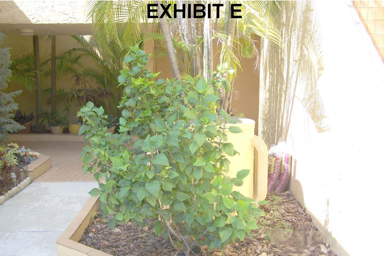
FPL's liquid-filled transformer installed southeast of Building 9310 in South Winds Condominium
