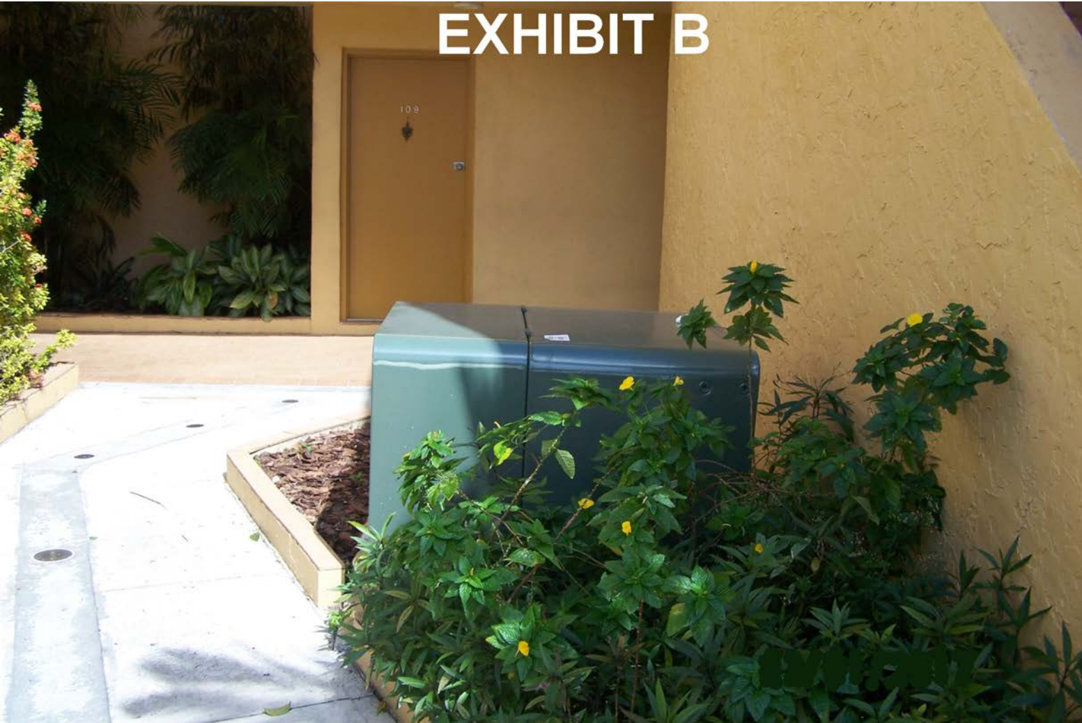
FPL's liquid-filled transformer installed west of Building 9300 in South Winds Condominium
