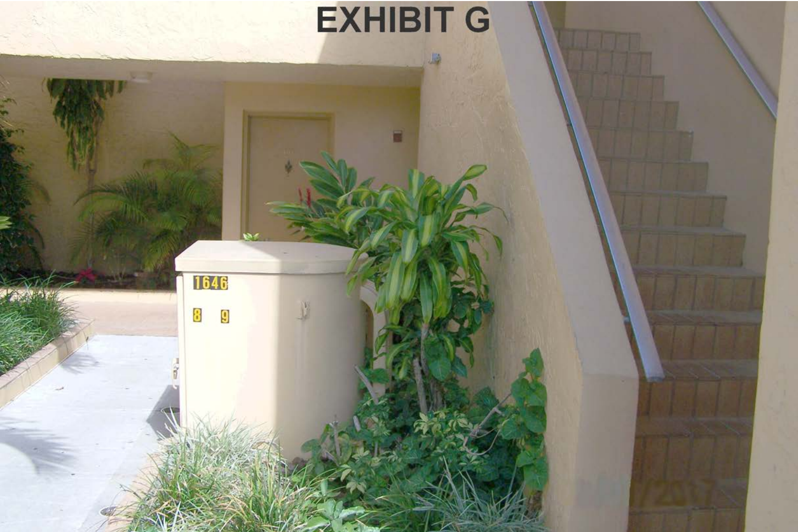
FPL's liquid-filled transformer installed west of Building 9340 in South Winds Condominium
