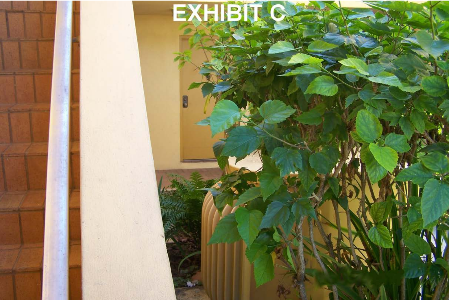
FPL's liquid-filled transformer installed east of Building 9300 in South Winds Condominium
