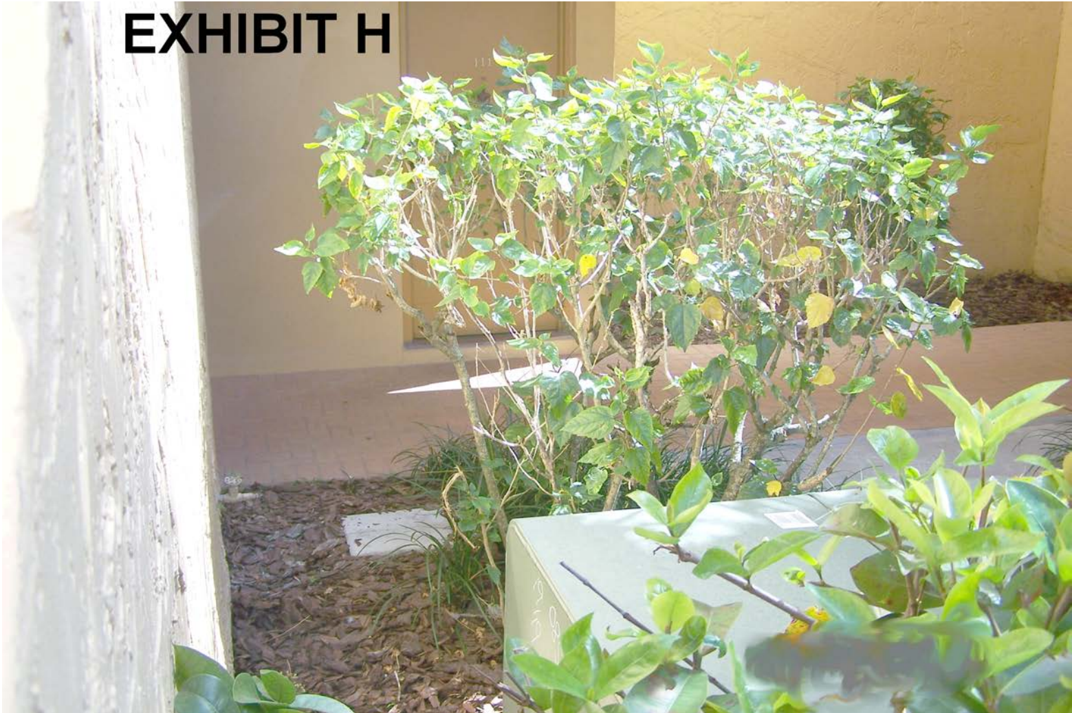
FPL's liquid-filled transformer installed northeast of Building 9311 in South Winds Condominium
