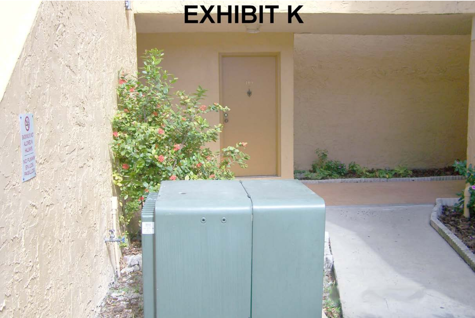
FPL's liquid-filled transformer installed west of Building 9301 in South Winds Condominium
