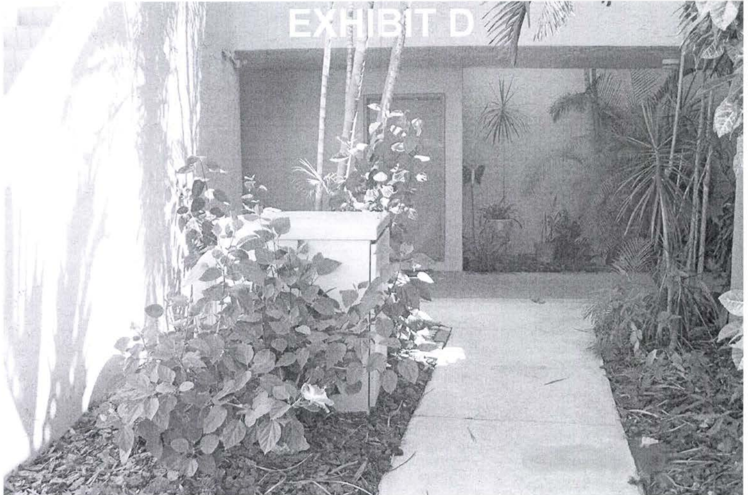
FPL's liquid-filled transformer installed northeast of Building 9310 in South Winds Condominium
