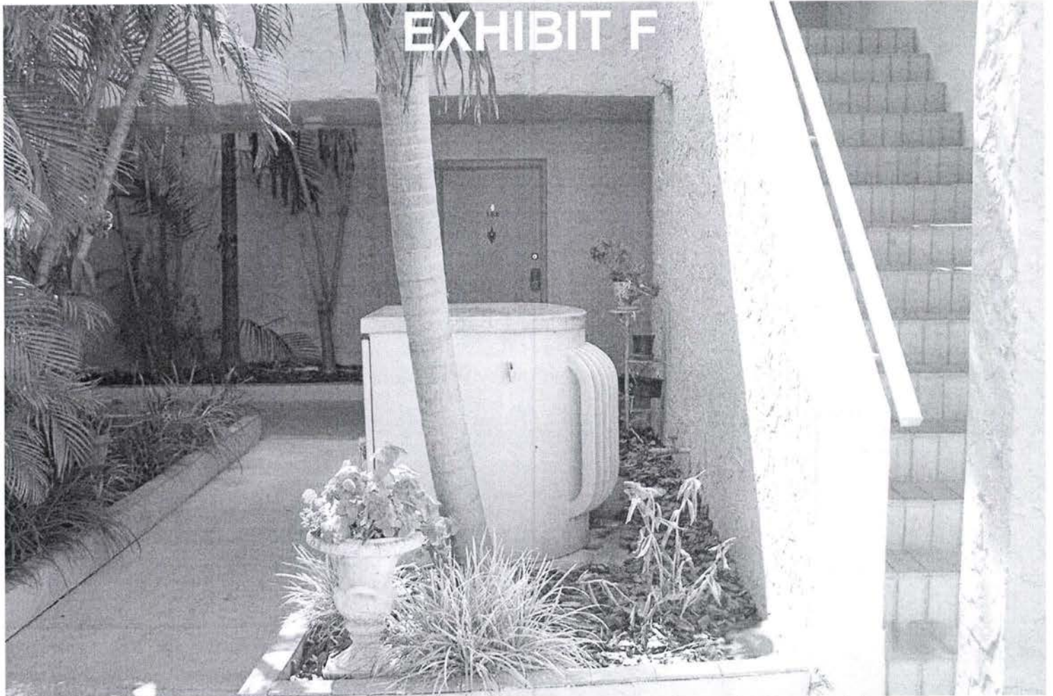
FPL's liquid-filled transformer installed east of Building 9320 in South Winds Condominium
