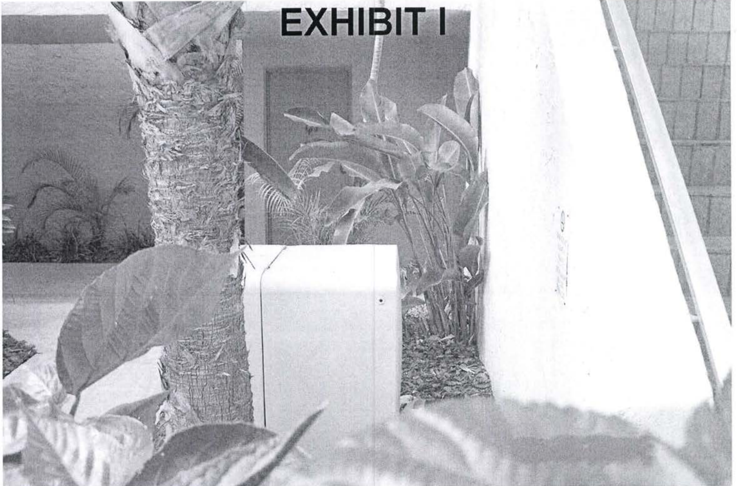
FPL's liquid-filled transformer installed southeast of Building 9311 in South Winds Condominium
