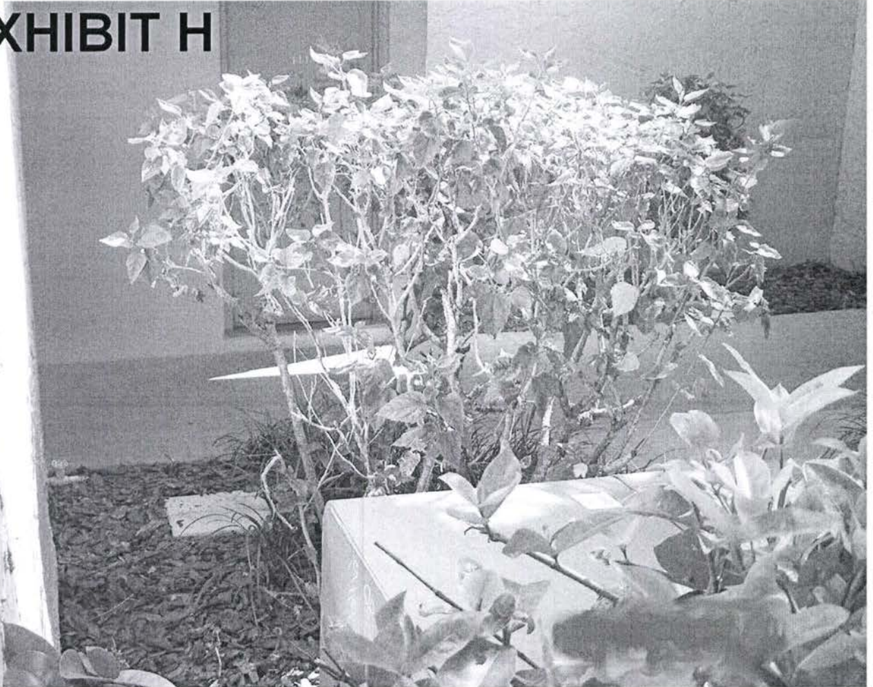
FPL's liquid-filled transformer installed northeast of Building 9311 in South Winds Condominium
