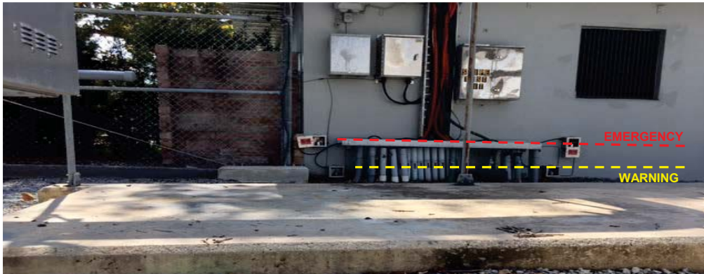
Alarm log for South Daytona Substation
