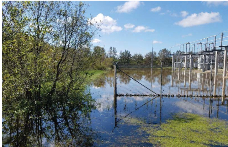
Corkscrew Substation Rain Event Flooding
