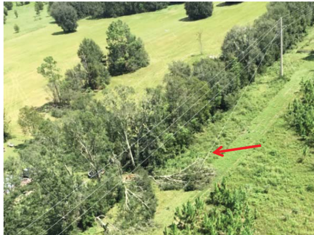
Structure 112R1 - Wire down due to vegetation
