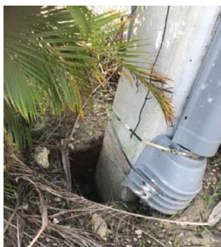
Base of leaning concrete pole
