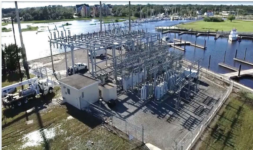
St. Augustine Substation
