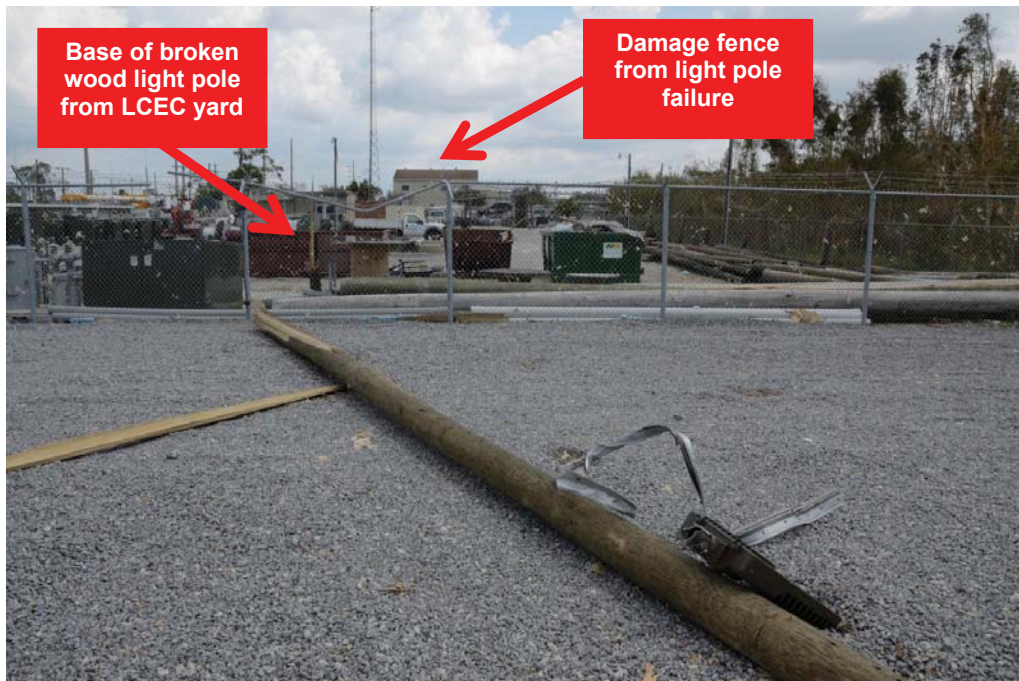
Belle Meade Substation (Looking East) adjacent to LCEC yard (Lee County Electric Coop)
