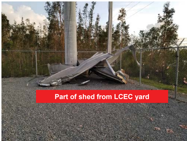
Belle Meade Substation (Looking West)
