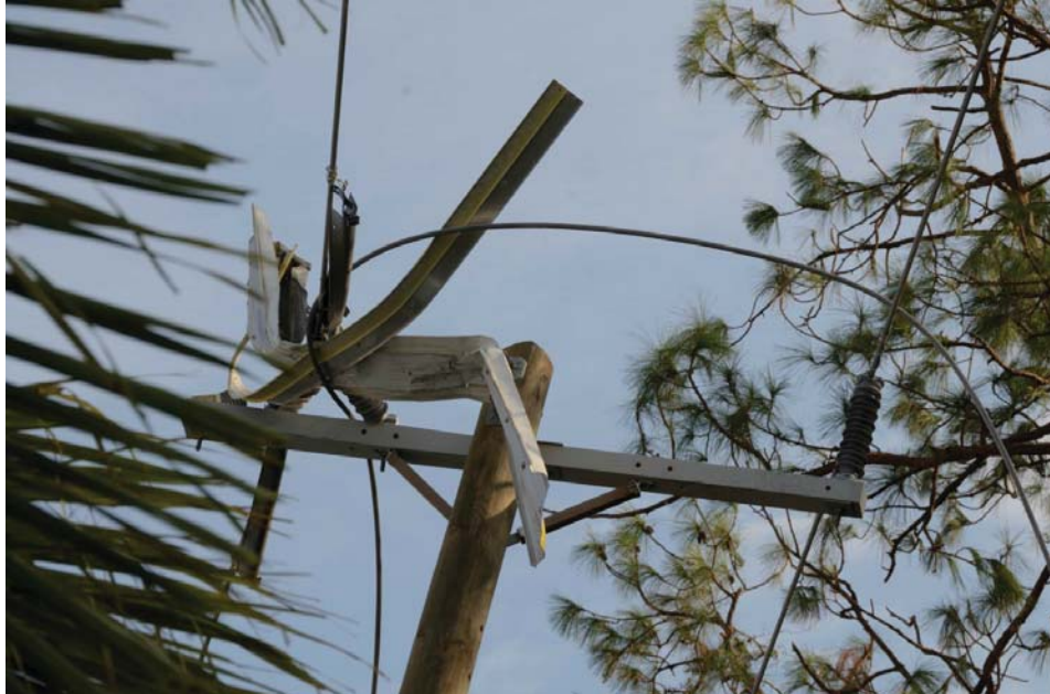
Debris wrapped around pole in line.
