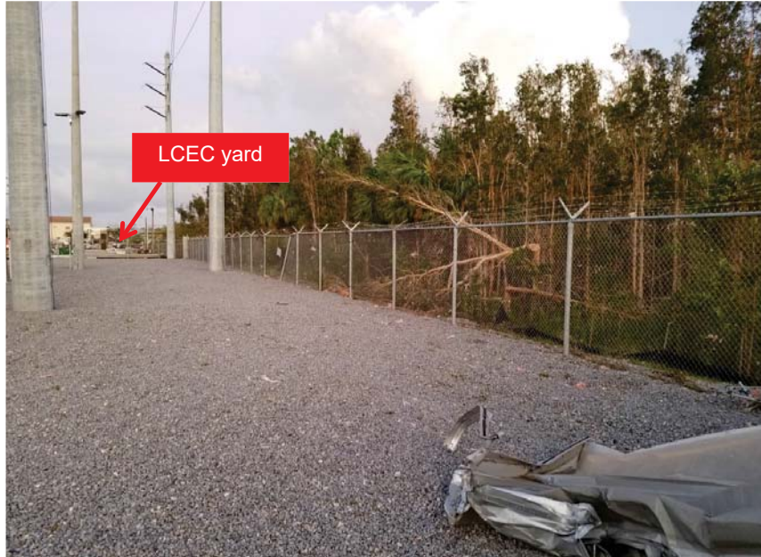
Belle Meade Substation (Looking East)
