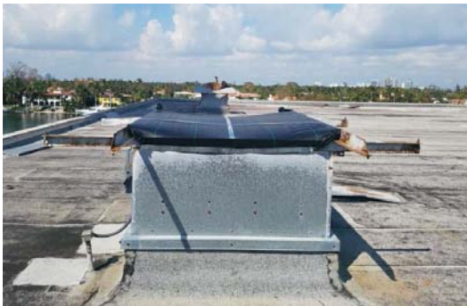
Indian Creek Substation – Roof Exhaust Fan
