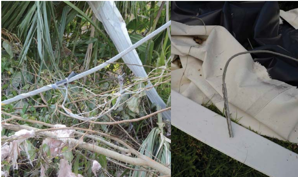
Insulator tie and failed splice. Below: ALS out of support and on ground
