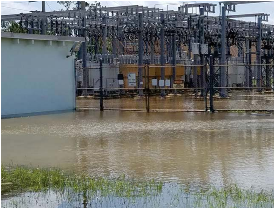
Pine Ridge Substation rain event flooding
