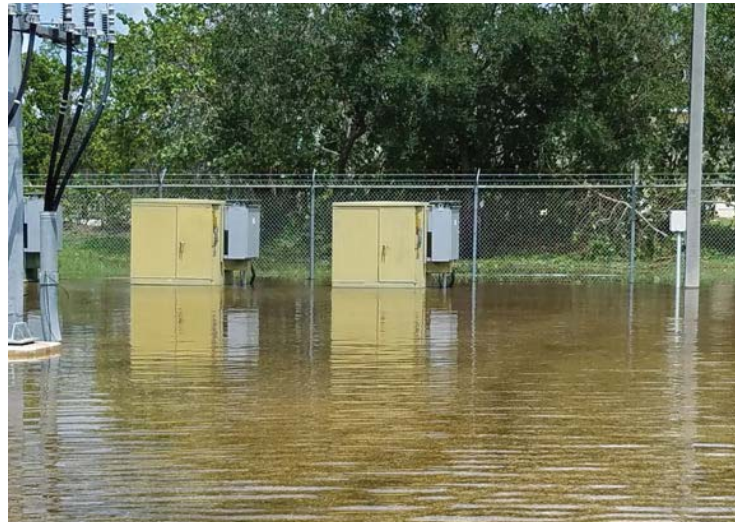
Pine Ridge Substation Flooding
