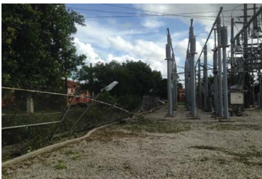
Crystal River Substation – Fence
