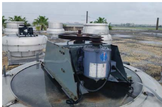
Watkins Substation – Roof Exhaust Fan
