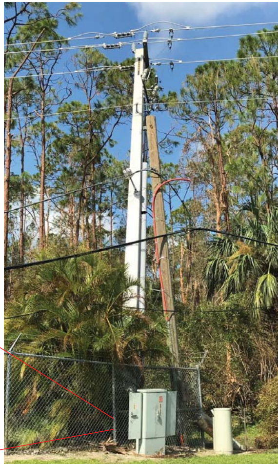
Leaning concrete pole
