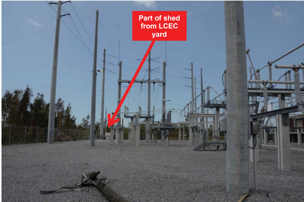
Belle Meade Substation (Looking West)
