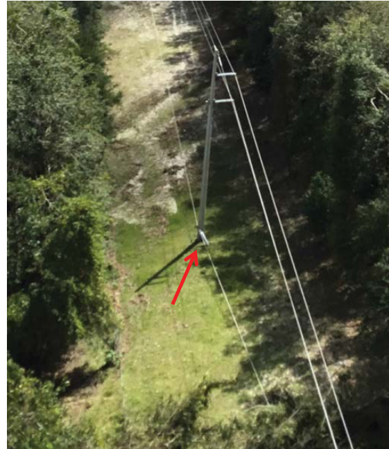
Structure 55R13A – Broken insulator
