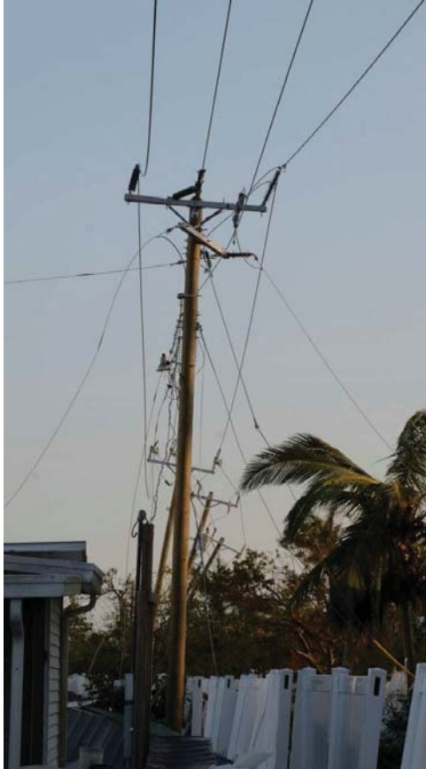
View of leaning poles
