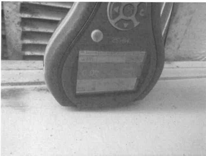
Photo 13. Elevated moisture level in south wall of conference room just under vent
