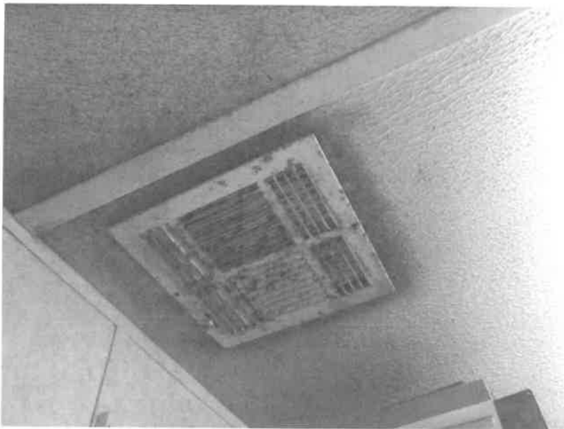
Photo 4. Air conditioning vent in Chris' office with fungal growth. Location of swab surface sample
