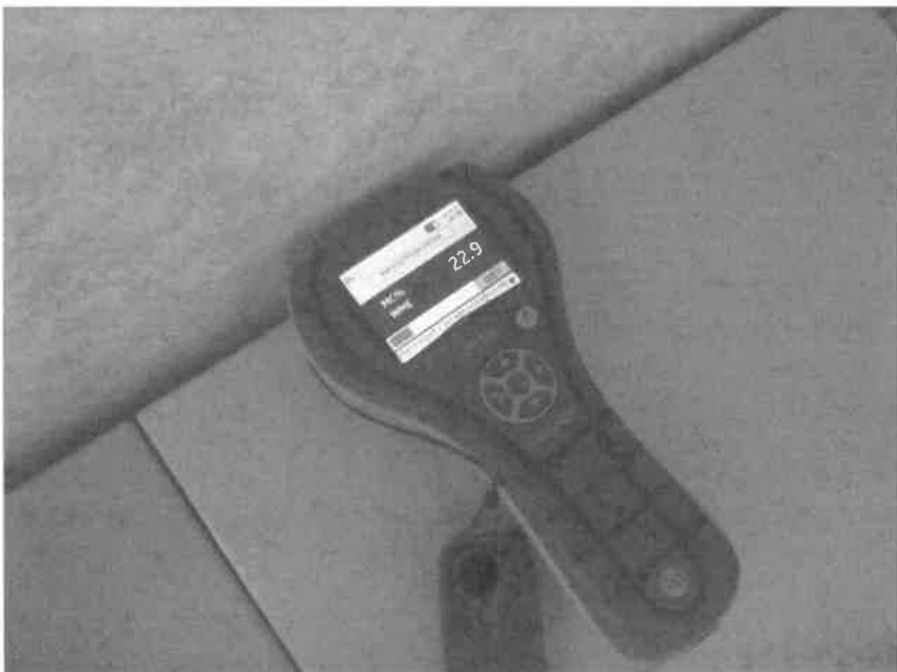
Photo 21. Elevated moisture level in wall under stained ceiling seen in Photo 20
