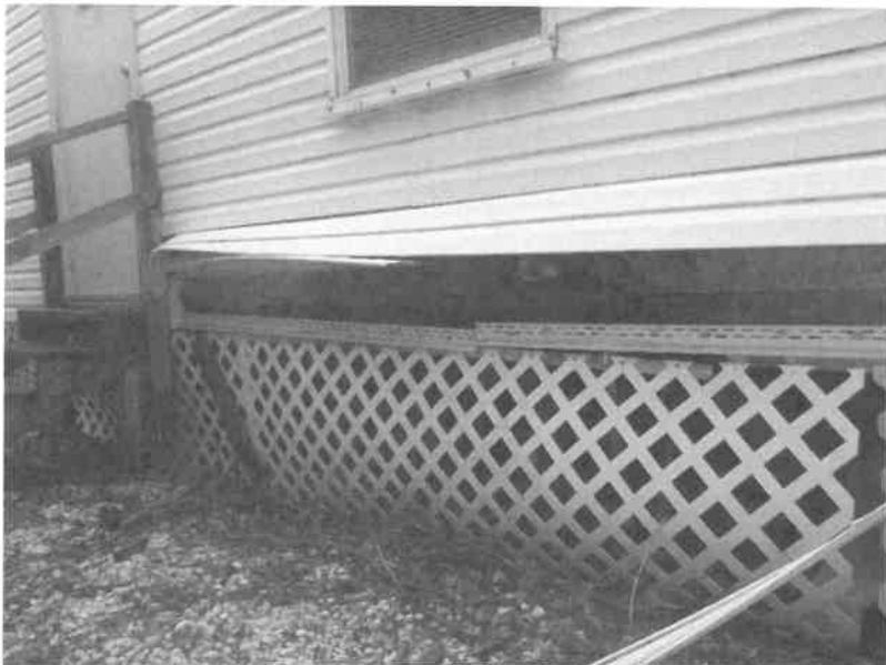
Photo 27. Damage to siding on east side of building
