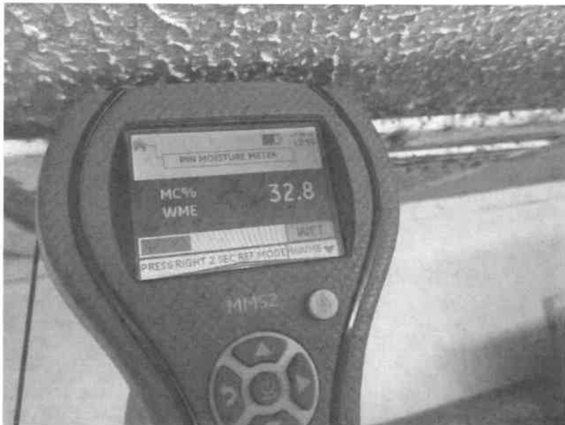
Photo 9. Elevated moisture level in ceiling material around lab AC vent seen in photo 8
