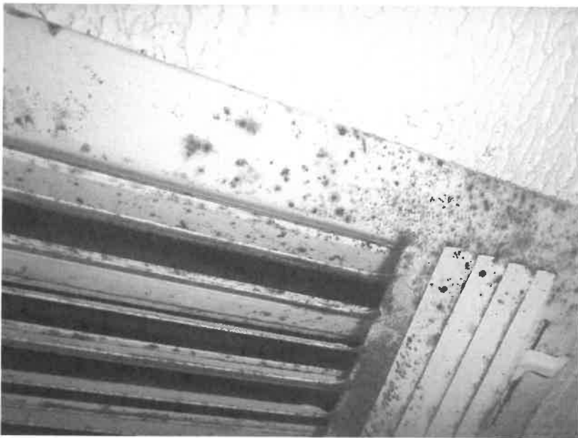
Photo 5. Close-up of fungal growth on AC vent in men's restroom
