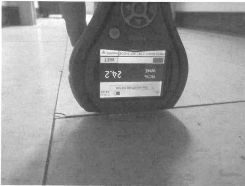
Photo 11. Elevated moisture level in floor outside storage room seen in Photo 10
