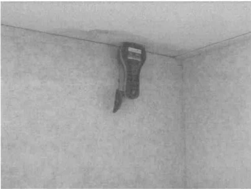
Photo 20. Water stain and elevated moisture level in south-west corner of ceiling in Judy's office
