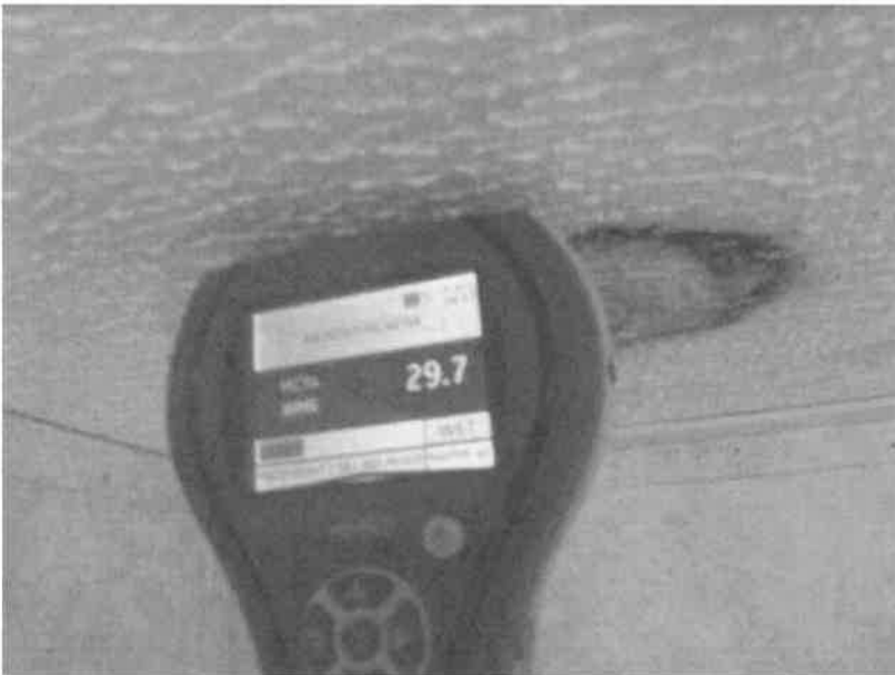
Photo 17. Elevated moisture levels around a water and possible fungal stained area in the ceiling of the women's restroom
