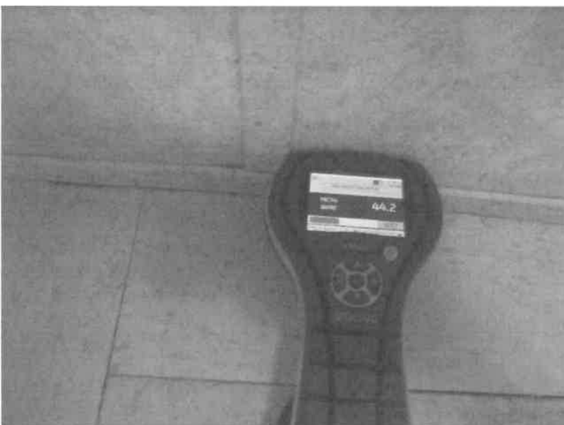
Photo 18. Elevated moisture level in the base of the south wall of the women's restroom
