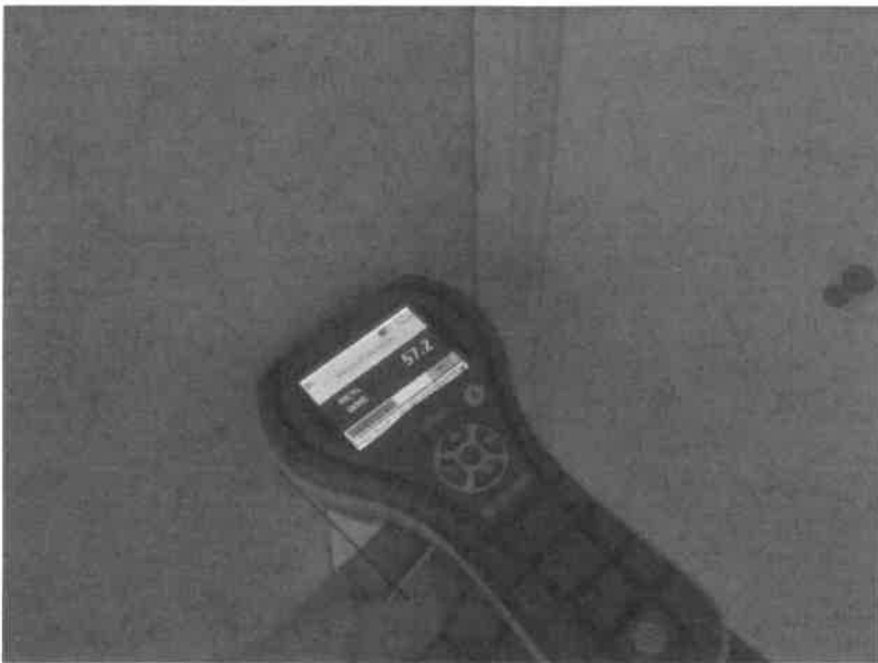
Photo 16. Elevated moisture level about a foot from the base of the wall under the window outside of the women's restroom
