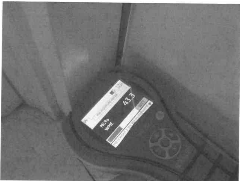
Photo 22. Elevated moisture level in left side of door frame to door outside of Kaitlin's office
