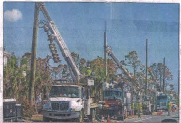
Workers install power poles in Mexico Beach in the immediate aftermath of October's Hurricane Michael, which devastated the eastern Panhandle. [LANNIS WATERS/PALM BEACH POST]
